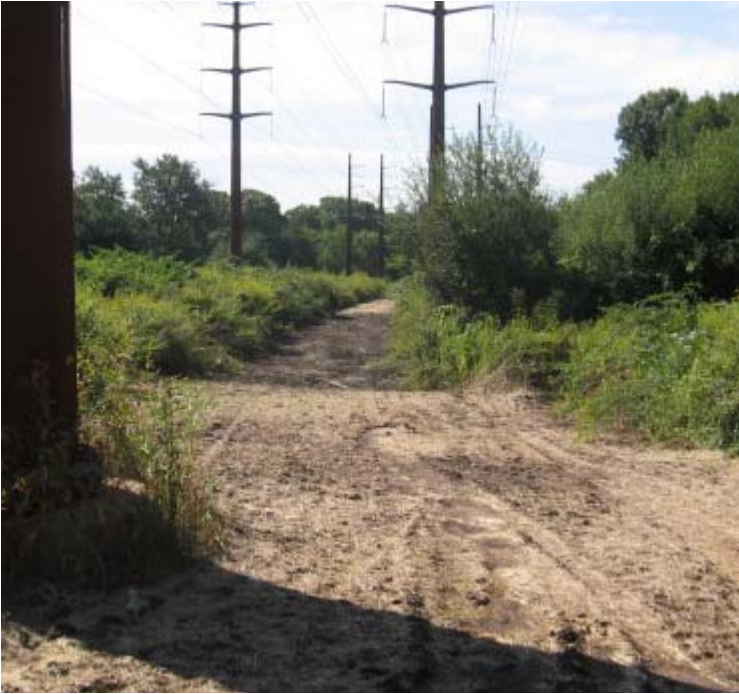
Sunset Dr (Orange): A view of the restoration efforts near the wetland area here. Exposed upland soils have been graded, mulched and seeded. Wetland soils have been graded.
