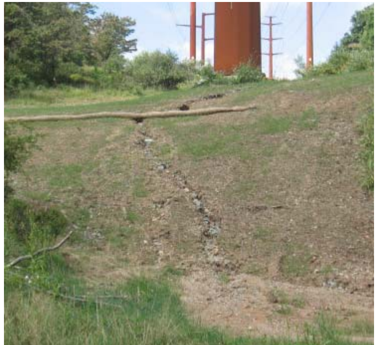
Dogburn Rd: Stormwater run-off continues to erode the disturbed area near structure #24077.
