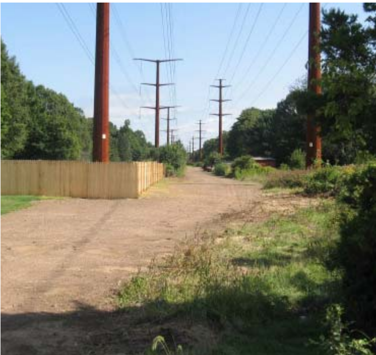
Treat Ln (Orange): A view of the restoration efforts in this area.
