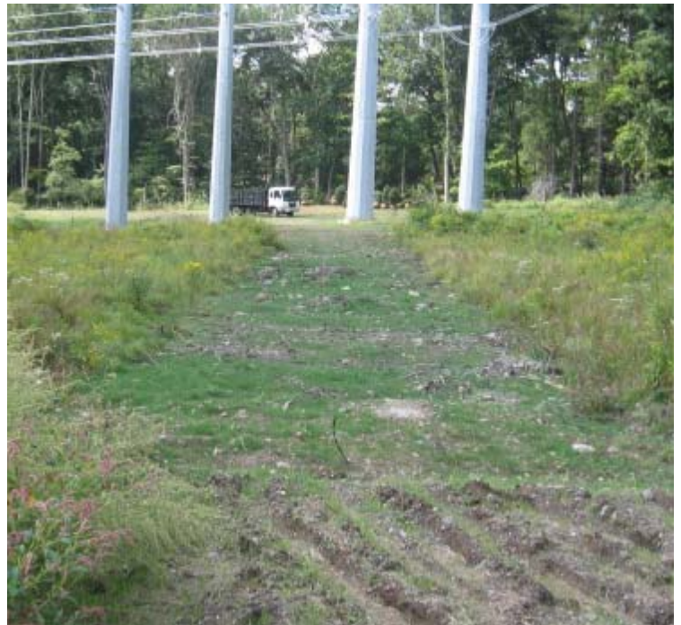
Rimmon Rd/B'nai Jacob: A view of the restored access road through the newly routed ROW. Vegetation growth continues here.
