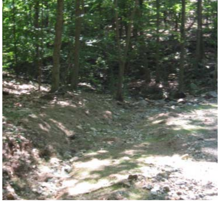
Cowpath Ln: The wetland crossing between structures #24129-24130, is permanent and appears stable at this time. Waterbars, a stone swale, and a stone check dam remain to help control run-off.
