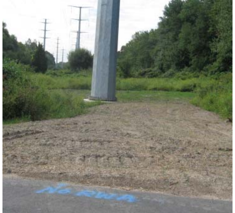
Manville Rd: The access road remains in the wetland here, as permitted. The stone access has been covered with hay mulch and seeded with loam.
