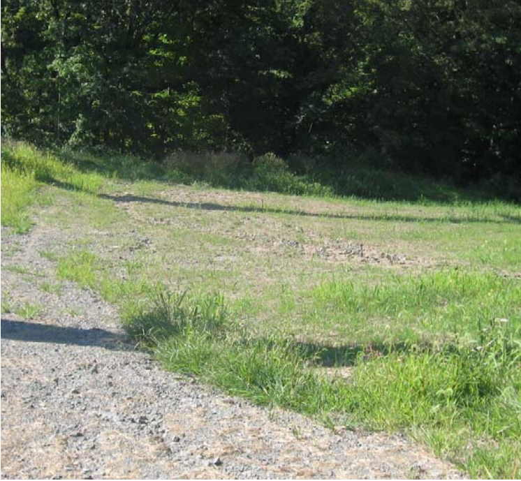
Wheelers Farm Rd (Milford): Some scouring has resumed along the slope near structure #3832. Gullies were also observed. Place check dams or divert flow until the slope is stable.
