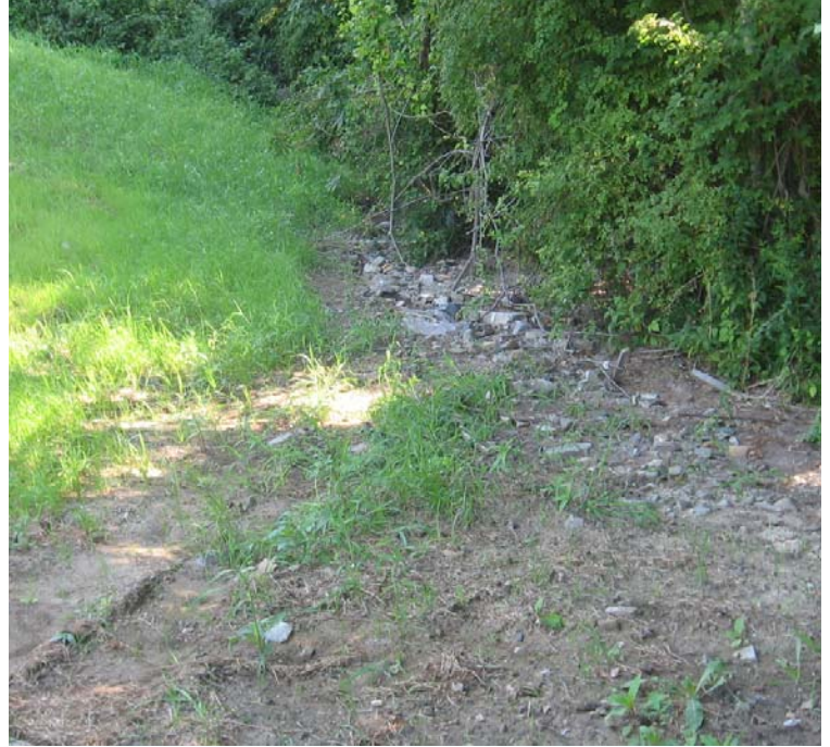
Lexington Way (Milford): Stormwater runoff flowing from a culvert beneath Hwy 15 is causing scouring/channelized flow along the perimeter of the ROW here.
