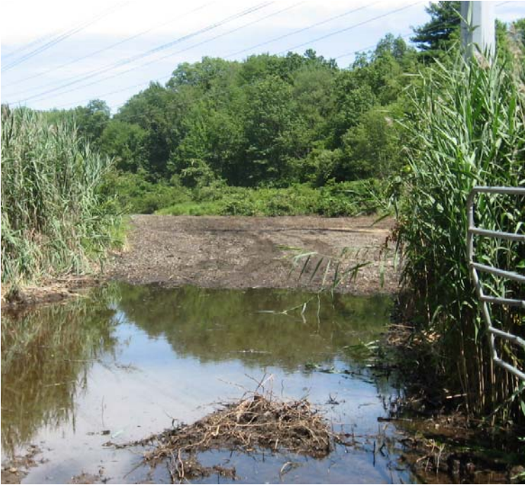
West River St (Milford): The access road has been restored to the original grade.
