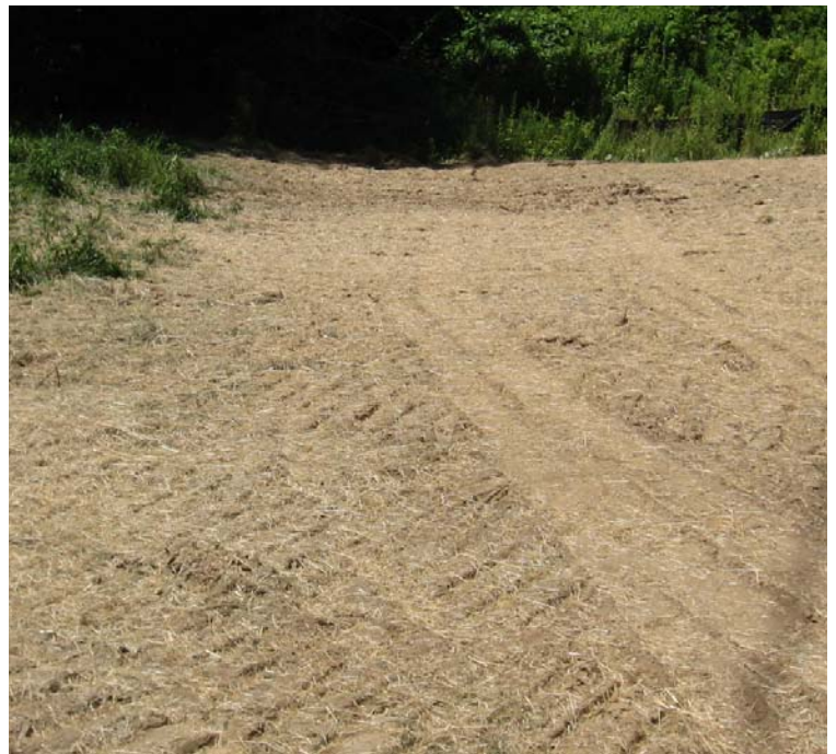
Wheelers Farm Rd: The crane pad near structure # 3832/24019 has been reclaimed and soils have been graded and mulched. The erosive gully in this area has been graded. Silt fence protection remains.
