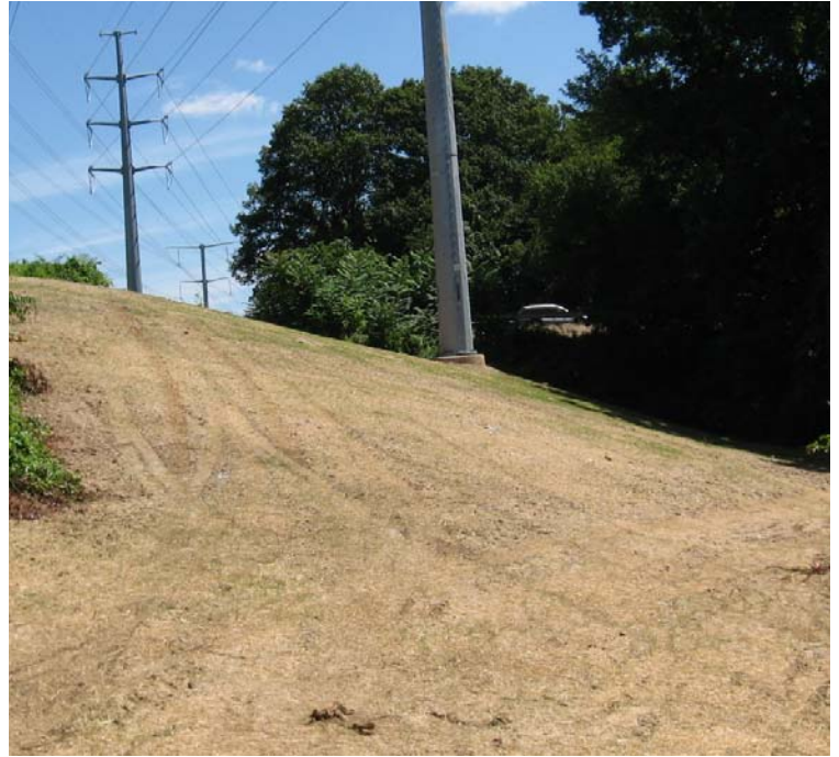
Lexington Way: Crane pads have been removed and exposed soils have been temporarily stabilized with mulch. Silt fence remains along the wetland boundary.
