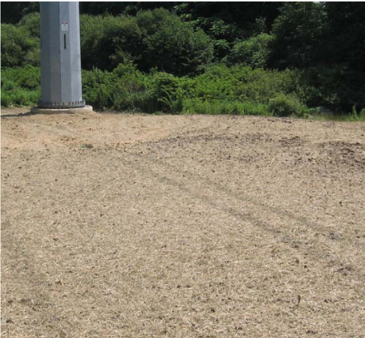
Oronoque Rd: Crane pads have been removed and exposed soils have been temporarily stabilized with mulch near structure # 24008.
