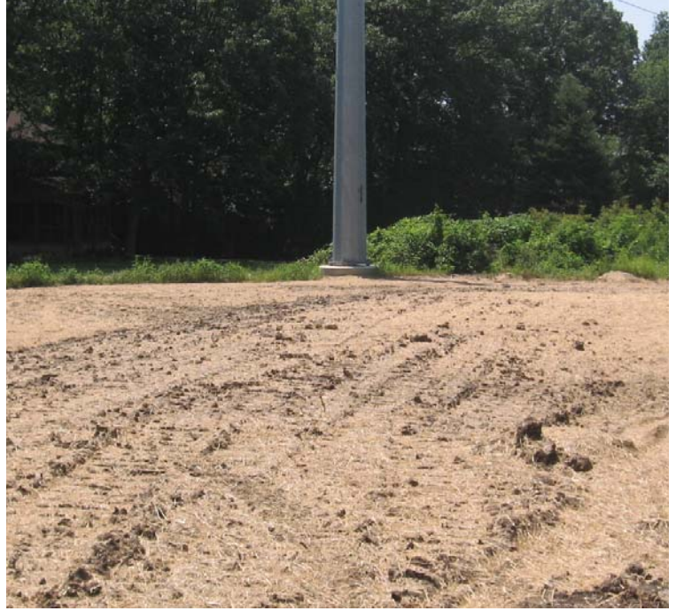
Oronoque Rd: Crane pads have been removed and exposed soils have been temporarily stabilized with mulch.
