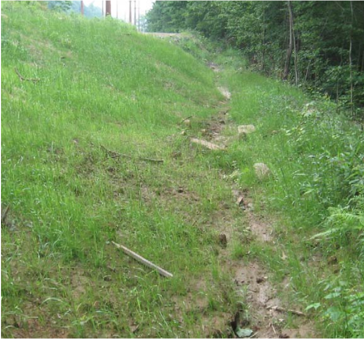
Gaylord Mtn Rd (Hamden): Vegetative growth has been noted in the swale located along the perimeter of the ROW.
