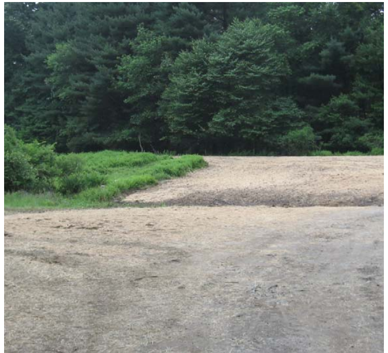
Clearview Ln: Wetland timber mats have been removed from the wetland near structure #3903/24090. Exposed upland soils have been temporarily stabilized with mulch.
