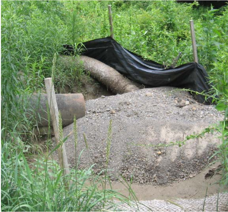
Glen Dam (Woodbridge): The sediment basin near structure #3950 is no longer functional.
