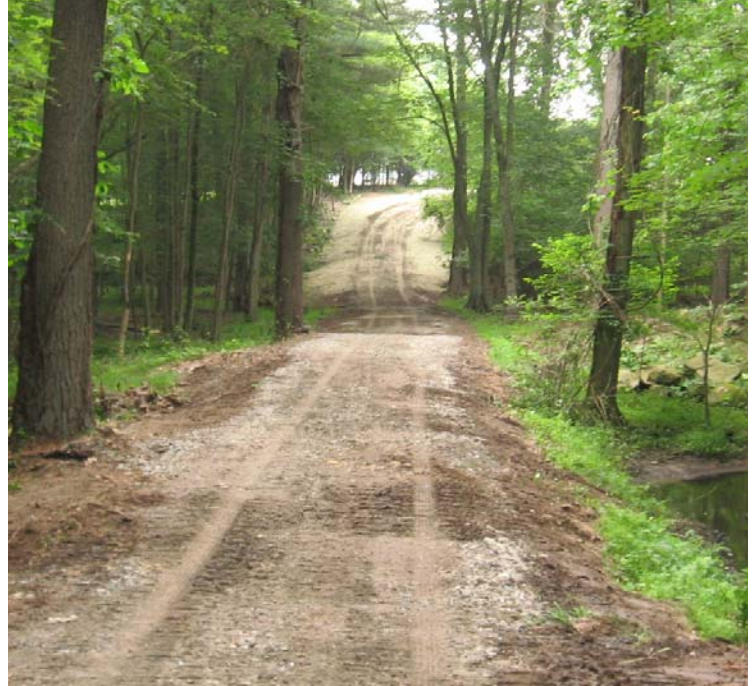
Clearview Ln: Wetland timber mats have been removed from the access road off Clearview Lane. The existing road has been graded.
