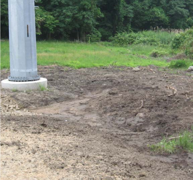
Clearview Ln: Wetland timber mats have been removed from the Wetland and soils have been graded near structure #24091.
