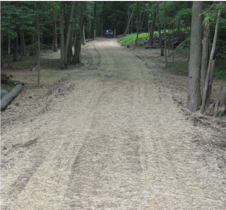
Clearview Ln: Upland access roads have been graded to the original grade and temporarily stabilized with mulch.
