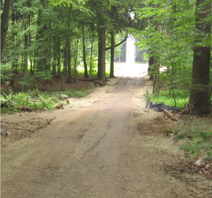
Clearview Ln: Wetland timber mats have been removed from the wetland crossing near structure#24090.
