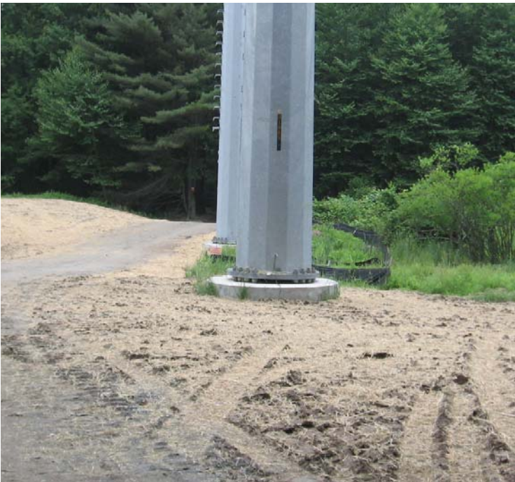
Clearview Ln (Woodbridge): A view of 115/345 kV restoration efforts. The access road has been returned to the original grade, and exposed soils have been temporarily stabilized with mulch.
