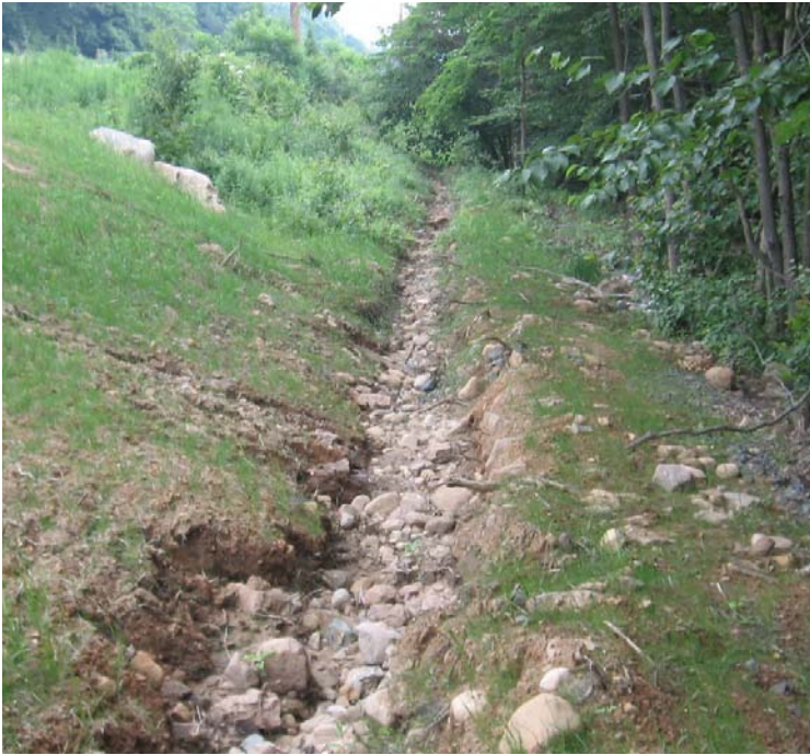
Gaylord Mtn Rd: View of the erosive gully located in the vegetative swale.
