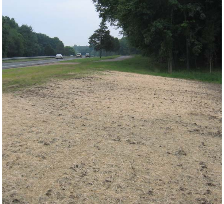
Clearview Ln: Exposed upland soils have been graded and temporarily stabilized with mulch.
