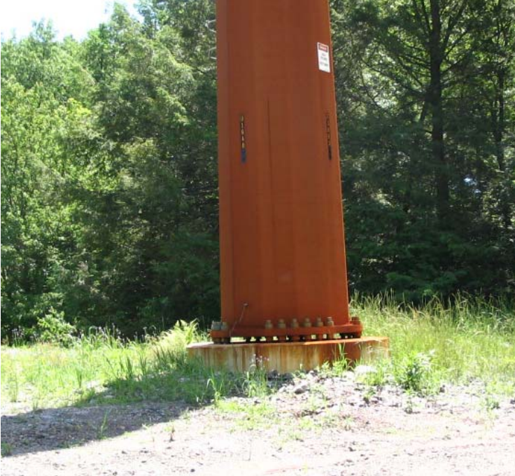
Lambert Rd (Orange): A view of 115kV restoration efforts near Structure #3863. Some vegetative growth has been observed.
