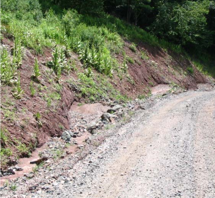
Old Ln (Hamden): Access road controls continue to help control stormwater runoff in this area. Sediment basins need attention here.
