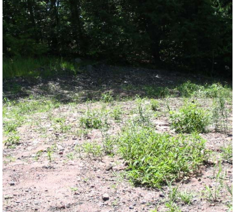
Lambert Rd: A view of 115kV restoration efforts near structure #3863. Some vegetative growth has been observed.
