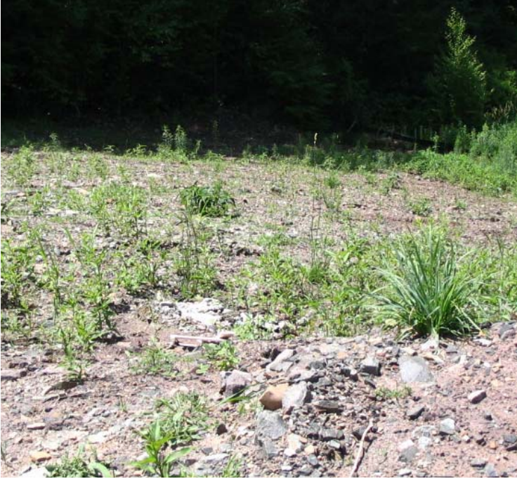
Lambert Rd: Vegetative growth has been noted and soils appear stable along the slope near structure #3863.
