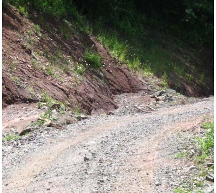
Old Ln: Sediment basins along the access road need attention.
