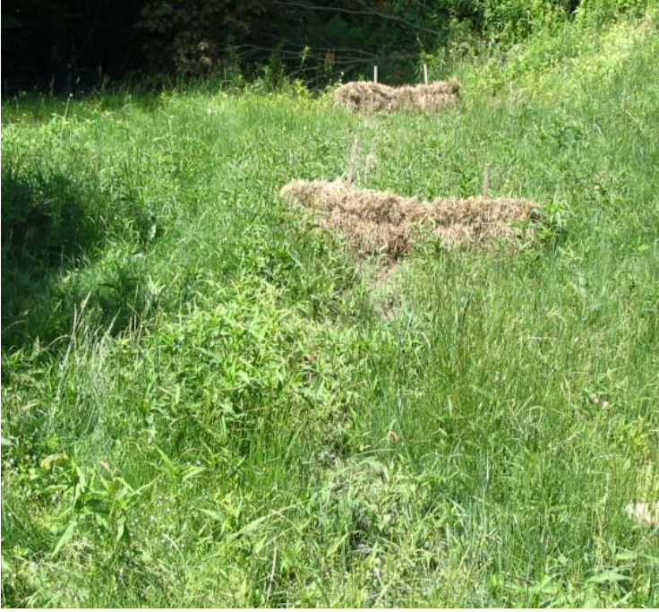
Wheelers Farm Rd (Milford): Vegetation covers approximately 80-85% of the restored area near structure #3832. However, channelized flow from stormwater runoff continues here. Controls remain functional.
