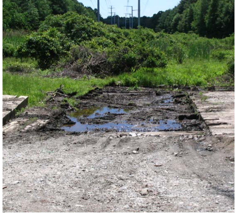
Clearview Ln (Woodbridge): Timber mat removal and 115/345 kV restoration efforts have begun in this area.
