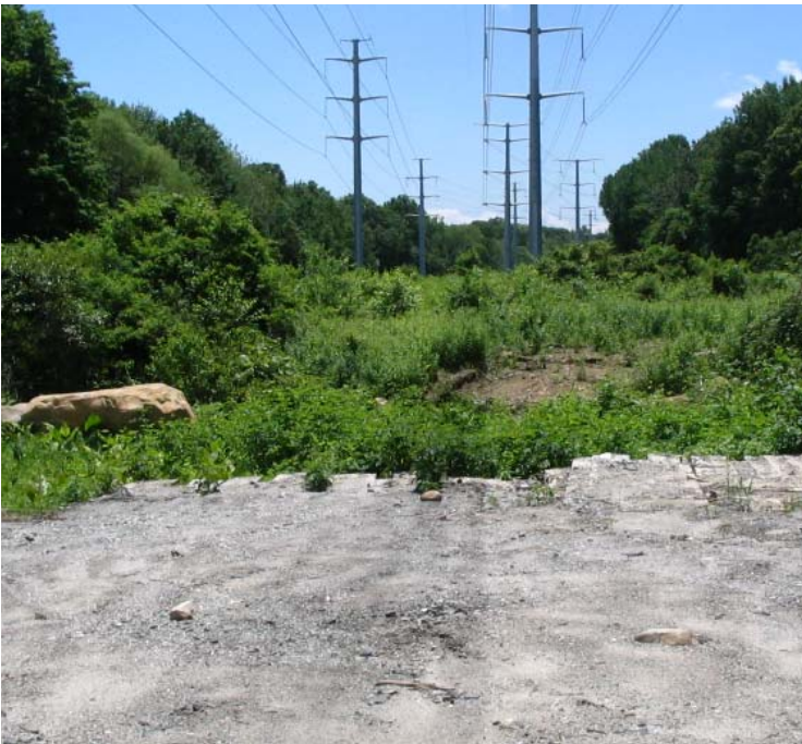
Rimmon Rd (Woodbridge): Vegetative growth has been noted and soils appear stable where timber mats were used to cross a stream near structure #3918.
