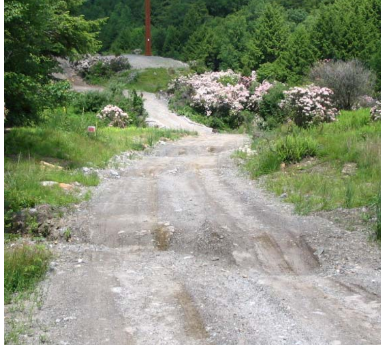
Litchfield Turnpike: Waterbars and sediment basins remain functional within the access road in this area.
