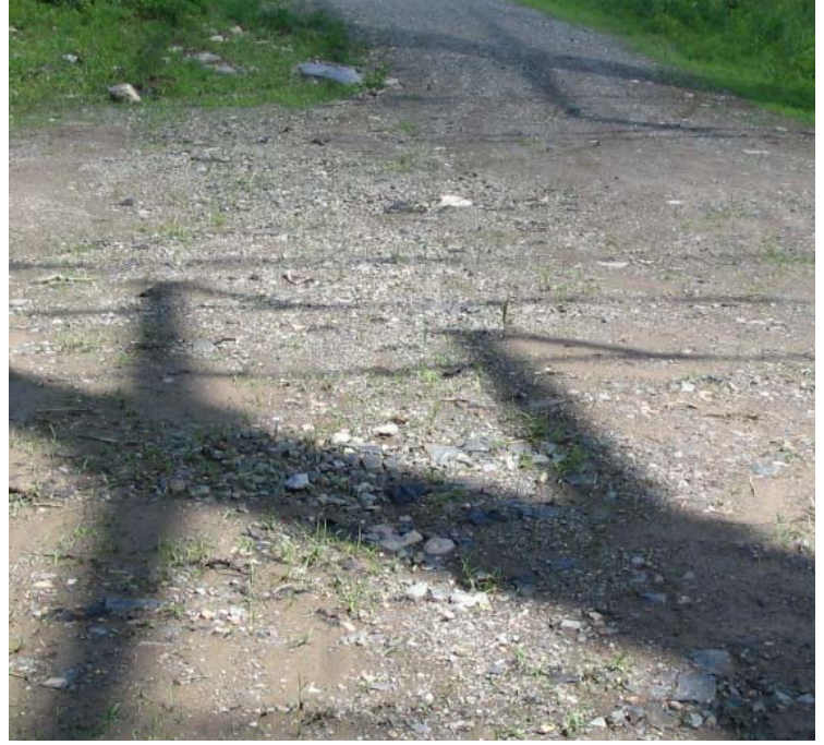
Wheelers Farm Rd: Stormwater flows across the crane pad resulting in channelized flow near structure #3832.
