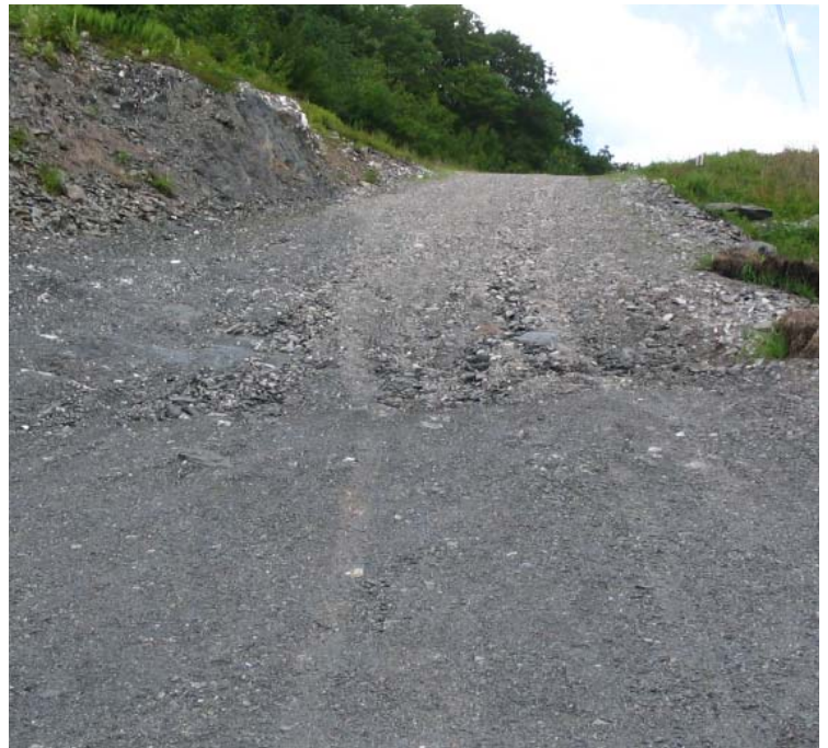
Litchfield Turnpike (Bethany): The waterbar near structure #24148 remains functional.
