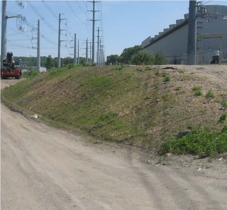
Caswell St (Milford): Vegetative growth has been noted and soils appear stable along the slope near structure #3887.
