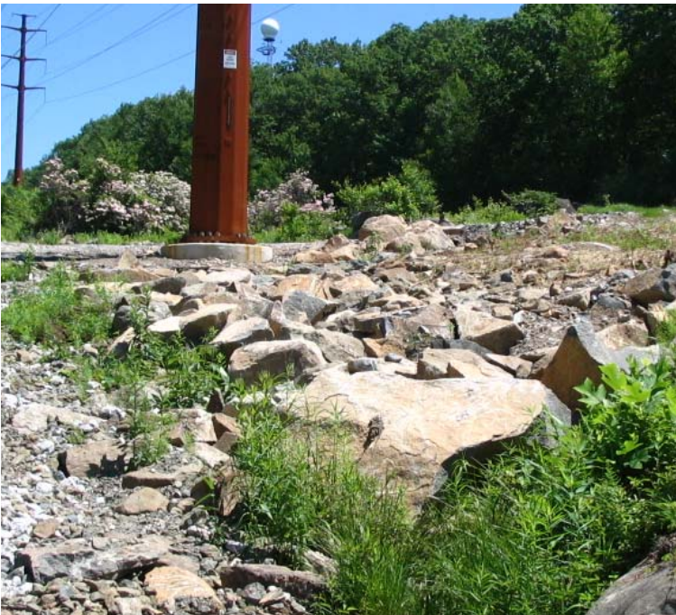
Downs Rd: An additional view of the rip-rap controls near structure #3982. There is a culvert inlet here that collects runoff from the eastern side of the access road.
