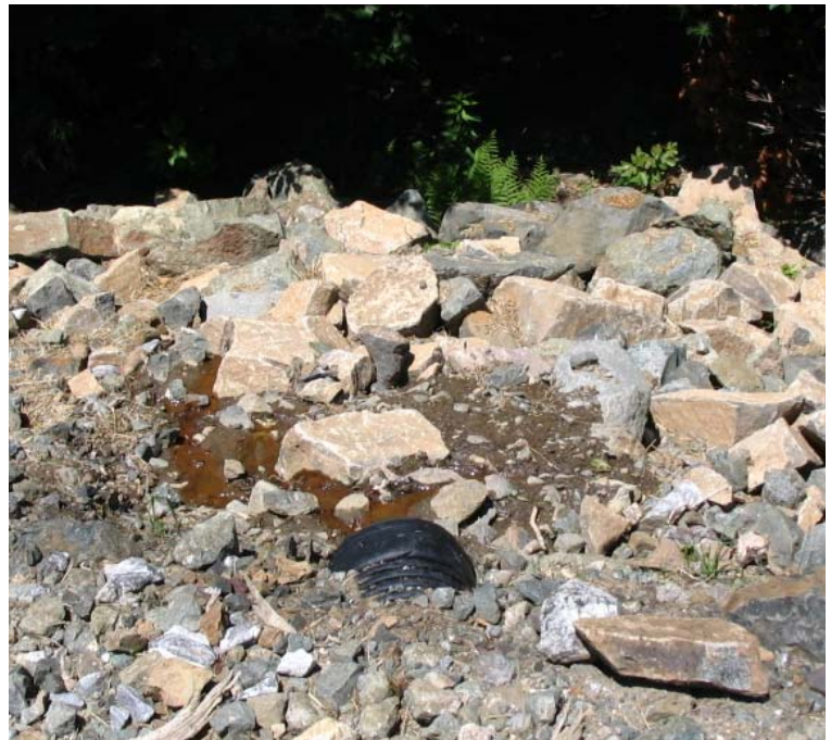
Downs Rd: A view of the culvert outlet and rip-rap controls located on the western side of the access road near structure #3982.
