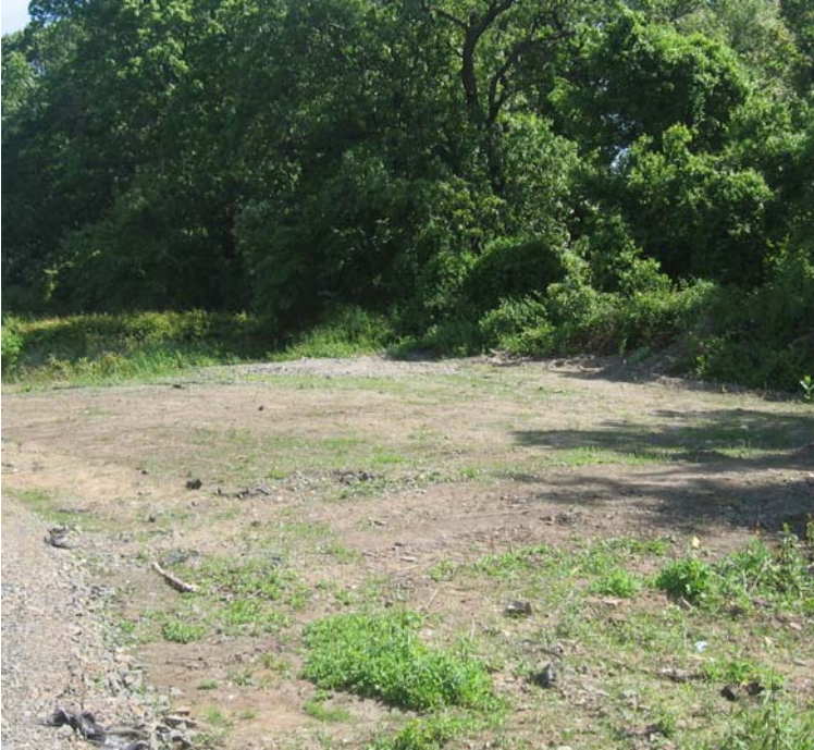
Naugatuck Ave: A view of 115kV restoration efforts near structure #3803. Some vegetative growth has been observed.
