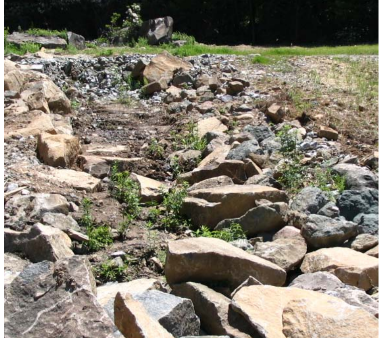
Downs Rd (Bethany): Rip-rap controls continue to function near structure #3982.
