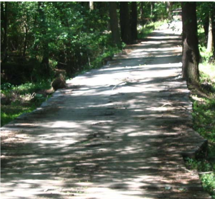
Clearview Ln: An additional view of the timber mats used to cross wetland #138.
