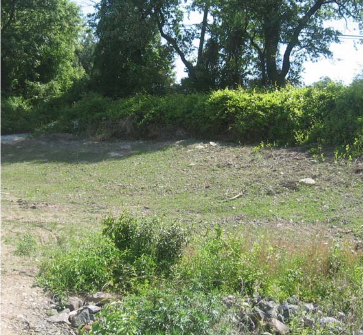
Naugatuck Ave: A view of 115 kV restoration efforts near structure #3804. Vegetative growth has been observed here.
