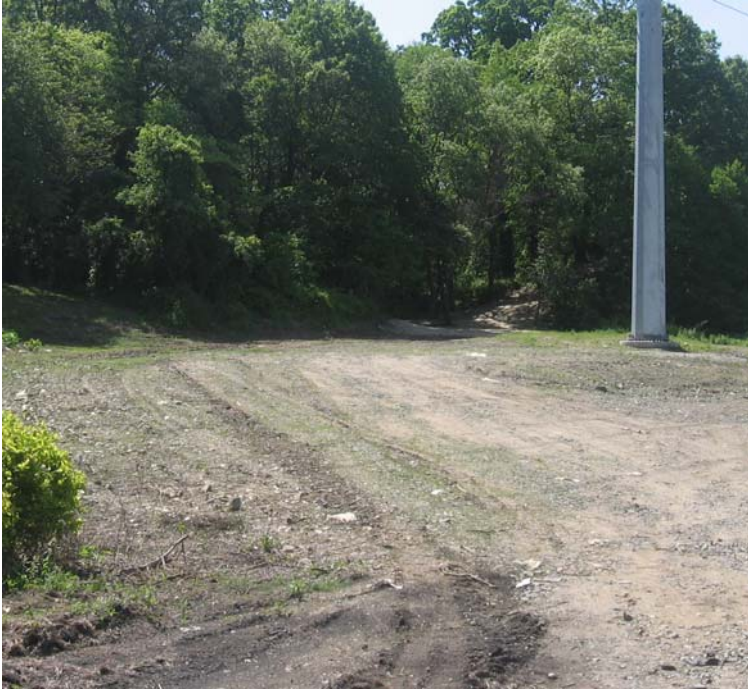
Naugatuck Ave: A view of 115kV restoration efforts near structure #3802. Some vegetative growth has been observed.
