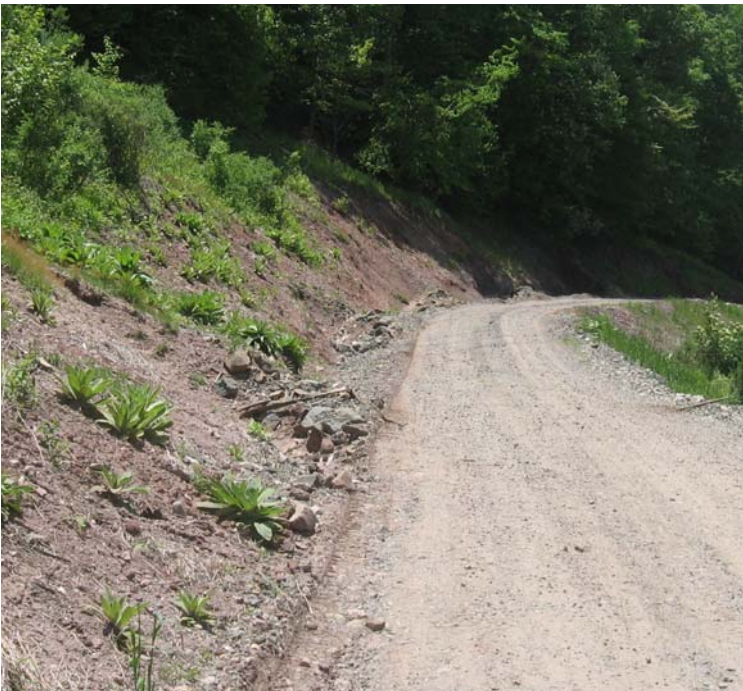
Old Ln: Access road controls remain functional on the slope in this area.
