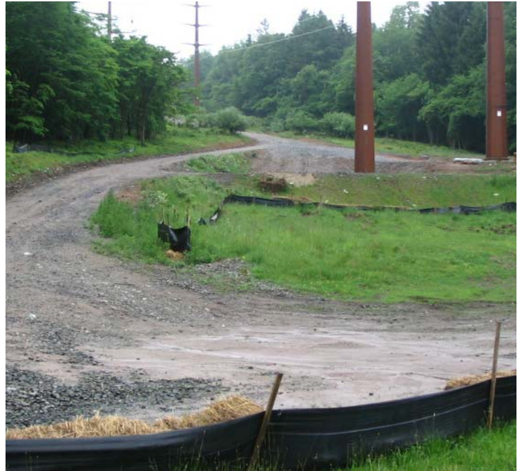
Dogburn Rd (Orange): A view of the access road near structures #3890/24077. Sediment accumulation was observed against the silt fence controls above Maltby Lake.
