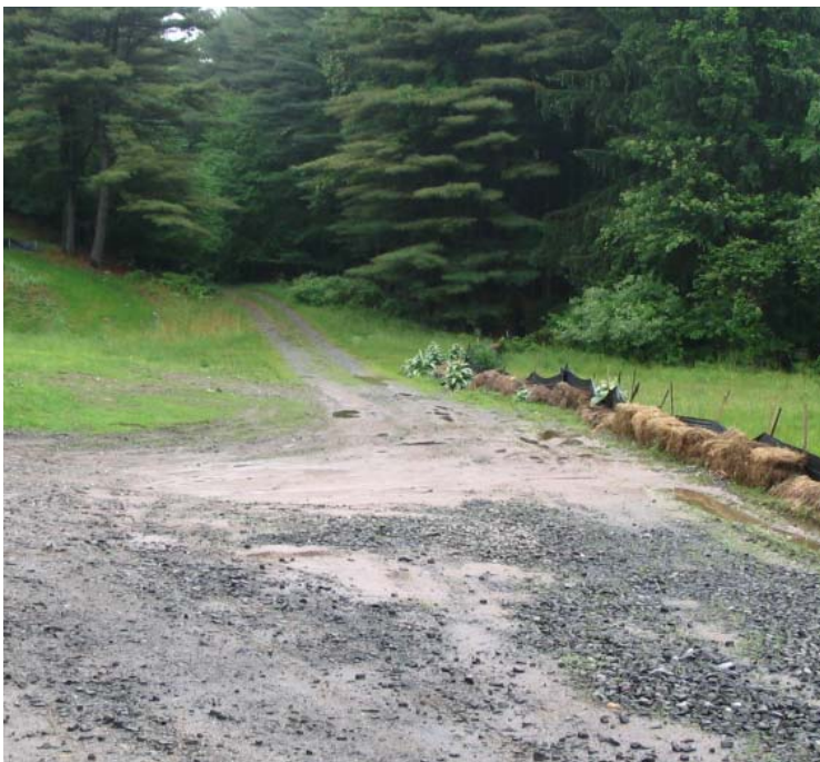
Dogburn Rd: An additional view of sediment accumulation within the access road near structures #3890/24077. Silt fence controls remain functional in this area.
