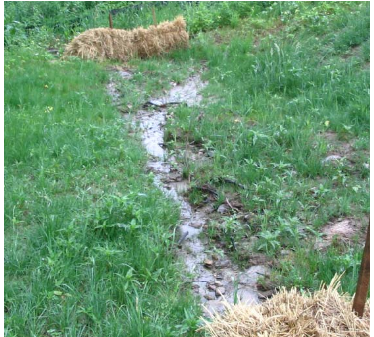
Wheelers Farm Rd (Milford): Channelized flow was observed near structure #3832. Controls remain functional in this area.
