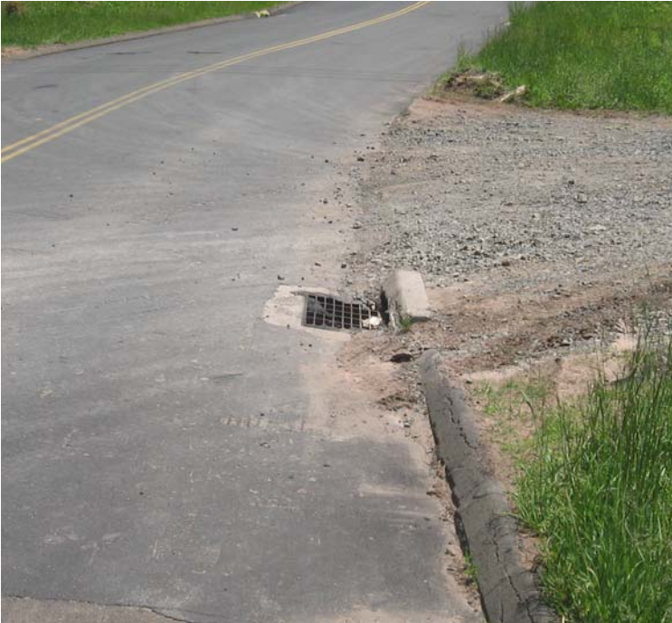
Old Ln (Hamden): No catch basin protection has been provided here.
