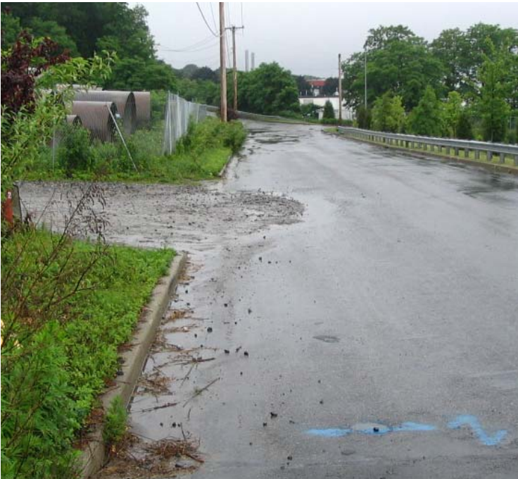
Shelland St (Milford): Some sediment tracking was observed at the storage yard entrance on Shelland St.
