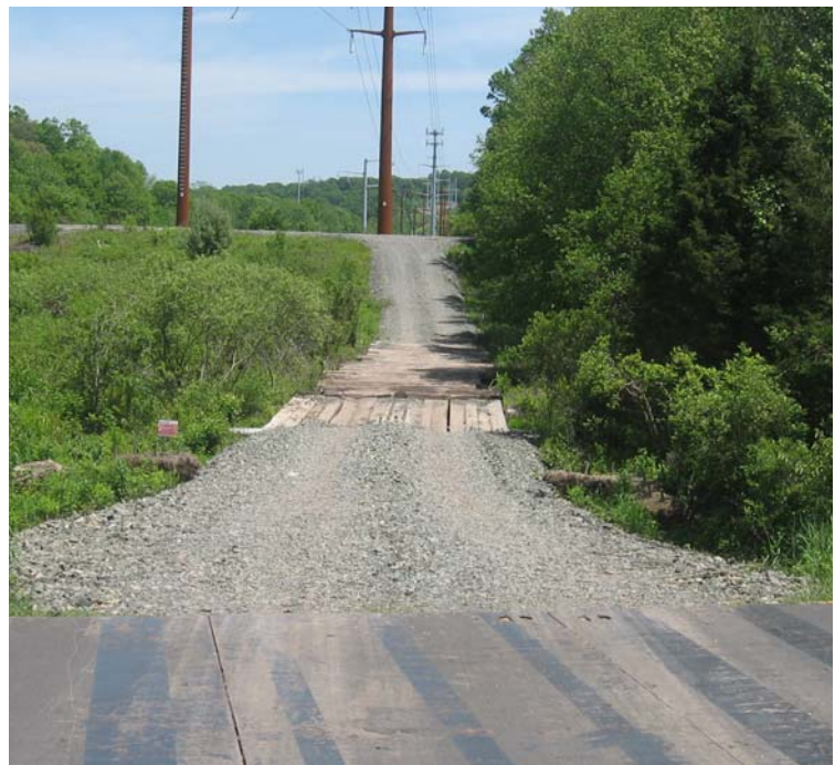
Brooksvale Ave north (Hamden): The wetland timber mat crossing remains in this area.
