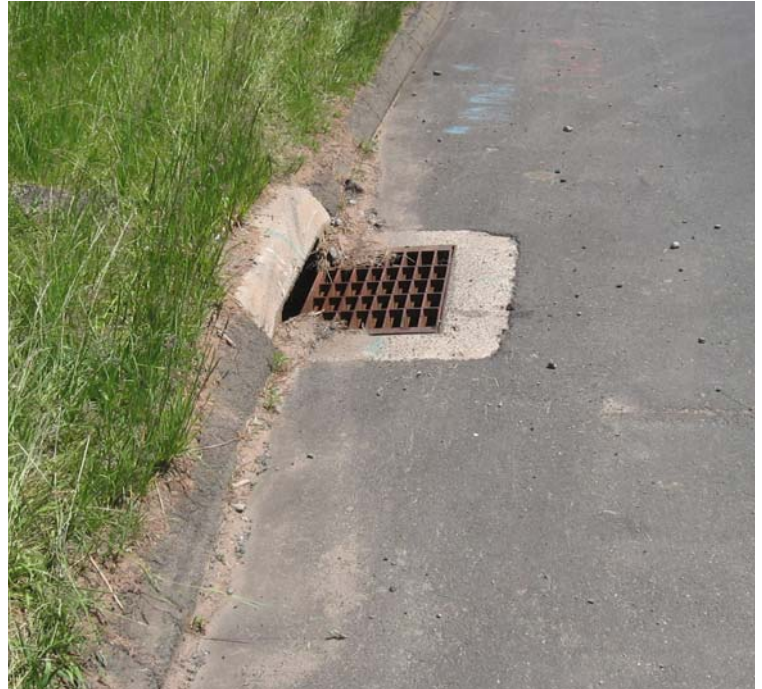
Old Ln: No protection has been provided for the catch basin located on the west bound side of Old Ln.
