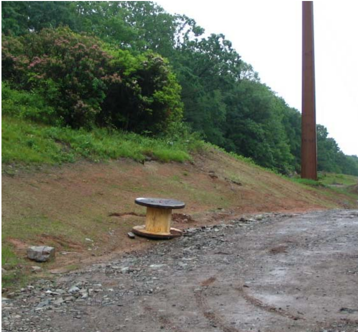
Rt 34 (Orange): Vegetation growth has been observed along the slope near structure #3887.
