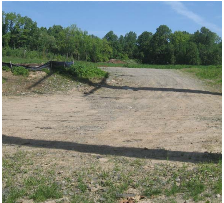
Wheelers Farm Rd: Ground water is no longer flowing across the access road and crane pad near structure #3832. However, stormwater continues to channelize within the ROW.
