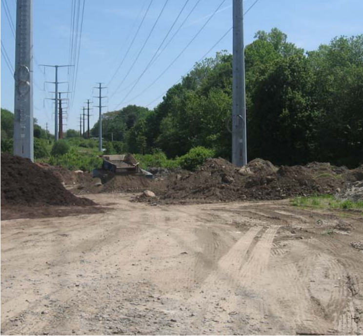
North St (Milford): A view of non-project related activity within the ROW near structure #3845/24032. This activity is within the wetland buffer.
