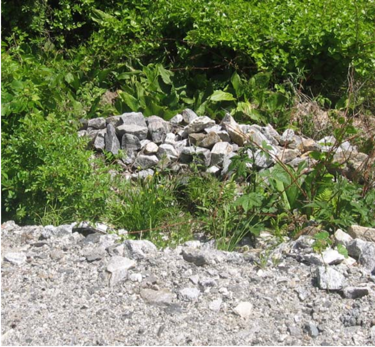
Gaylord Mtn Rd north: A view of the first culvert outlet and sediment basin along the access road. No sediment accumulation was noted here.
