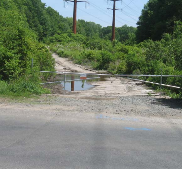
Pine Tree Dr (Orange): Timber mats remain within the wetland areas here.
