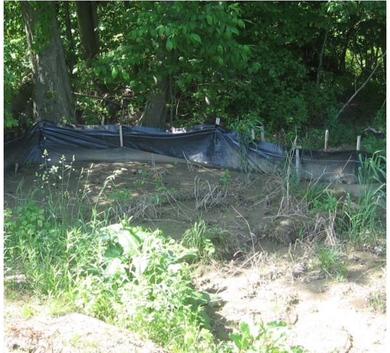
Wheelers Farm Rd: No further sediment accumulation has been observed within the controls near structure #3832.
