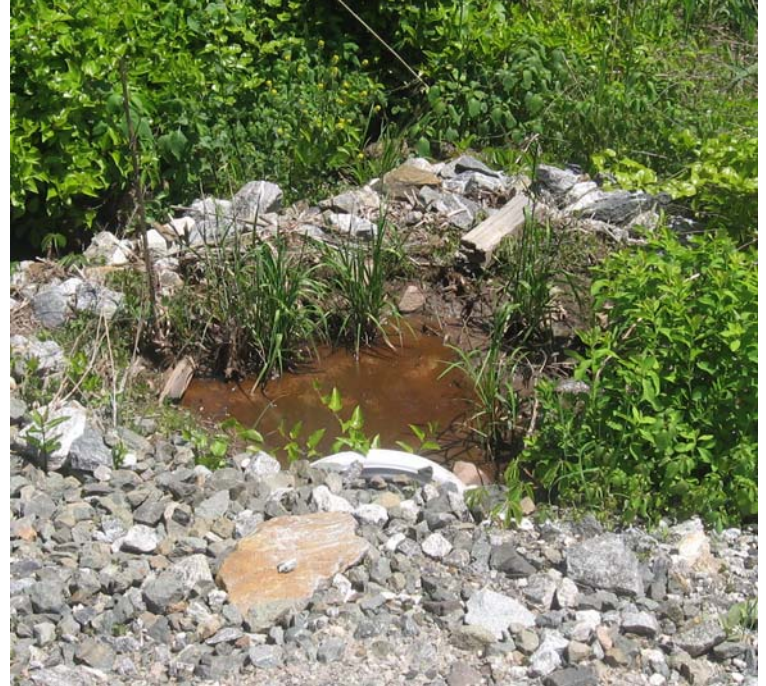
Gaylord Mtn Rd north: A view of the third culvert outlet and sediment basin located adjacent to the access road. Sediment accumulation has been noted within the basin here.
