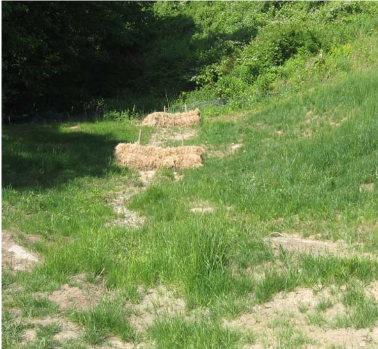
Wheelers Farm Rd (Milford): Grass growth was observed within the erosive gully near structure #3832.
