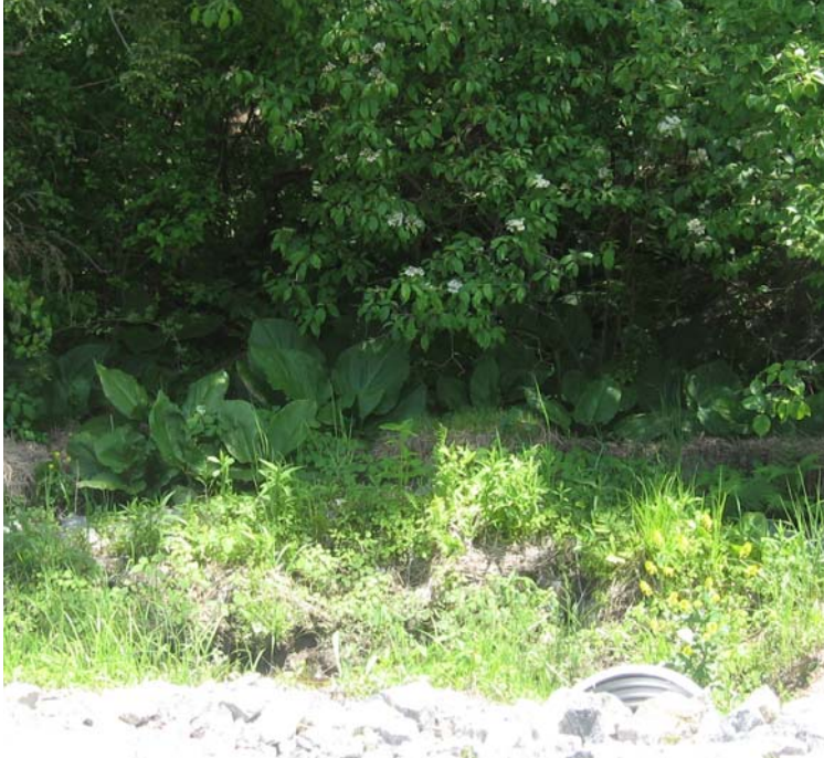
Gaylord Mtn Rd north: A view of the second culvert outlet and sediment basin located adjacent to the access road. Wetland vegetation has been noted in this area. Sediment has accumulated within the sediment basin.
