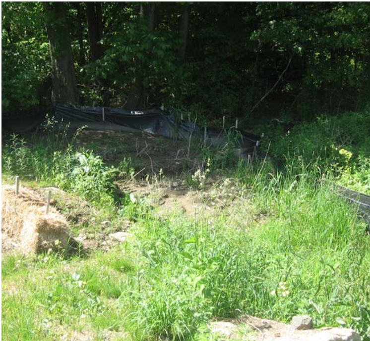
Wheelers Farm Rd: An additional view of the silt fence near structure #3832.
