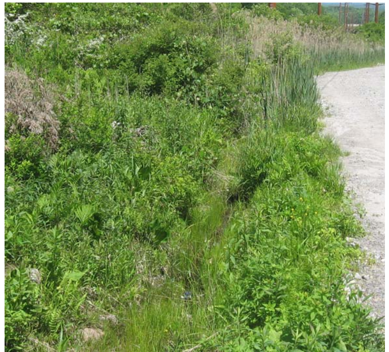
Gaylord Mtn Rd north: An additional view of the vegetative growth within the trench along the access road.
