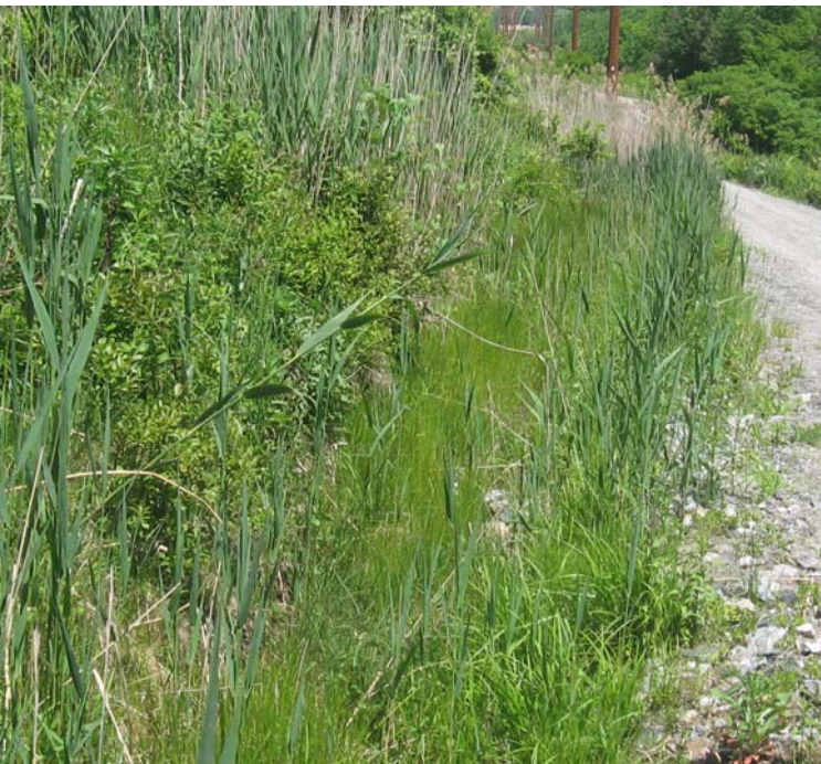
Gaylord Mtn Rd north (Hamden): Vegetative growth was observed within the trench located along the access road.
