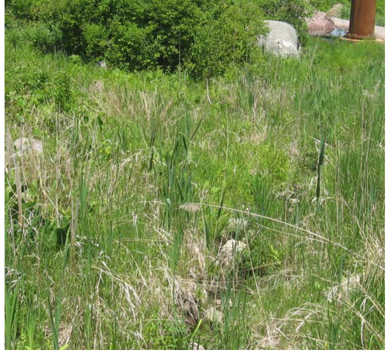
Gaylord Mtn Rd north: An additional view of the trench located along the access road. Vegetation growth has been noted.
