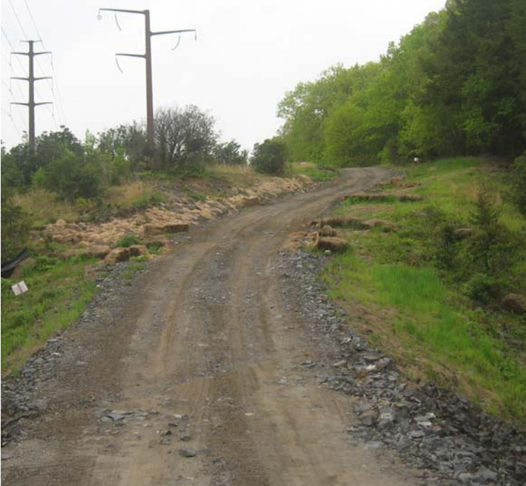
Litchfield Tpk: Access road controls remain functional near the wetland crossing between structures #24156-157.
