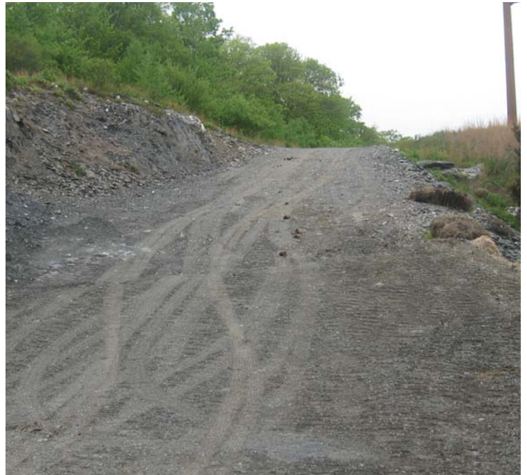
Litchfield Tpk: Access road controls (i.e waterbars) remain functional near structure #24148.
