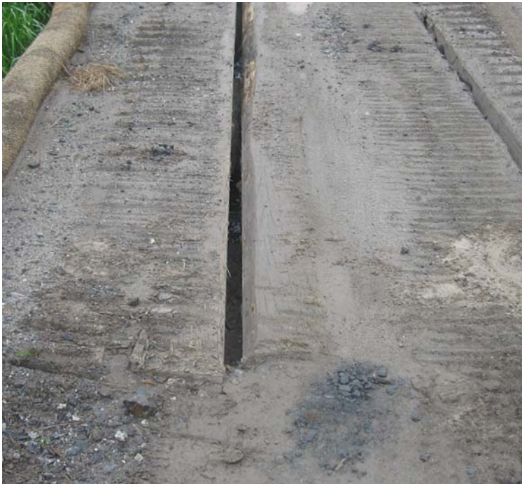
Litchfield Tpk: A view of sediment accumulated on the timber mat crossing between structures #24153-154.
