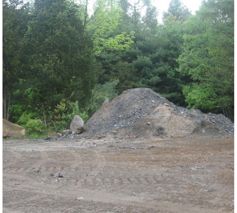
Hatfield Road north (Bethany): Spoil piles remain within upland portions of the ROW. Spoils in this area appear to be contained on site.
