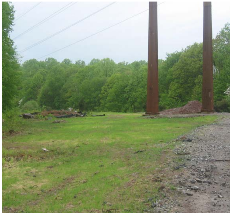
Brooksvale Ave (Hamden): A view of 115 kV restoration efforts near structure #4004. Spoils remain in upland portions of the ROW in this area. Spoils appear to be contained on site.
