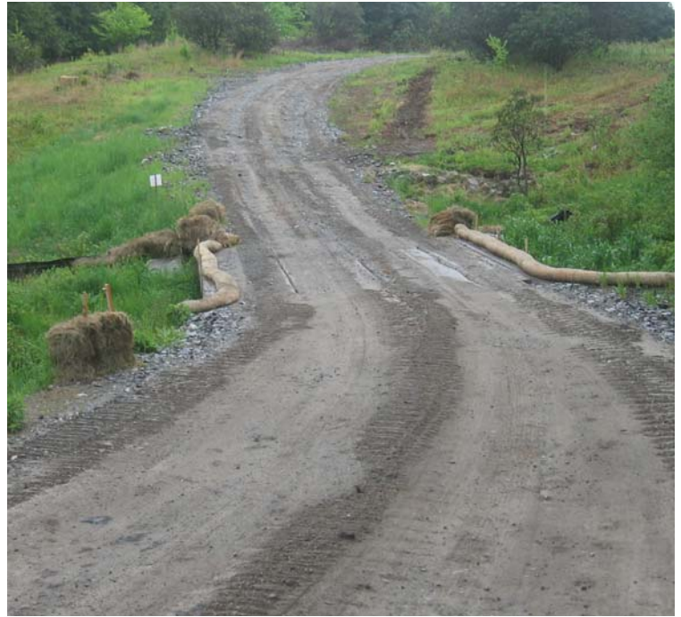
Litchfield Tpk: Access road controls (i.e waterbars) continue to function at the wetland crossing between structures #24152-153. Sediment continues to accumulate on the timber mat crossing here.
