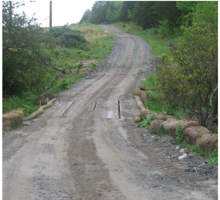
Litchfield Tpk: A view of the timber mat crossing between structures #24154-155. A culvert remains beneath the timber mats here, which allows for water flow.
