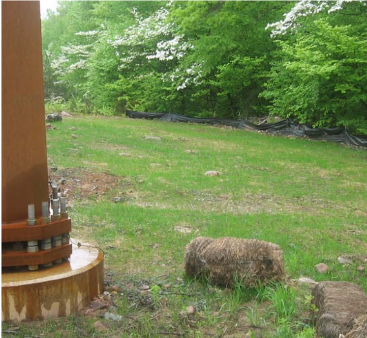
Tom Swamp Rd (Hamden): A view of 115 kV restoration efforts near structure #4002.
