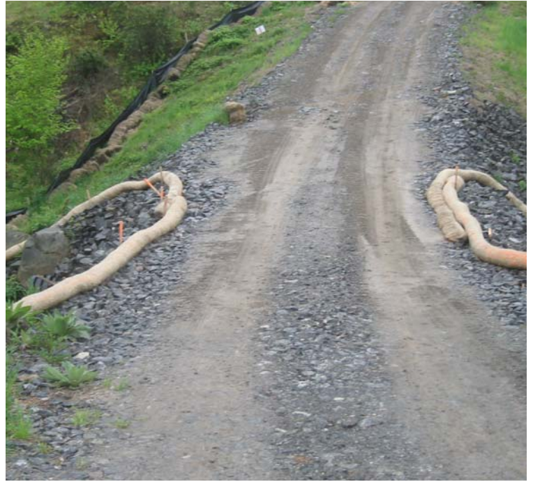
Litchfield Tpk: A view of the wetland crossing between structures #24156-157. Erosion controls remain functional.
