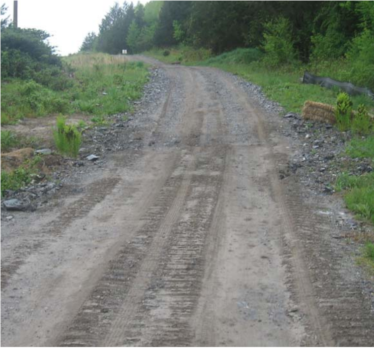
Litchfield Tpk: Access road controls (i.e waterbars) remain functional at the wetland crossing between structures #24154-155.
