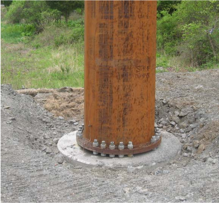
Litchfield Tpk: Stormwater controls have been installed at the base of structure #24148.
