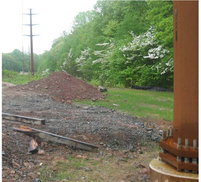
Tom Swamp Rd: Spoil piles remain within the ROW in this area. Spoils appear to be contained in upland portions of the site.
