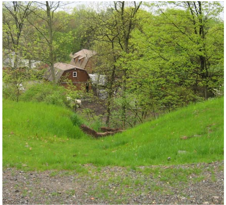
Fresh Meadow Ln (Milford): The vegetated swale near structure #3835 appears stable at this time.
