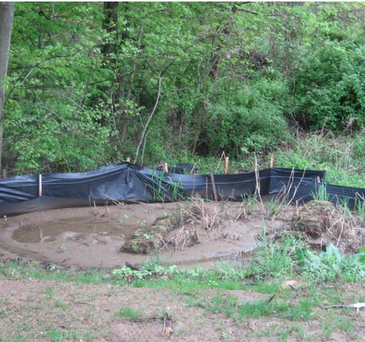
Whealers Farm Rd: Silt fence controls are nearing capacity near structure #3832.
