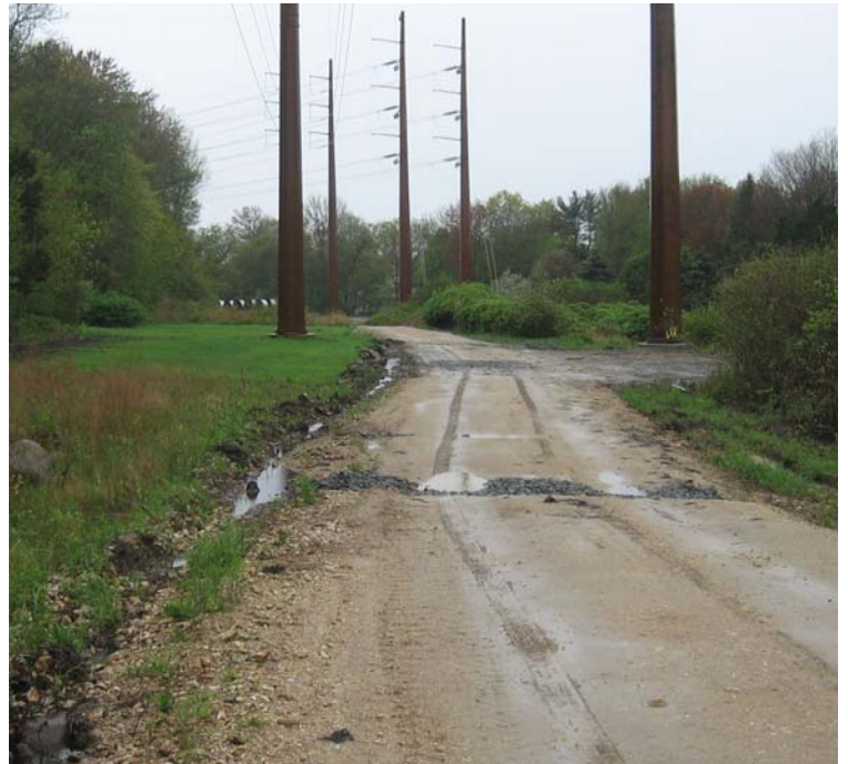
Russell Ave (Orange): A trench was installed along the access road in this area to help control stormwater runoff. Vegetation growth has been noted in this area near 115 kV structures.
