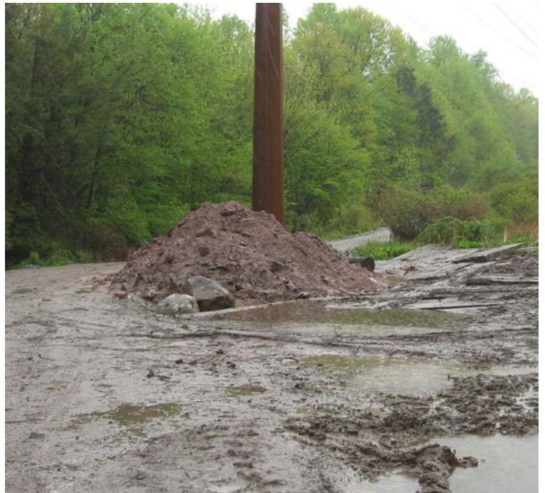
Gaylord Mtn Rd (Hamden): A spoil pile remains in the wetland area near structure #24179.
