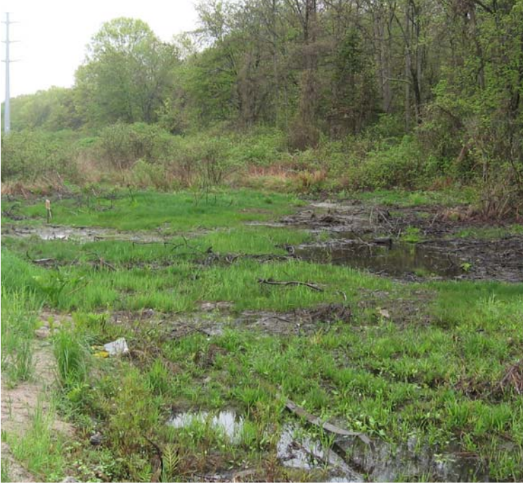
West River St (Milford): A view of 115 kV restoration efforts near structure #3837.
