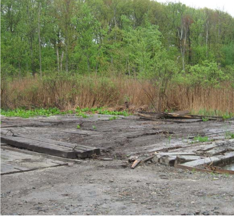
Hunting Hill Rd (Orange): Wetland timber mats remain for access to structures #3881/24068.
