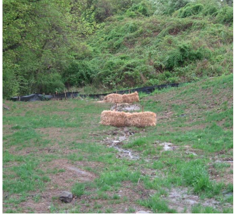
Whealers Farm Rd (Milford): Haybale controls have been added to help control stormwater runoff near structure #3832.
