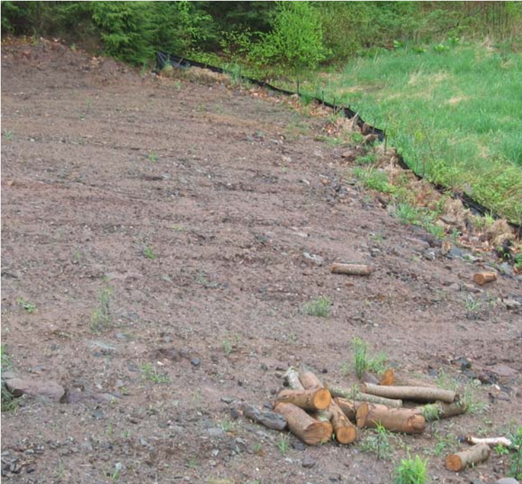
Lambert Rd (Orange): Grading/115 kV pad reclamation continues near structure #3863 in order to decrease the slope on the southern side of the crane pad. Exposed soils appear stable at this time.
