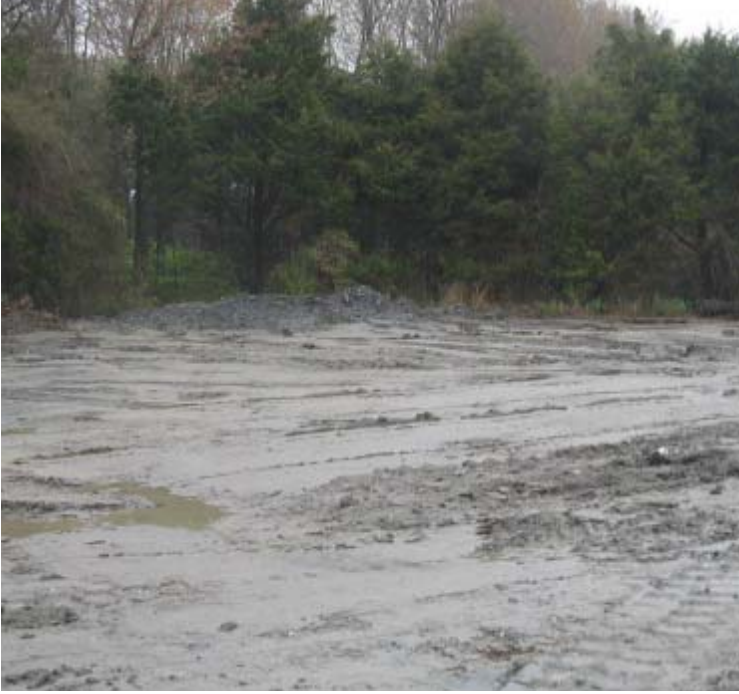
Brookwood Ave (Woodbridge): Spoils have been removed from the ROW near structure #24096.
