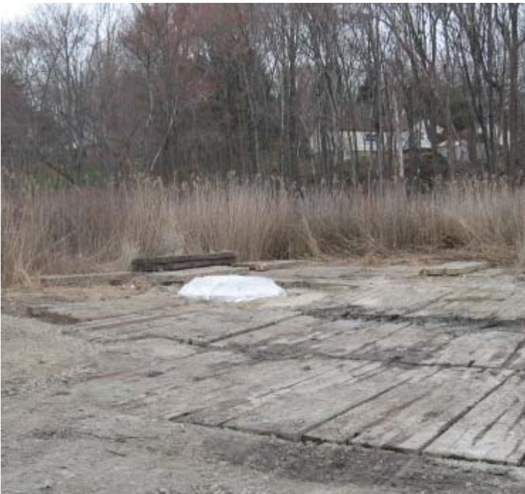
Hunting Hill Rd (Orange): Structure #24068 has been installed in the wetland here, as approved.
