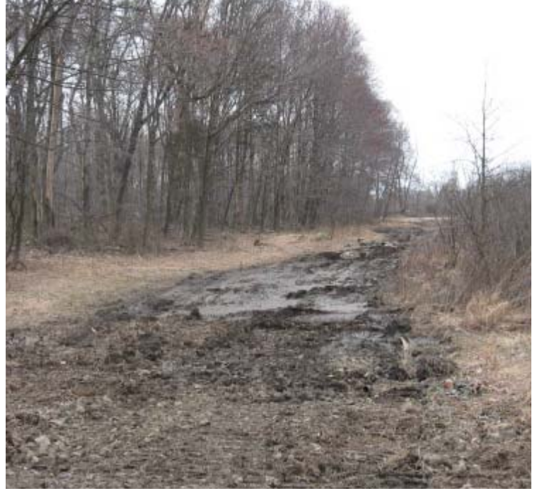
Pease Rd (Woodbridge): The tire ruts located within the abandoned portion of the ROW have been graded.
