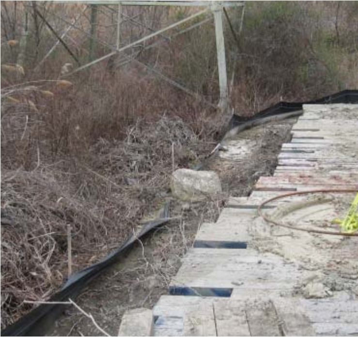
Naugatuck Ave (Milford): Silt fence is in need of repair near structure #3804.
