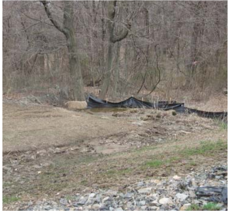
Whealers Farm Rd (Milford): Perimeter controls are nearing capacity and the erosive gully remains.
