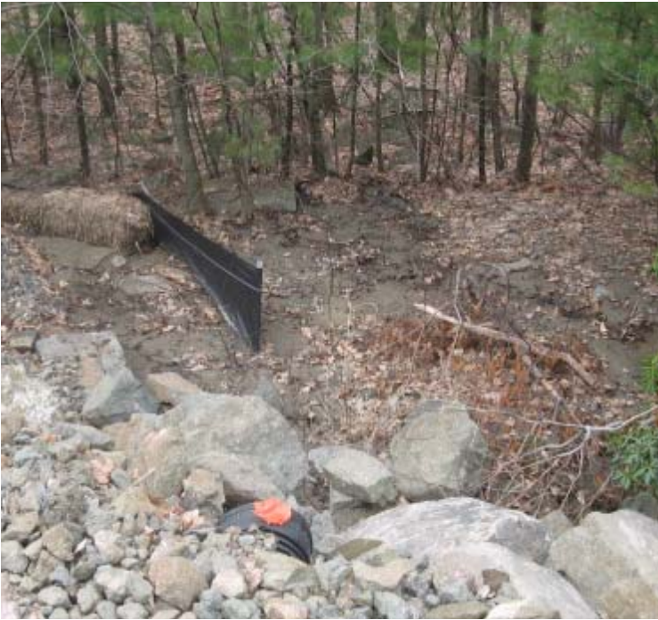
Downs Rd (Bethany): Sediment laden runoff is bypassing controls near structure #24169.
