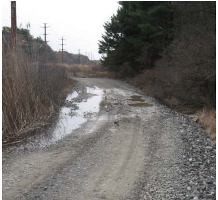
Clearview Ln (Woodbridge): Sediment laden storm water is flowing across the access road and into the adjacent wetland.
