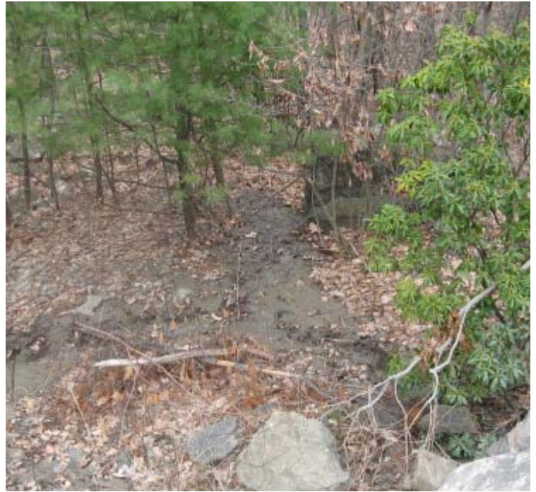
Downs Rd: An additional view of sediment migrating off the ROW near structure #24169.
