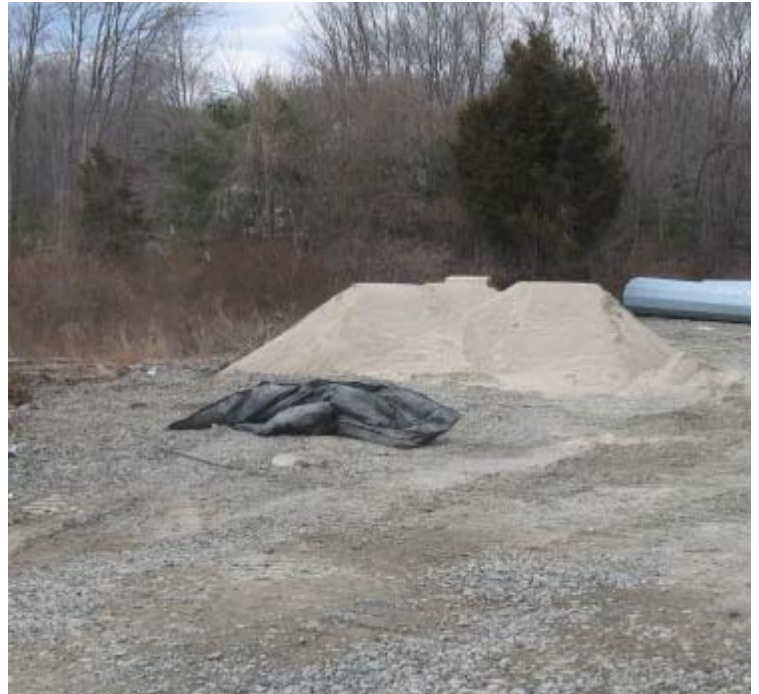
Oak Ln (Woodbridge): Sand, used for foundation installation, remains piled upgradient of the wetland near structure #24092.
