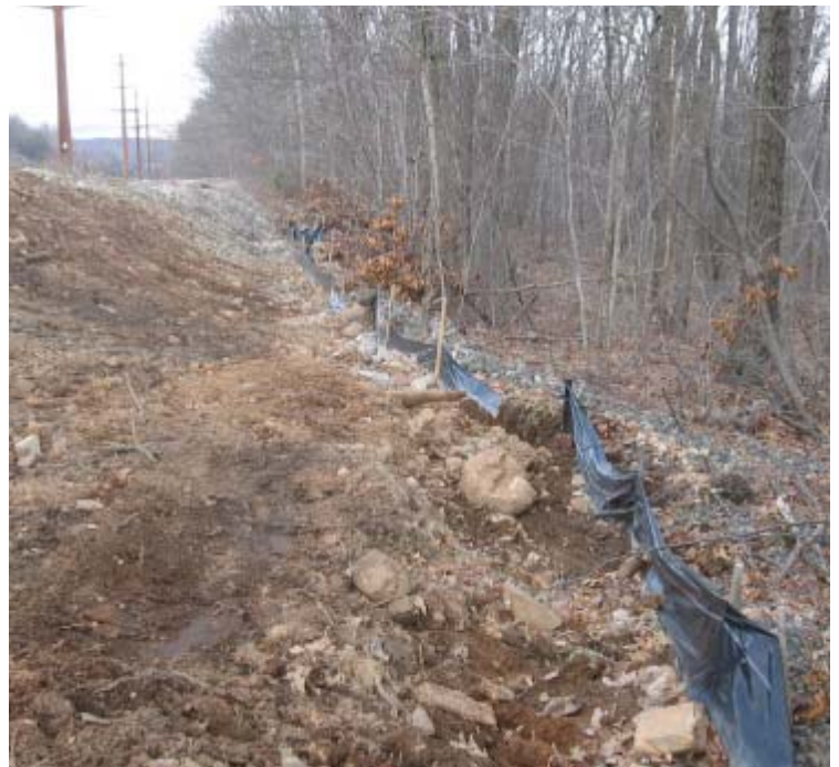
Gaylord Mtn Rd: An additional view of ROW perimeter controls. Stone and waterbar trenches were added in this area to help control stormwater runoff.
