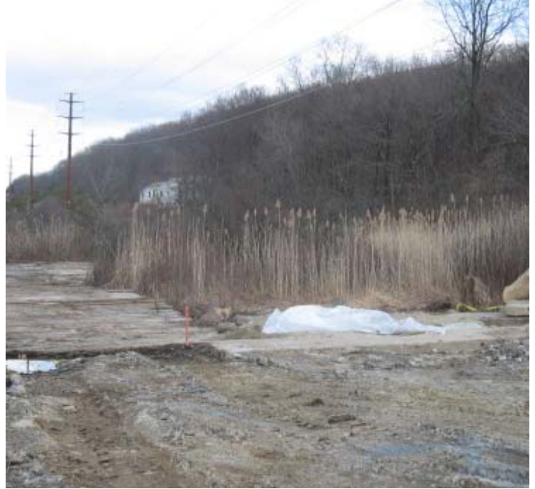
Hatfield Rd (Hamden): Structure #24166 has been installed within wetland #109. Additional timber mats were placed in the wetland here to gain access for lattice tower removal.
