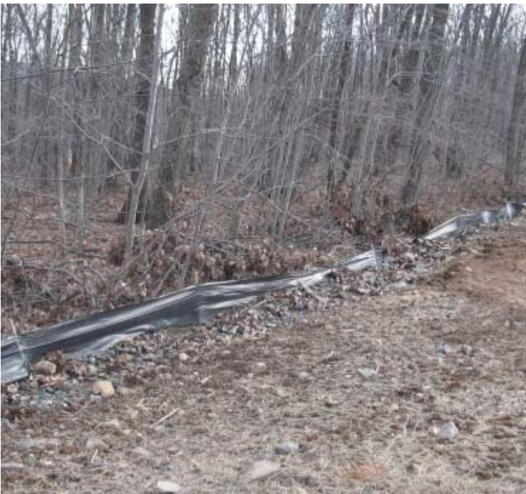
Gaylord Mtn Rd (Hamden): ROW perimeter controls remain functional but are nearing capacity in some locations.
