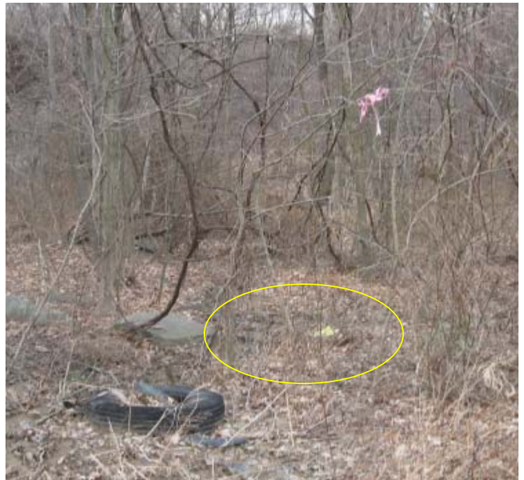
Wheelers Farm Rd: A small amount of sediment has migrated off the ROW near structure #3832.
