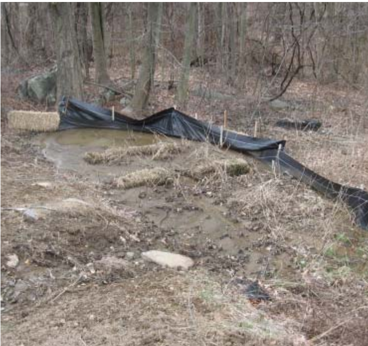
Wheelers Farm Rd: Silt fence controls are in place but haybale controls are at capacity near structure #3832.
