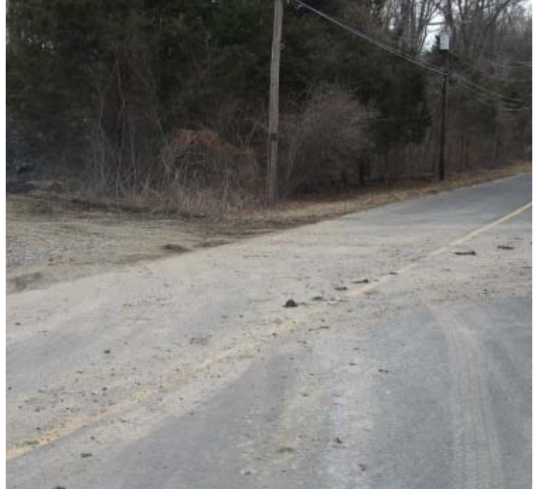
Brookwood Dr: Sediment tracking was evident here this week.
