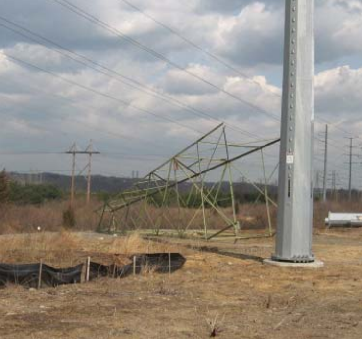
Naugatuck Ave (Milford): Lattice tower removal continues in this area (Naugatuck to Oronoque).
