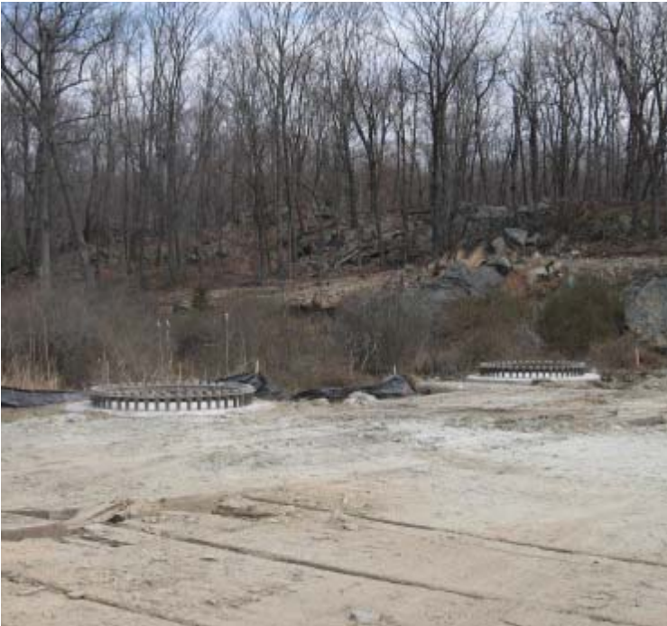
Route 34 (Orange): Two foundations have been installed in a wetland for structure #24072.
