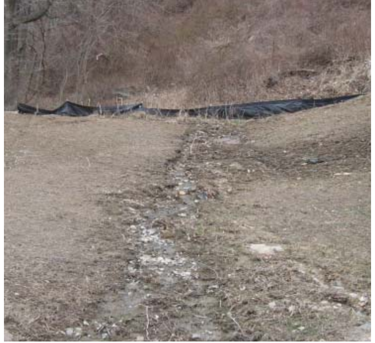
Wheelers Farm Rd (Milford): An erosive gully was noted near structure #3832.
