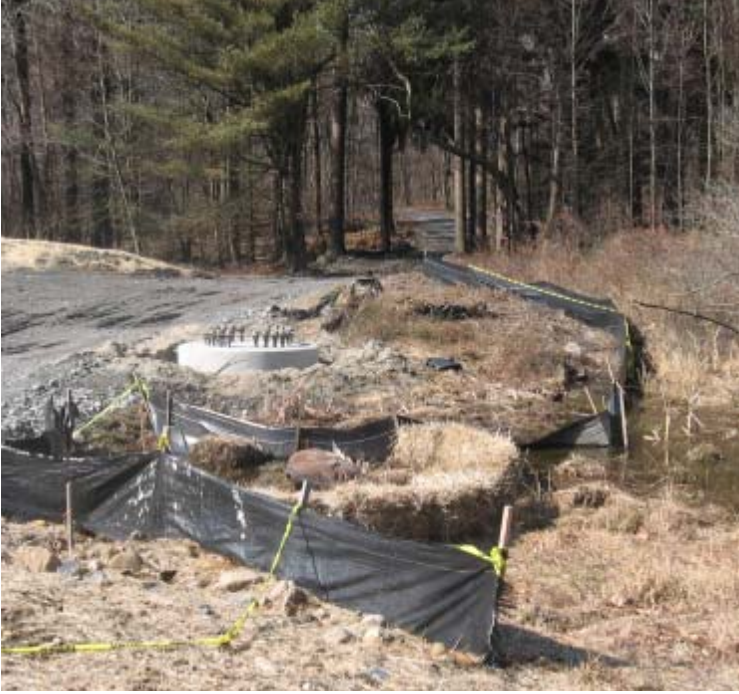
Clearview Ln (Woodbridge): The foundation for structure #24090 has been installed. The foundation is located on the edge of a wetland.
