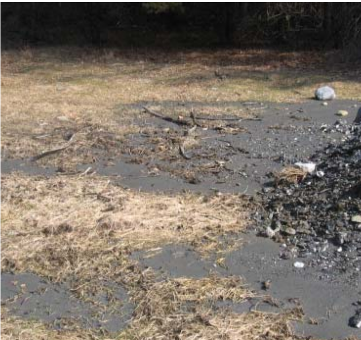
Clearview Ln: Sediment has begun to migrate from the spoil pile near structure #24090.
