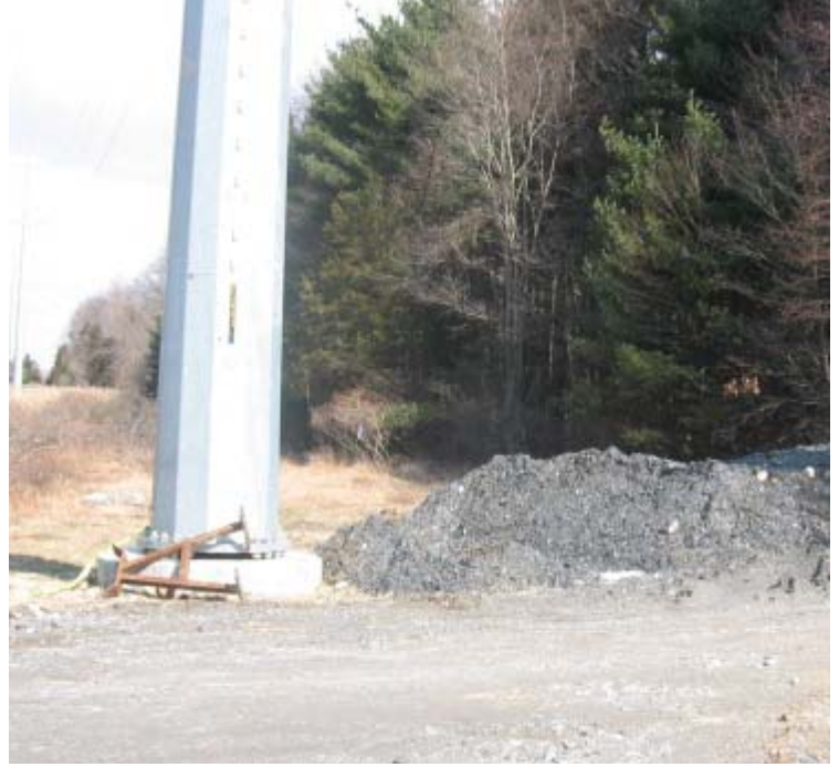
Clearview Ln: Spoils from structure #24090 remain piled in a wetland buffer. No controls have been installed to contain the pile.
