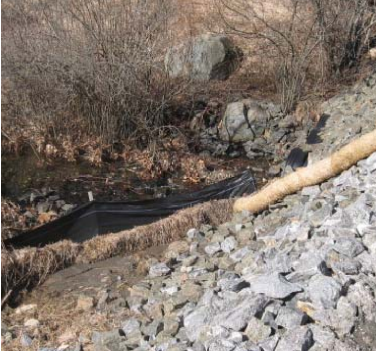
Litchfield Turnpike (Bethany): Access road controls are functioning properly, at the stream crossing, between structures #24156-57. Due to the proximity of the controls to the stream channel, sediment should be removed from the controls.
