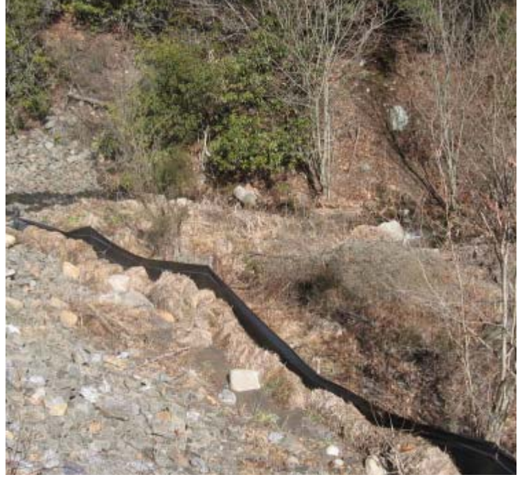
Litchfield Turnpike: A view of the controls on the opposite side of the stream crossing between structures #24156-57. Sediment is accumulating against the controls.
