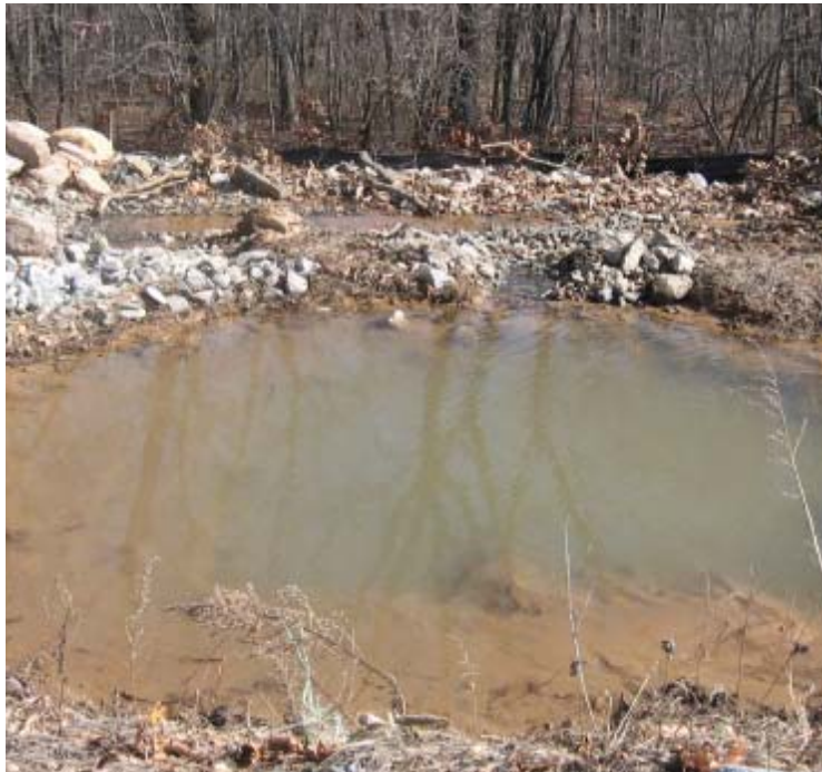
Gaylord Mtn Rd (Hamden): Sediment was removed from the basin near structure #3989.
