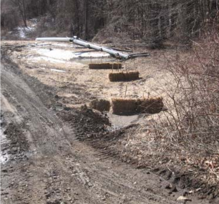
Glen Dam (Woodbridge): Access road controls have been improved. Water bars were re-established, hay bale check dams were installed, terracing was implemented, and mulch was applied as a temporary stabilization measure.
