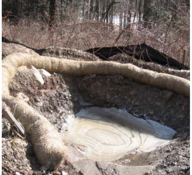
Glen Dam: Sediment has been removed from the basins along the access road, returning function to the sediment basins.
