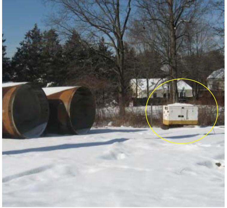
Racebrook Rd: A gas powered generator remains in the wetland area here.
