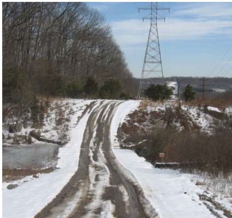
Brooksvale Ave (Hamden): Excess sediment remains accumulated on the timber mat crossing at wetland #100. Additional controls are recommended for this area.
