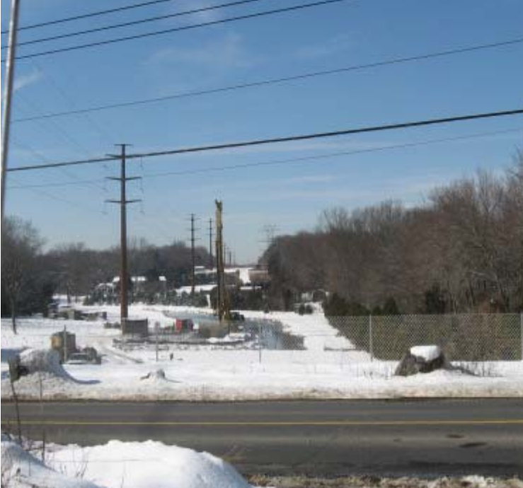
Dogwood Rd (Orange): Drilling has begun for proposed structure #24065. Proper controls are in place to protect the wetland in this location.
