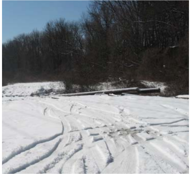
Rimmon Rd (Woodbridge): A disassembled "H" frame structure remains in the wetland area near structure #24105.
