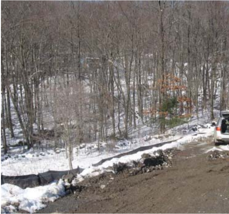
Route 34: Silt fence controls remain in place in order to protect the wetland in this area (near structure #24074).
