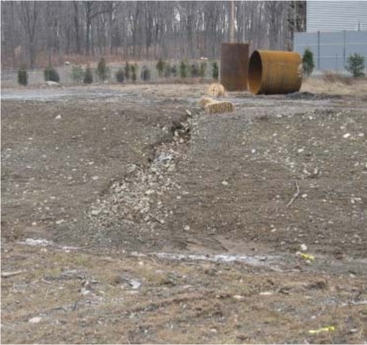
Plains Rd (Milford): Stormwater runoff has eroded the slope of the drainage swale between the ROW and the East Devon Substation.
