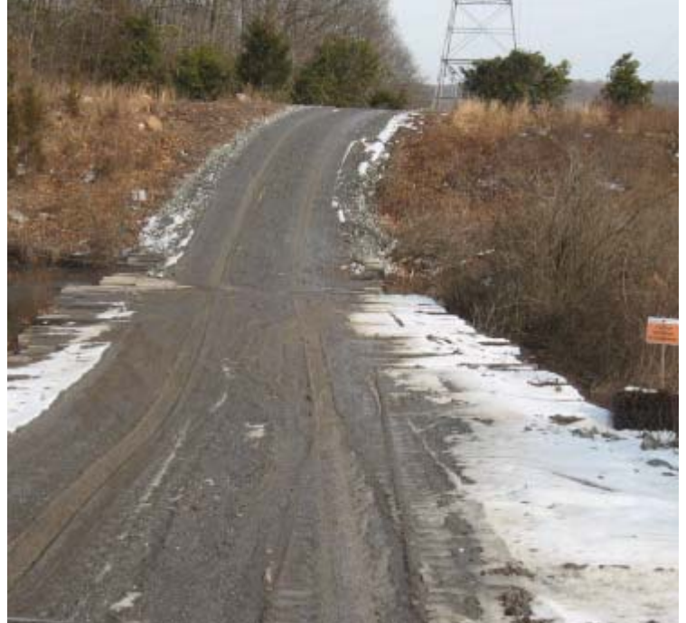
Brooksvale Ave: A view of sediment accumulation on the timber mat crossing. Controls are needed on both sides of the access road, near wetland #100.
