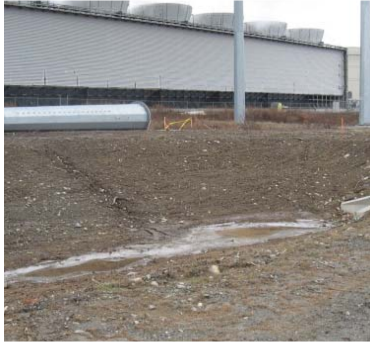
Plains Rd: An additional view of the slope erosion within the drainage swale.
