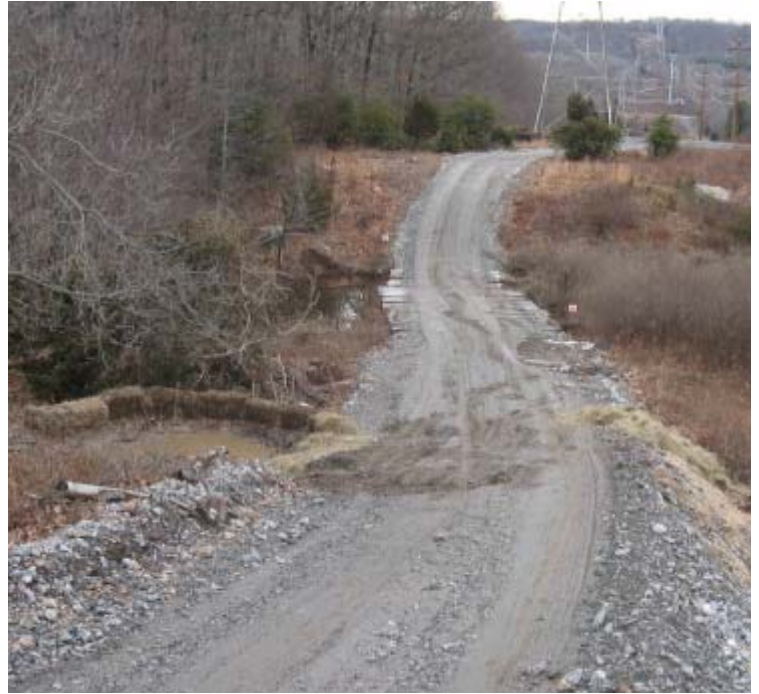
Brooksvale Ave (Hamden): Sediment from the access road has accumulated on the timber mats here. Some sediment has seeped through the mats and into the wetland.
