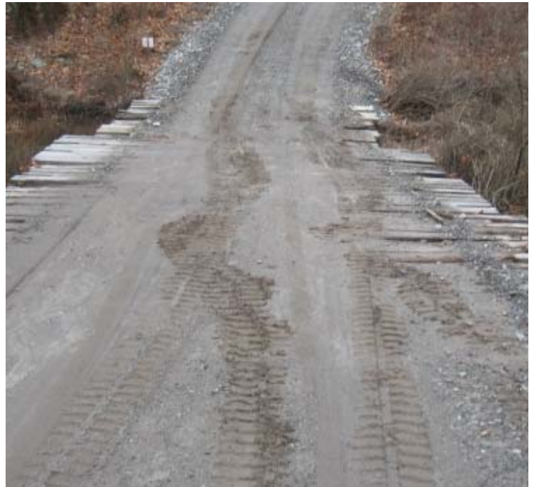
Brooksvale Ave: Additional view of sediment accumulation on the timber mats.
