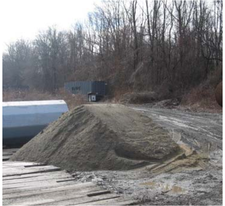
Manville Rd (Woodbridge): Sand, used during foundation installation, is being stored on the access road in this wetland area near structure #24103.
