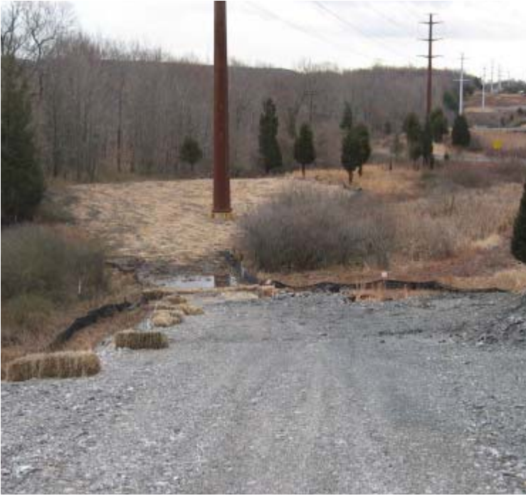
Litchfield Turnpike (Bethany): Wetland timber mats and the stone crane pad have been removed near structure #3961. Exposed soils have been graded and temporarily stabilized with mulch.
