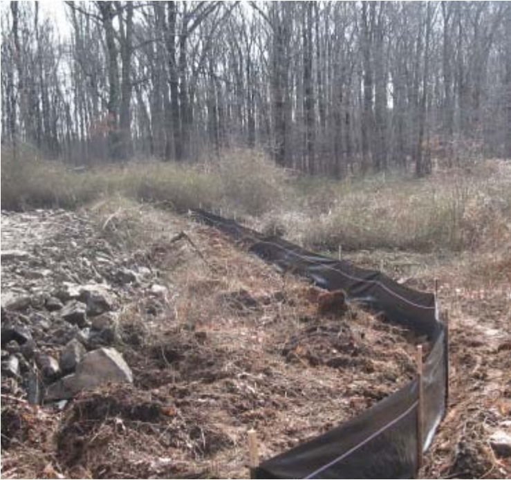
Route 34 (Orange): A new "line-pulling pad" was installed within the wetland buffer here. Proper controls are in place.
