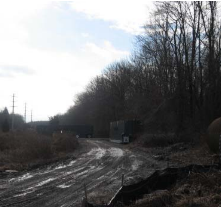
Manville Rd: Frac tanks are being used for dewatering in this area since the dewatering basin is no longer functional.
