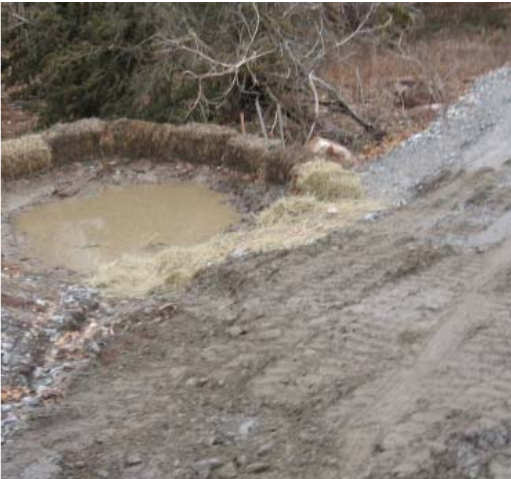
Brooksvale Ave: Existing controls remain functional, but additional controls are needed.
