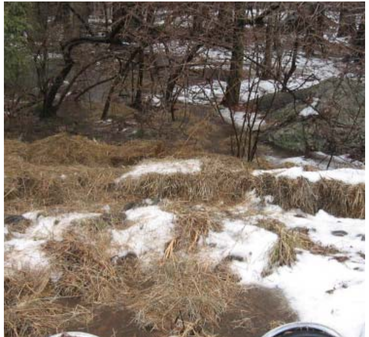
Gaylord Mtn Rd: Additional haybales were added to the sediment basin near structure #3992 to filter stormwater runoff.
