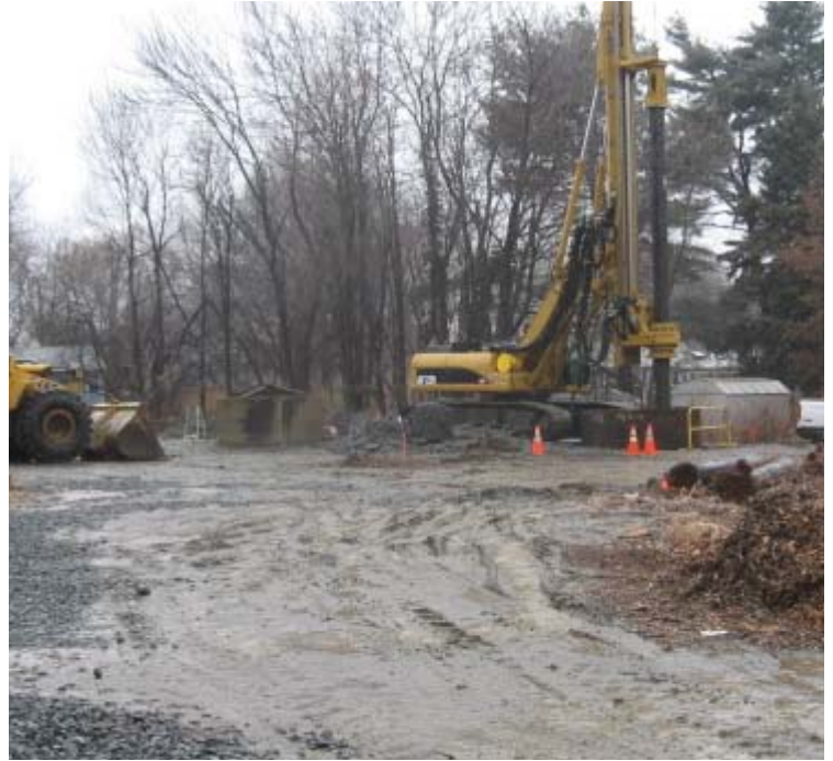
Russell Ave (Orange): Drilling continues at structure #24058. A pile of wood chips remains in the ROW here and new stone has been added to the tracking pad.
