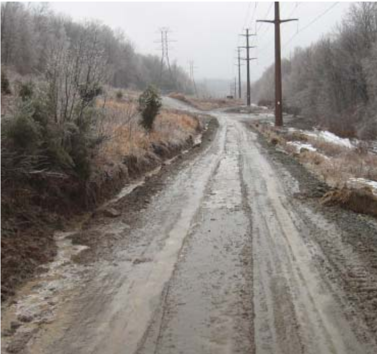
Gaylord Mtn Rd (Hamden): Additional waterbars were installed along the access road in an attempt to control stormwater runoff.
