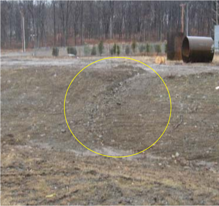
Plains Rd (Milford): Erosion is evident along the exposed slopes of the drainage swale located to the south of the East Devon substation.
