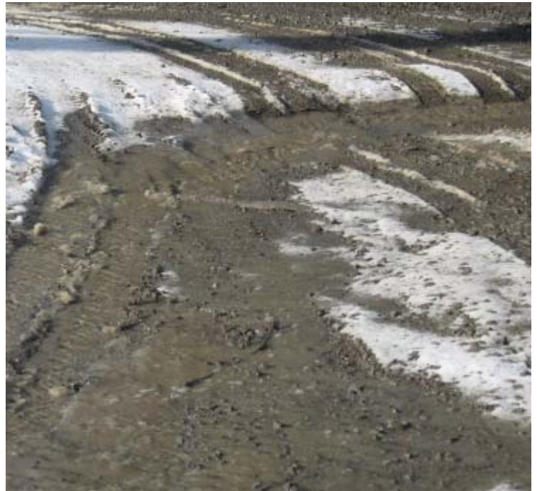
Pease Rd: View of stormwater being controlled by a waterbar.
