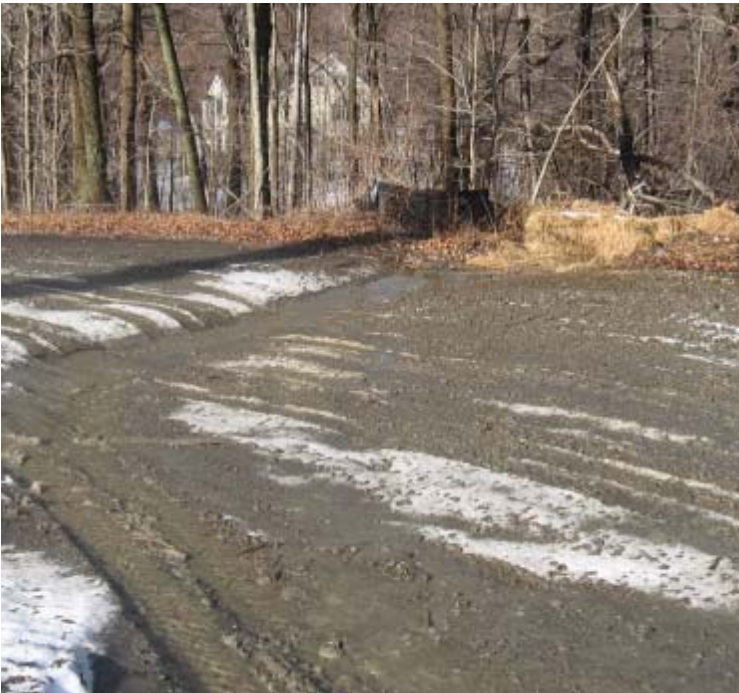
Pease Rd (Woodbridge): The waterbar was re-installed at the ROW access here.
