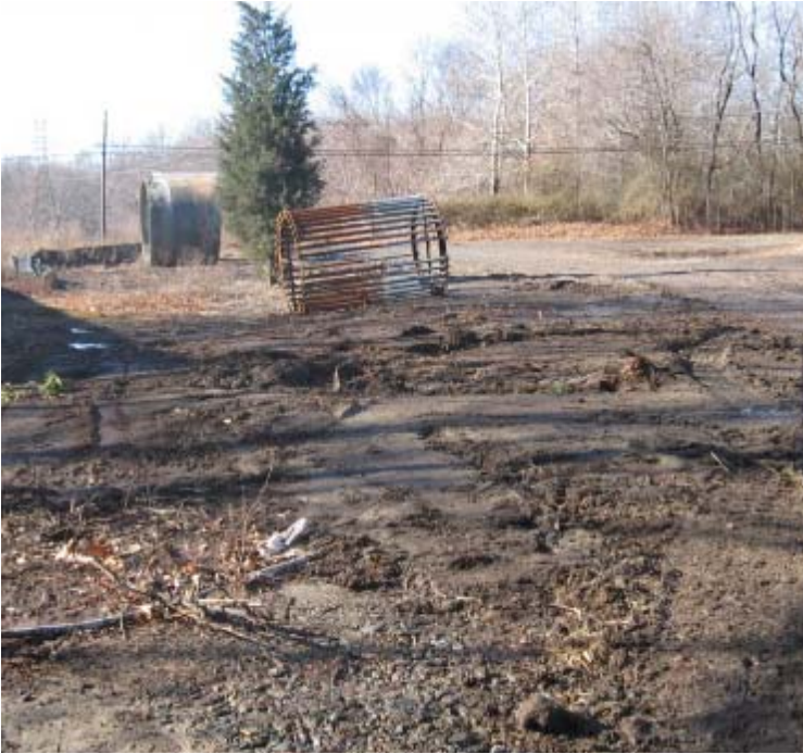
North St (Milford): The dewatering basin has been removed from the ROW near structure #3845.
