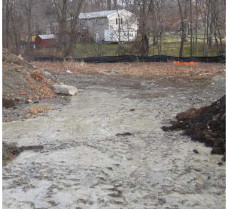
North St: View of the turbid water leaking from the dewatering basin near structure #3845.
