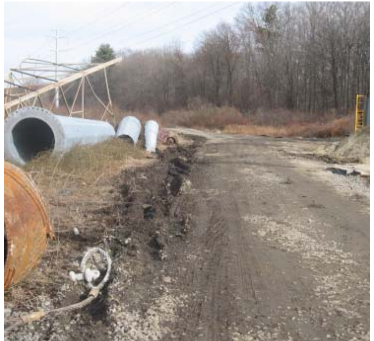
West River St (Milford): Tire ruts and a disassembled lattice tower remain in the wetland boundary near structure 24023.
