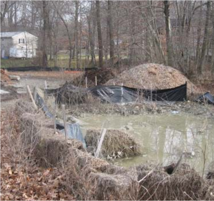
North St (Milford): The dewatering basin near structure #3845 was leaking during the inspection and turbid water was observed flowing towards the wetland (located in background of photo).
