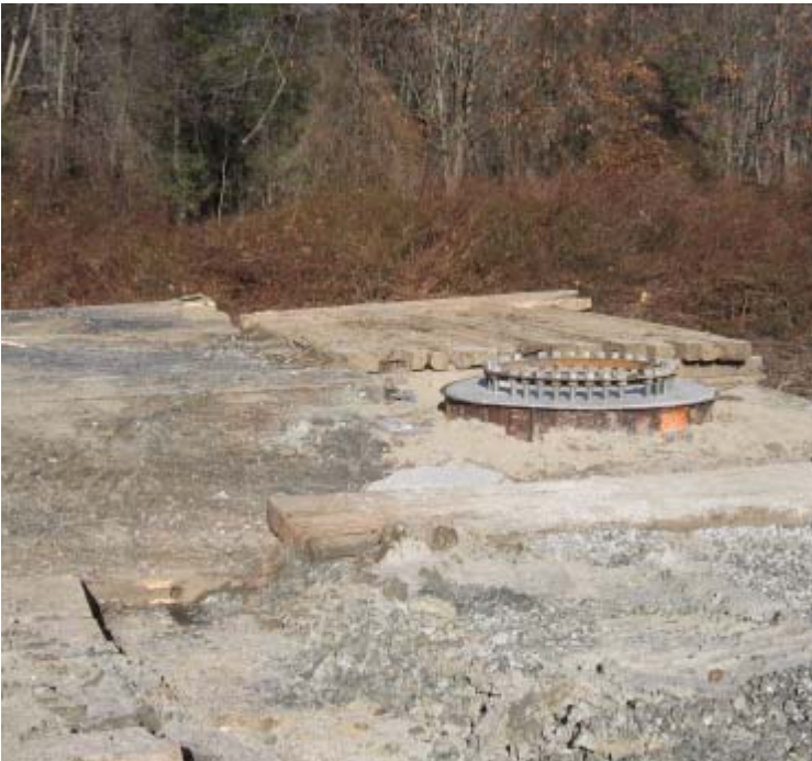
Eisenhower Park (Milford): Foundation installation is complete at structure #24026. Excess sediment remains on the crane pad and controls need to be installed around the perimeter of the pad.
