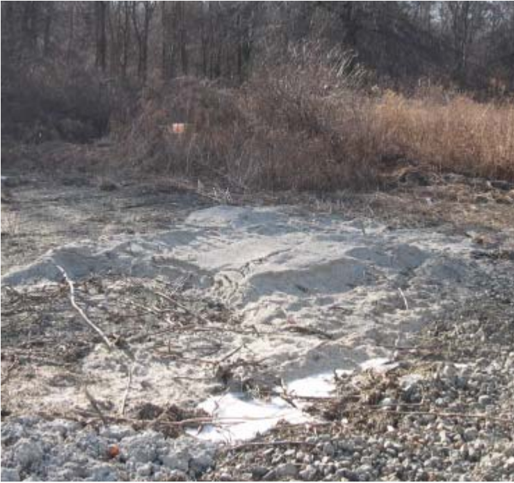
West River St (Milford): Sand used for foundation installation has been piled in a wetland area with no plastic liner above or beneath.
