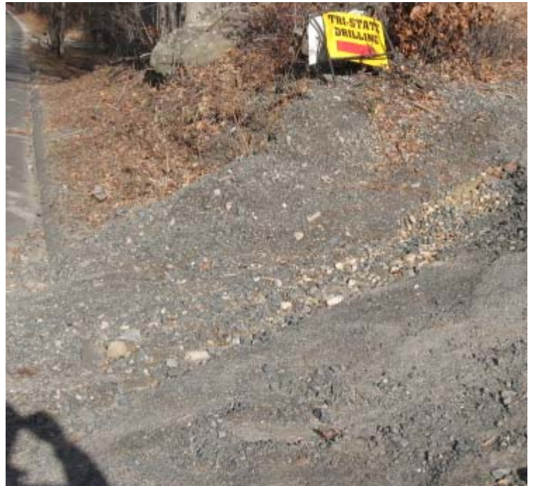
Pease Rd (Woodbridge): Stormwater runoff is eroding the access road here and sediment has migrated onto Pease Road.
