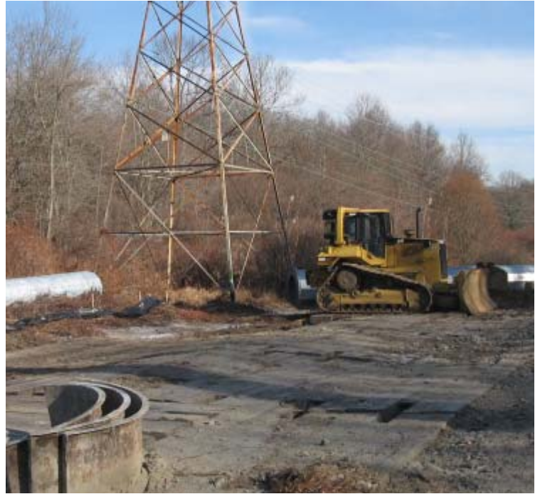
West River St: Equipment remains parked on a crane pad in a wetland area here.
