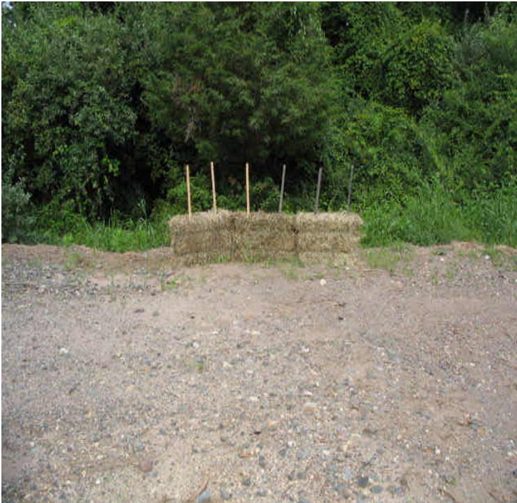
High Hill Rd: New haybales were installed to filter stormwater run-off from the access road.
