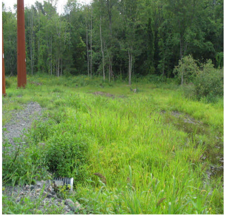
Carpenter Ln: Restoration work is complete within the wetlands. Areas were stabilizing with vegetative cover consisting mainly of native wetland species.
