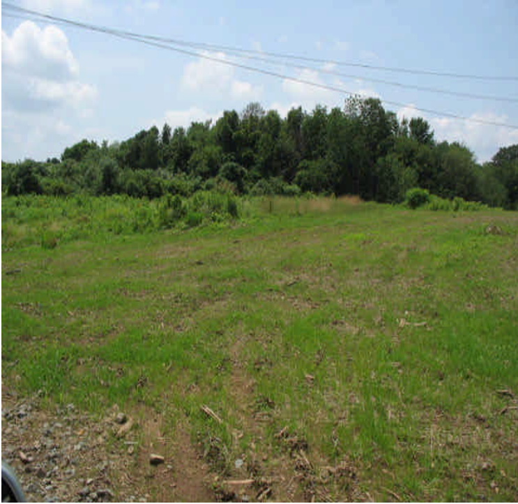
Carpenter Ln: Soil stockpiles were removed and the disturbed area remain graded and seeded. Some grass growth was noted.
