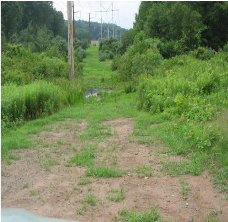
Durham Rd (South): Exposed access road sloping toward the wetlands. Needs minor controls to prevent run-off from entering the wetlands. The noted increase in vegetation will help filter run-off.
