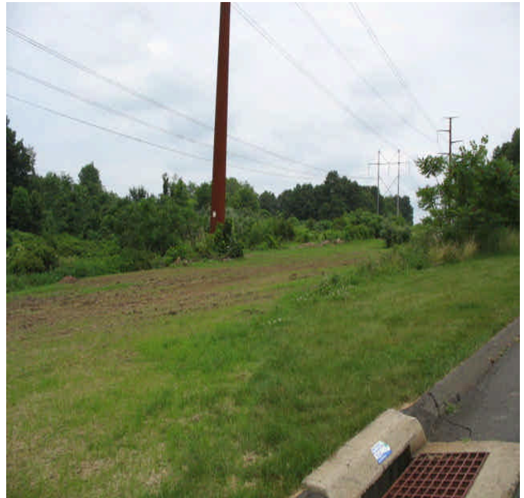
Stony Brook: Final grading/restoration complete. Topsoil, hay and seed remain in place.
