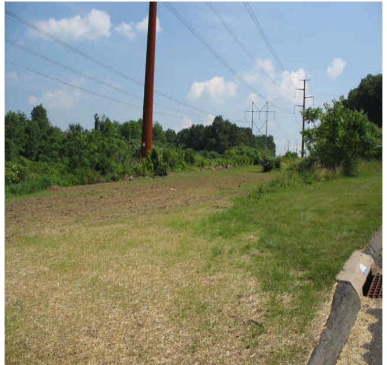
Stony Brook: Final grading/restoration complete. Topsoil, hay and seed have been spread.
