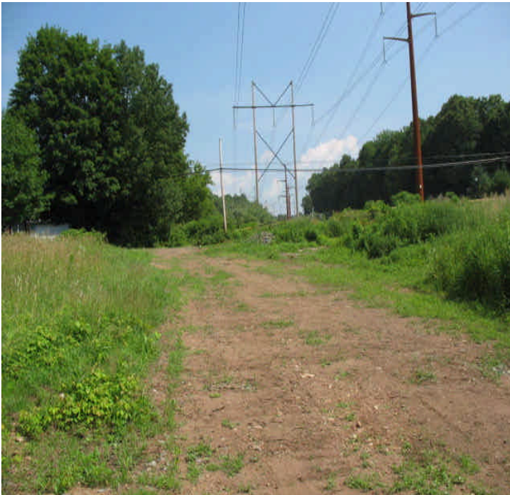
Durham Rd (South): Exposed access road sloping toward the wetlands. Needs minor controls to prevent run-off from entering the wetlands.
