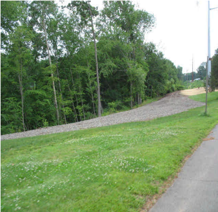
Harrison Rd: Pads and access roads removed, hayed, seeded, and landscaped as needed. New stone area installed in lawn by request of the landowner. (contractors state that the landowner has accepted the responsibility for topsoil and seeding).
