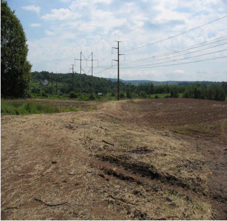
Tamarack Swamp: Access road pads narrowed and graded. Monitor for final cover.
