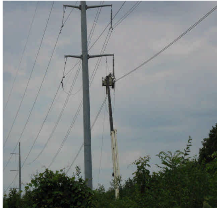
Old Farms Rd: Final section of line being installed at the 2A & 2B intersection.
