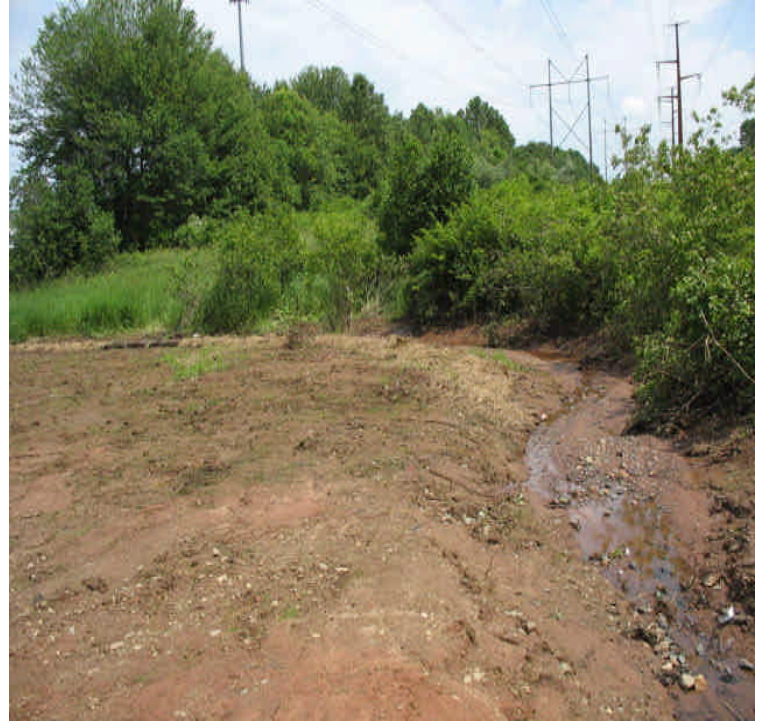
Powers Rd: Final restoration complete. Additional controls may be needed in exposed areas until the area is stable.
