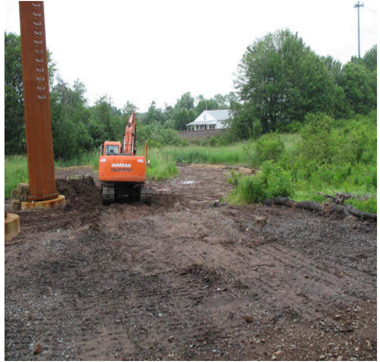
Powers Rd: Final restoration underway within the wetlands. Stone removal underway as needed. Crews are maintaining established vegetation when feasible.
