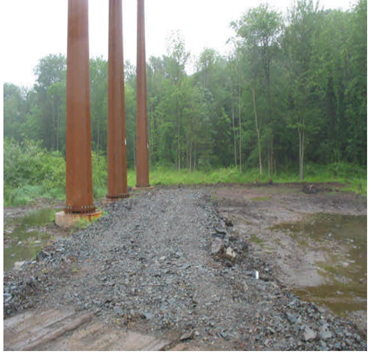
Carpenter Ln: Restoration work is complete within the wetlands. Minor seeding will be done when water subsides. Impacts were reduced from original permitted numbers and narrowed to a spur road.
