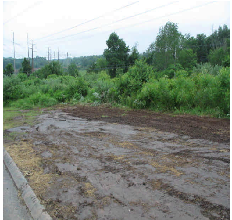
Stony Brook: Final grading/restoration complete. Topsoil, hay and seed have been spread. The area needs additional hay/seed.
