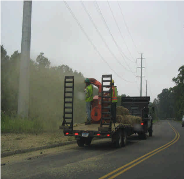
Old Farms Rd: Crews were spreading hay and seed on exposed areas along the roadway shoulder.
