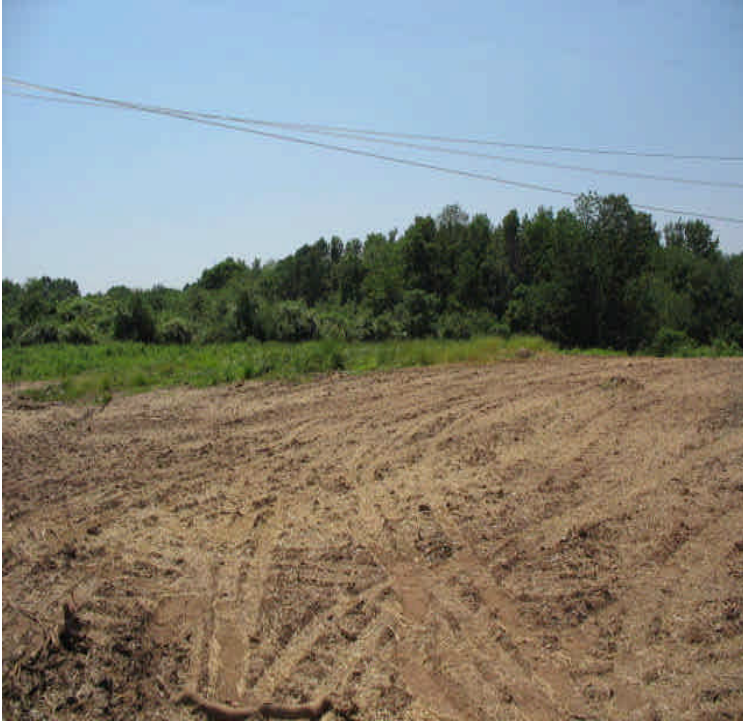
Carpenter Ln: Soil stockpiles were removed and the disturbed area has been graded and seeded
