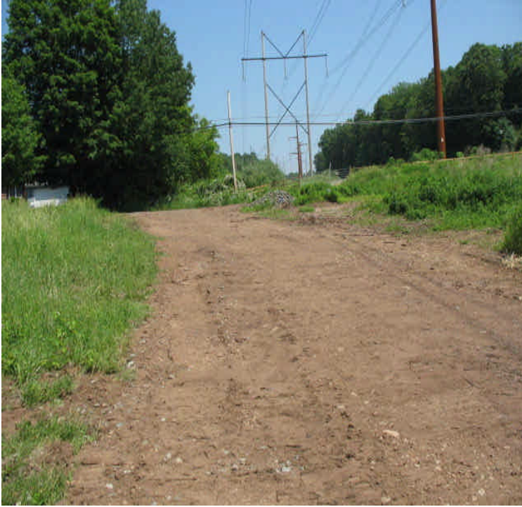
Durham Rd (south): Access road needs stabilization and controls need to be installed adjacent to the wetlands until stable.
