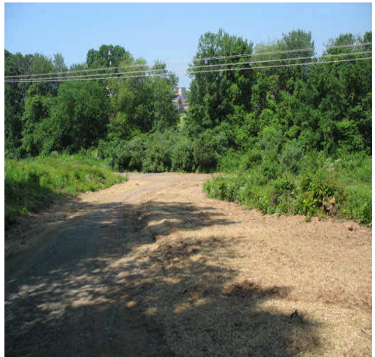
High Hill Rd: Final grading/restoration complete. Topsoil, hay and seed have been spread.
