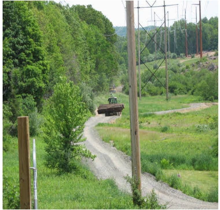
Liney Hall: Timber mat and bridge removal is underway. Restore exposed areas upon completion of work.
