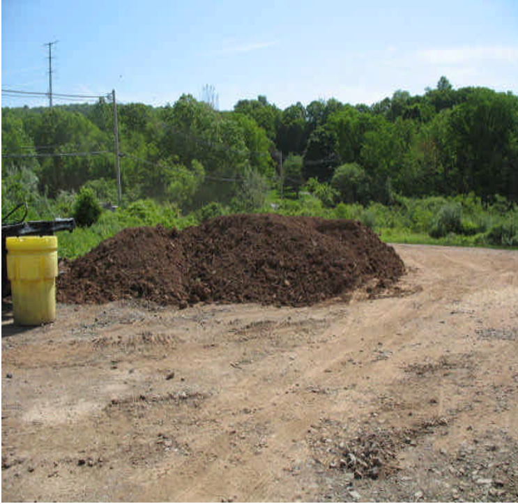
Carpenter Ln: Soil stockpile on site resulting from work within wetlands. Note that a spill control container has been left onsite proactively during restoration activities.
