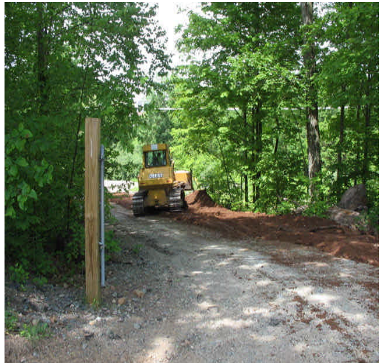
High Hill Rd: Final grading/restoration was underway. Crews were spreading topsoil at the site entrance.
