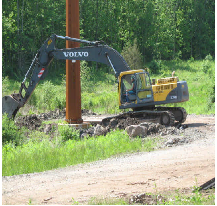
Carpenter Ln: Restoration work is underway within the wetlands. Monitor controls and equipment closely during work.
