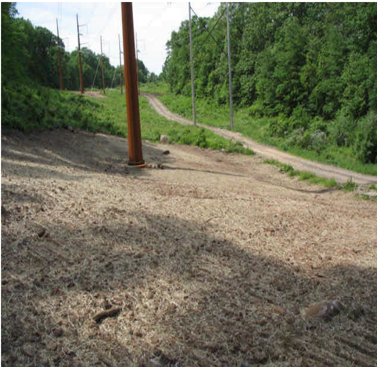
High Hill Rd: Final restoration continues. Crews were removing soils and applying hay and seed.
