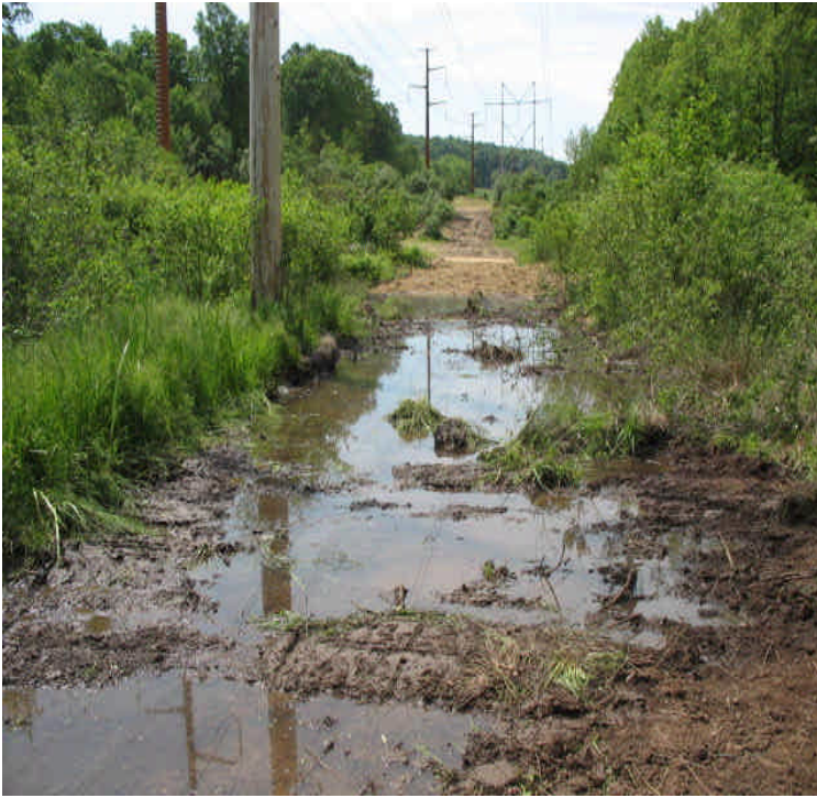
Durham (south): Timber mats and bridge have been removed from the flooded crossing. Monitor and stabilize exposed soils.
