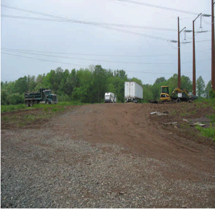
Carpenter Ln: Large area disturbed/exposed from line work. Crews continue to mobilize onsite for reclamation activities. Spill kits were also observed (proactively).
