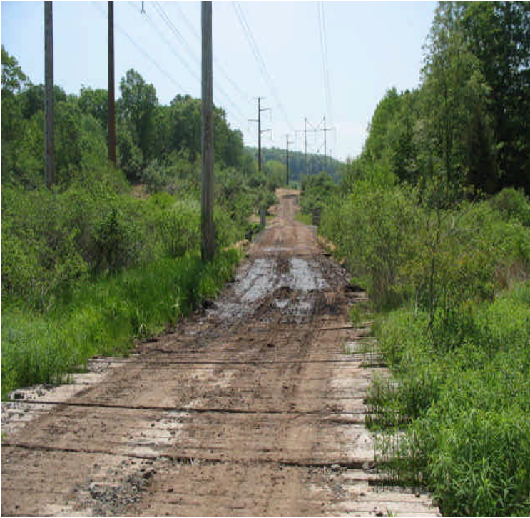
Durham (south): Timber mats and haybales added at flooded crossing. Additional mats and/or controls are needed when active. Sediment needs to be evaluated and removed by hand from the wetlands.
