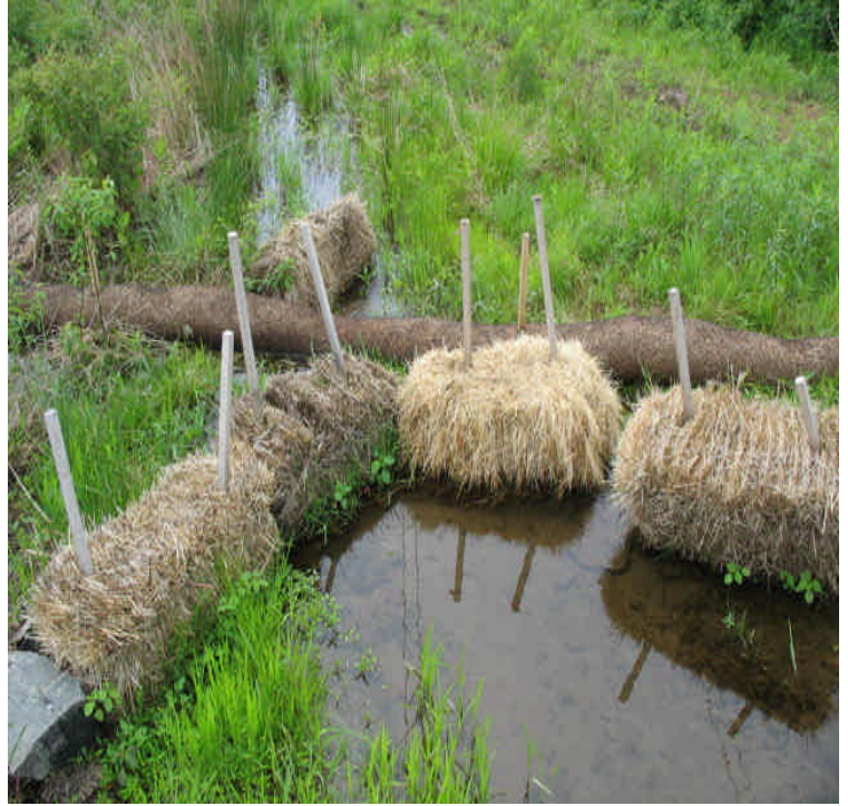
Carpenter Ln: New haybales and silt sock have been installed at the drainage outlet.
