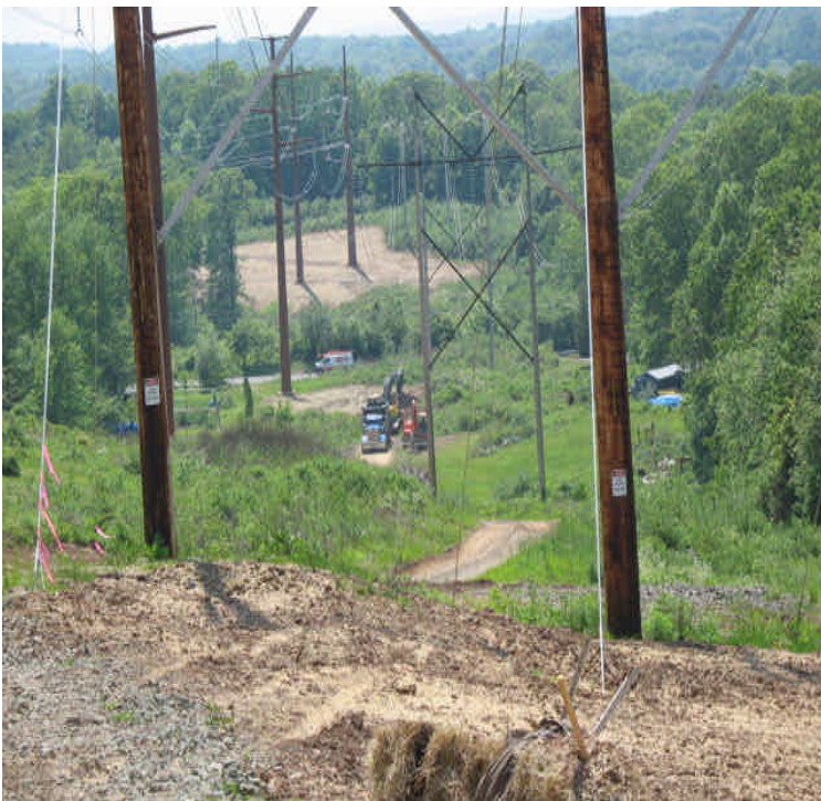
High Hill Rd: Final restoration underway. Removing stone/soils and applying hay and seed. Note the slope north of Durham Rd at final grade and seeded.
