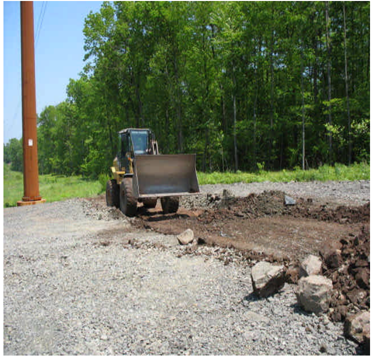
Stony Brook Rd: Final restoration of pads and access road narrowing were underway.
