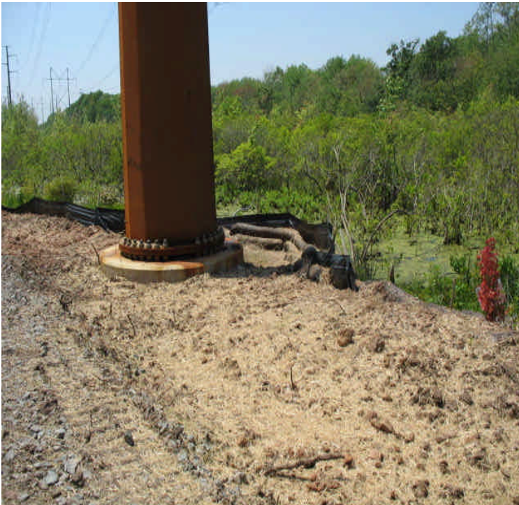
Tamarack Swamp Rd (southwestern side): Final grading is complete. Some sediment removed from the wetlands, hay and seed applied. Silt fence can be removed when vegetative cover has established.
