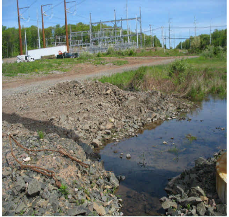
Carpenter Ln: The stone/sediment stockpile from pad work that was left in/adjacent to wetlands has been pushed further into wetlands to extend the pad.
