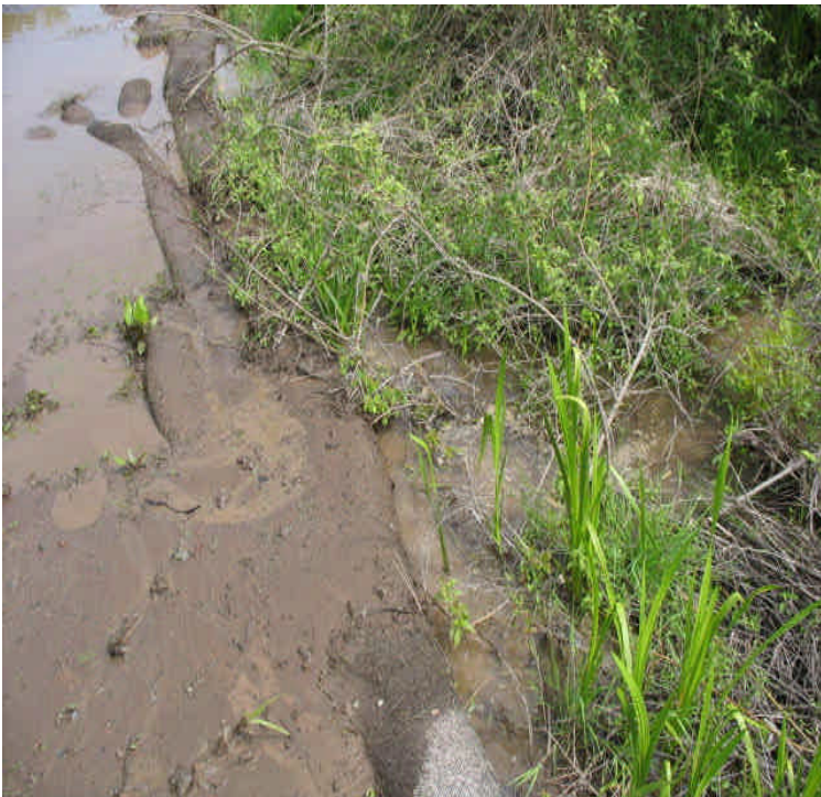
Durham Rd: Mud and turbid water noted spilling over the controls at the timber mat wetland crossing. Additional controls and possible sediment removal needed.
