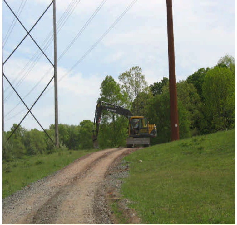
Liney Hall Ln: Final restoration of pads and access road narrowing were underway.
