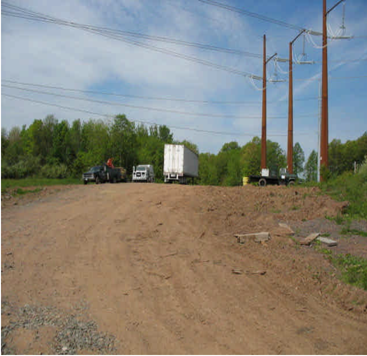
Carpenter Ln: Large area disturbed/exposed from line work. Crews continue to mobilize onsite for reclamation activities. Spill kits were also observed (proactively).
