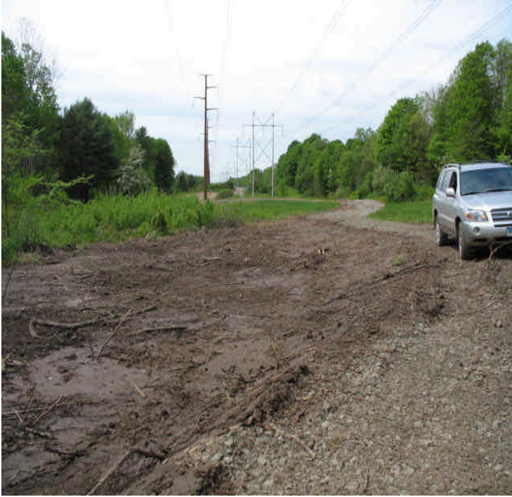
Liney Hall Ln: Timber mats removed from the wetlands. Minor amounts of stone remain in the wetlands and should be removed by hand.
