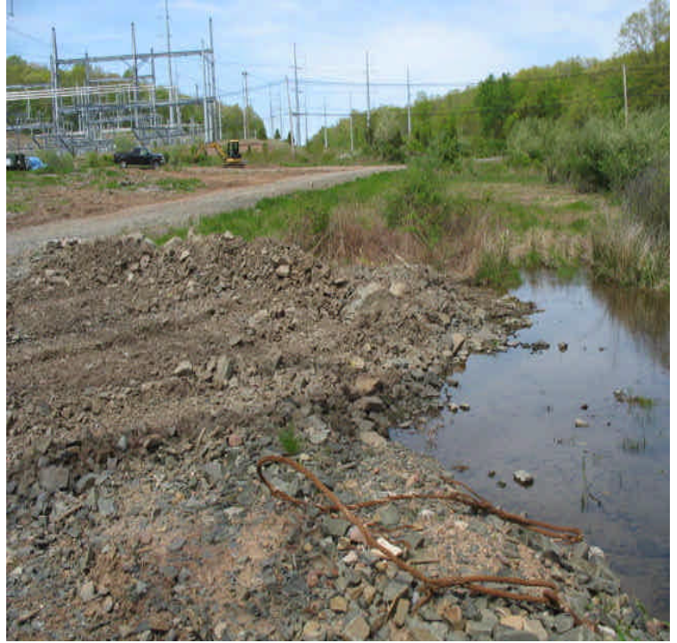
Carpenter Ln: The stone/sediment stockpile from pad work that was left in/adjacent to wetlands has been pushed further into wetlands to extend the pad.
