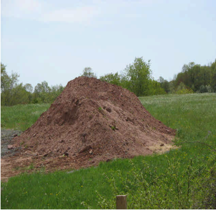
Tamarack Swamp: Stockpile located in the uplands. Stabilize or remove as soon as possible.
