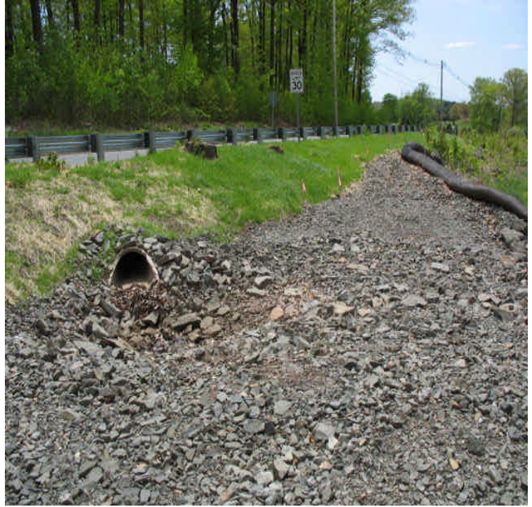
Harrison Rd: View of the recently installed stormwater solution for run-off from the roadway. Stormwater has been percolating through the stone during heavy rain. Continue to evaluate.
