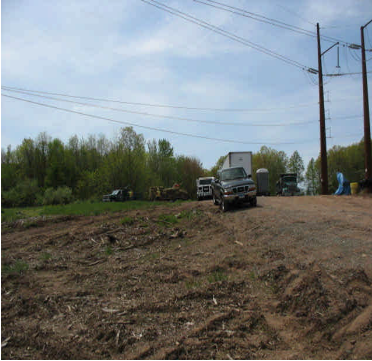
Carpenter Ln: Large area disturbed/exposed from line work. Crews were starting to bring equipment to the site for reclamation activities.
