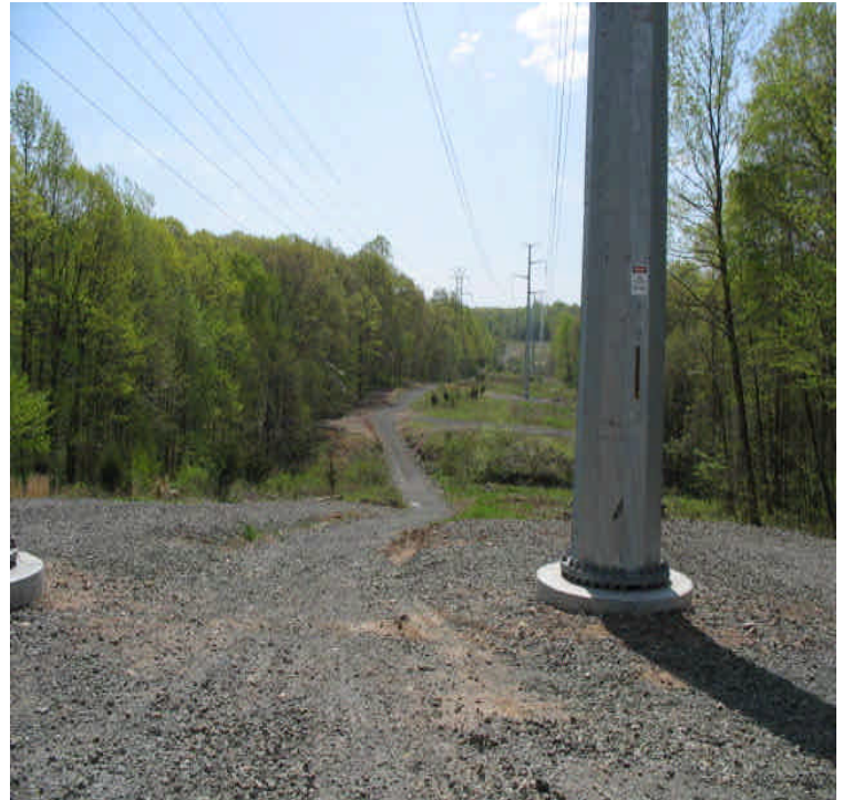
Tuttle Rd: Wetland crossings and water bars look good. Water is clear at the crossings and vegetative growth has returned.
