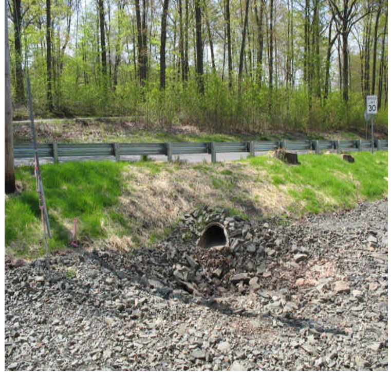
Harrison Rd: View of the recently installed stormwater solution for run-off from the roadway. Stormwater was percolating through the stone during heavy rain without causing erosion. Continue to evaluate
