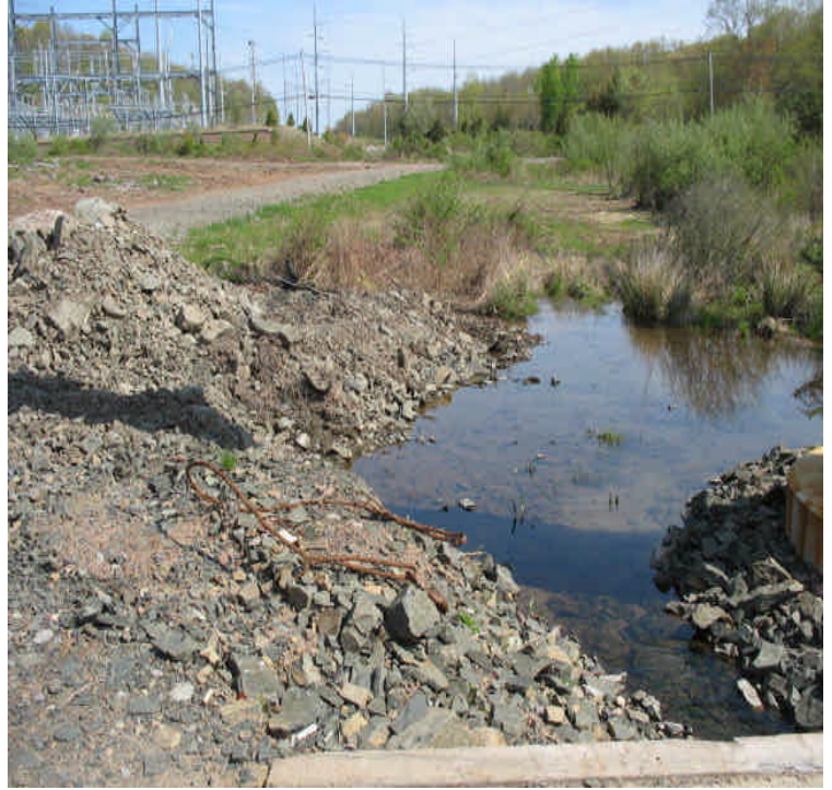
Carpenter Ln: Stone/sediment stockpile from pad work was located in/adjacent to wetlands. Relocate or remove the stockpile greater than 100 feet from wetlands. Also, controls at the outlet should be repaired prior to additional work.
