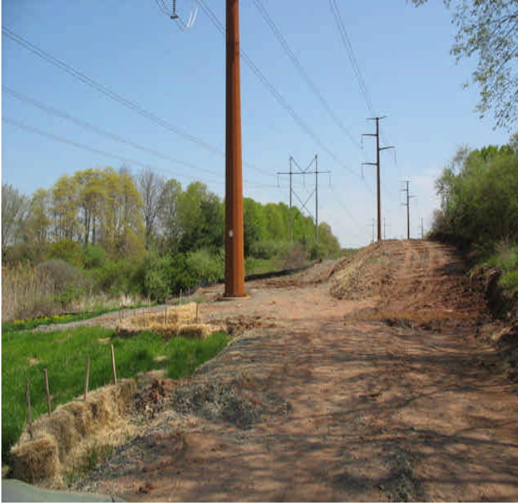
Powers Rd: Timber mat removal complete at the saturated crossing. Controls remain in place at the wetland. Hay/seed applied along the slope. Final reclamation is still proposed at the pad.
