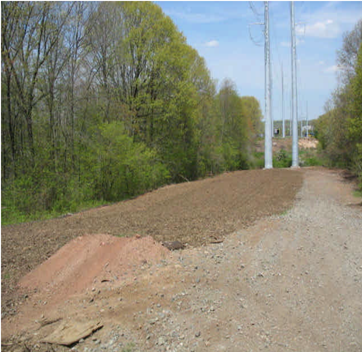
Docker Dr: Heavy mulch was applied over exposed soils for stabilization from stormwater/erosion and ATV traffic.
