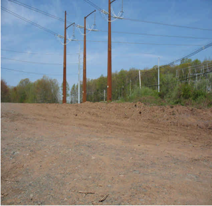
Carpenter Ln: Large area disturbed/exposed during line crew work remains upgradient from wetlands. Final grade and stabilize this area which has remained inactive for several weeks.
