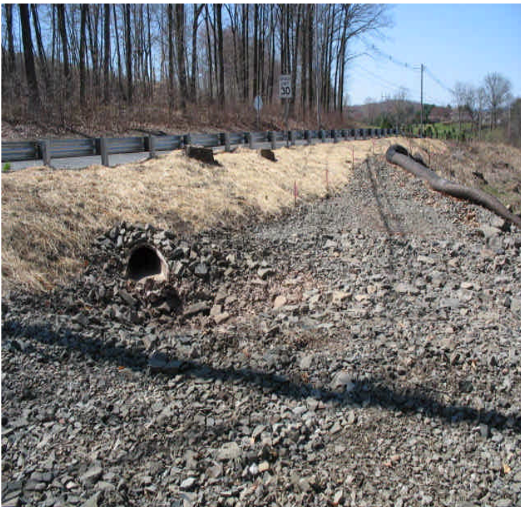
Harrison Rd: Crews installed a more permanent solution to filter and slow the stormwater from the roadway that outlets to the ROW. They were building a detention area/"surge pool" to allow water to flow over a flat grade prior to heading downslope.
