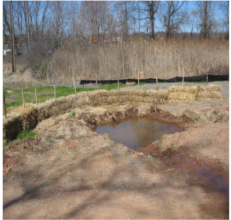
Powers Rd: Additional controls appear to be filtering all run-off from the bypass access road before it leaves the site.
