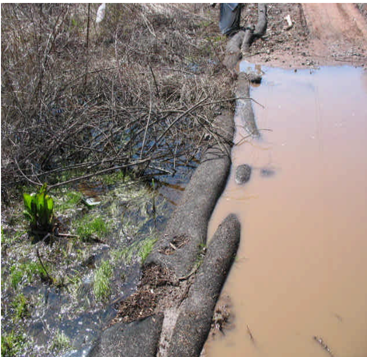
Durham Rd: Turbid water noted at the wetland crossing however sediment is filtering out before entering the wetlands. Continue to monitor carefully.
