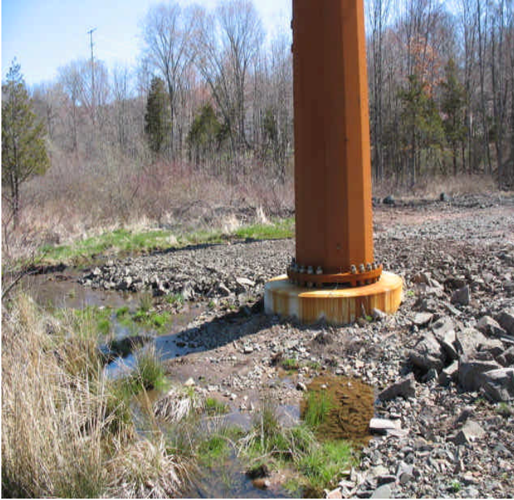
Carpenter Ln: New areas of stone installed were within the wetlands. Crews are reducing the overall wetland impacts by eliminating one of the proposed access roads to the structures but they are working on an access connection between the sets.
