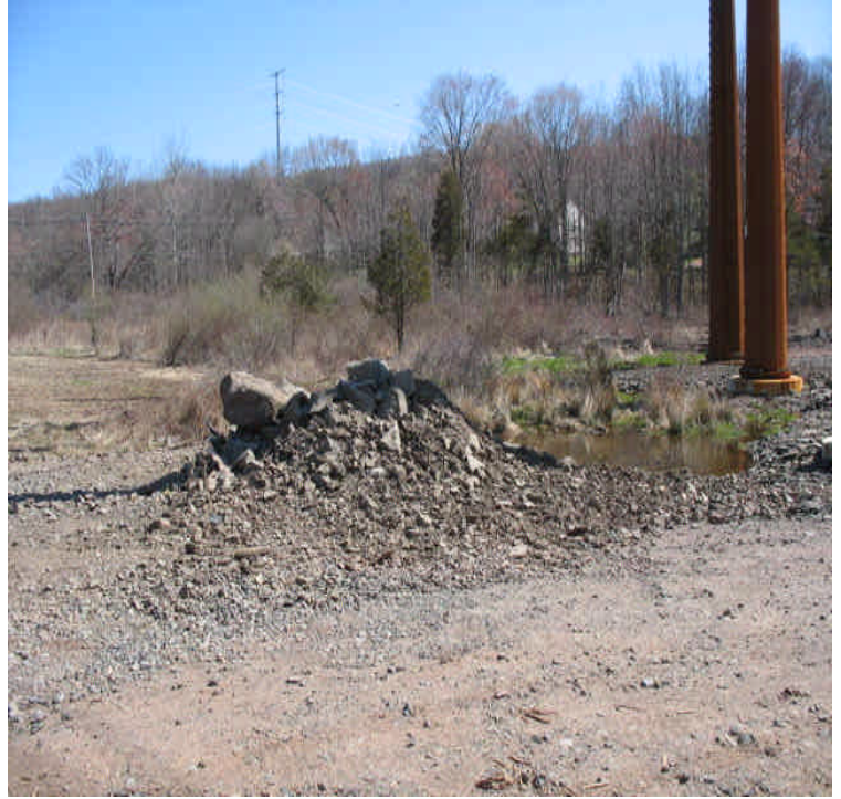
Carpenter Ln: Stone/sediment stockpile from the work was located upgradient from wetlands. Relocate or remove the stockpile greater than 100 feet from wetlands. Also, controls at the outlet did not appear to be repaired following the observation of turbidity in the water last week.
