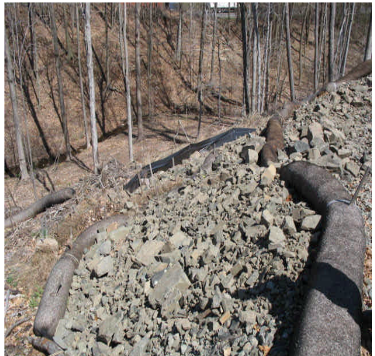
Harrison Rd: The top terrace of the slope below the newly installed detention area has been covered in riprap for stabilization. The pad here will remain, as requested by the golf club, for maintenance crew parking.
