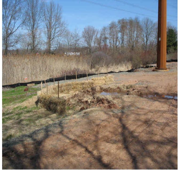
Powers Rd: Additional controls appear to be filtering all run-off from the bypass access road before it leaves the site.
