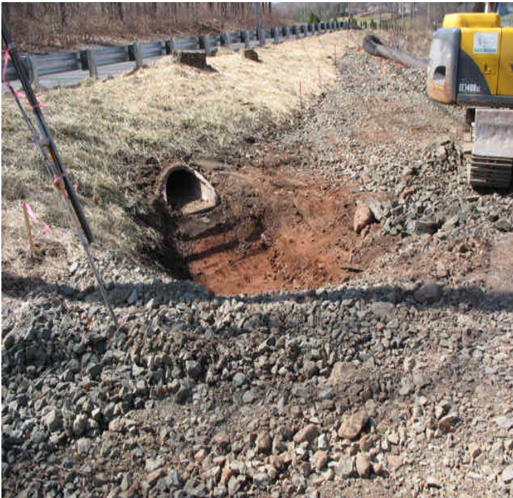
Harrison Rd: Crews were working on a more permanent solution to filter and slow the stormwater from the roadway that outlets to the ROW. They were building a detention area to allow water to flow over a flat grade prior to heading downslope.
