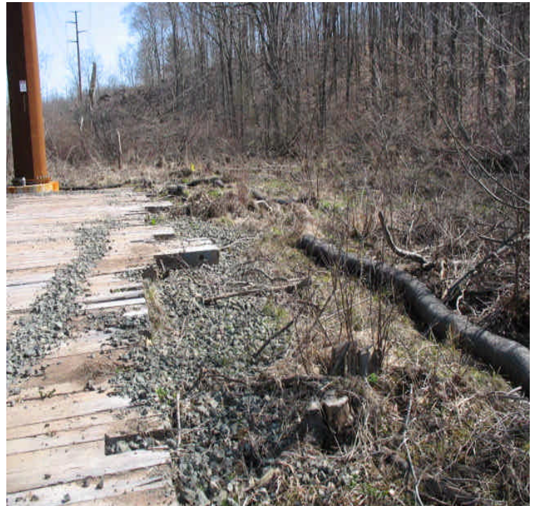
Liney Hall Ln: Stone resulting from snow plowing several weeks ago should be removed from wetlands. Final restoration is still needed.
