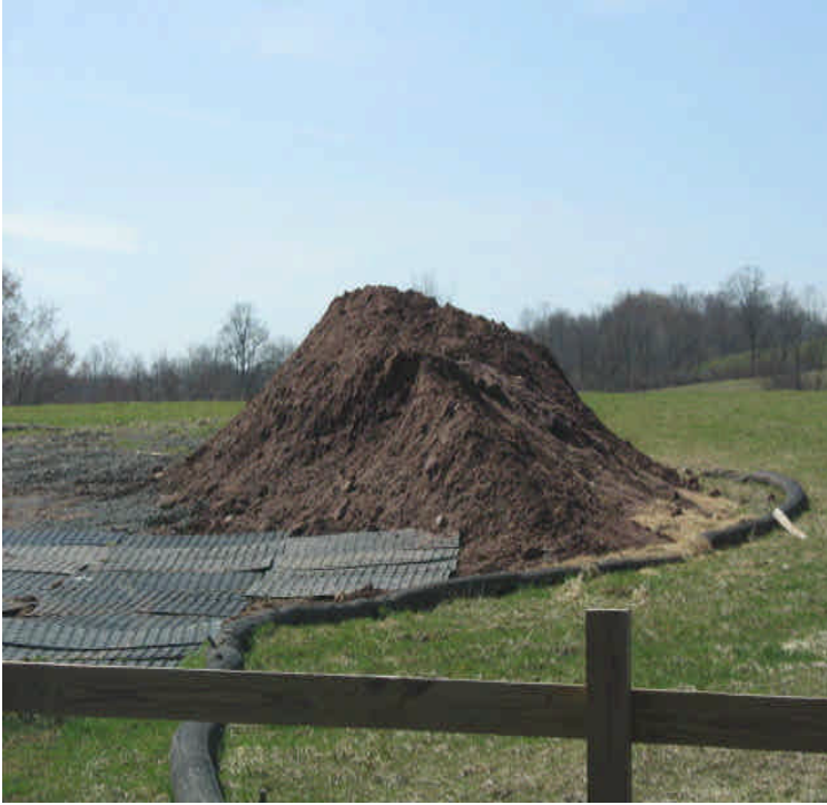
Tamarack Swamp: Soil stockpile should be removed or stabilized. Controls were present at the base but the soil is not fully contained.
