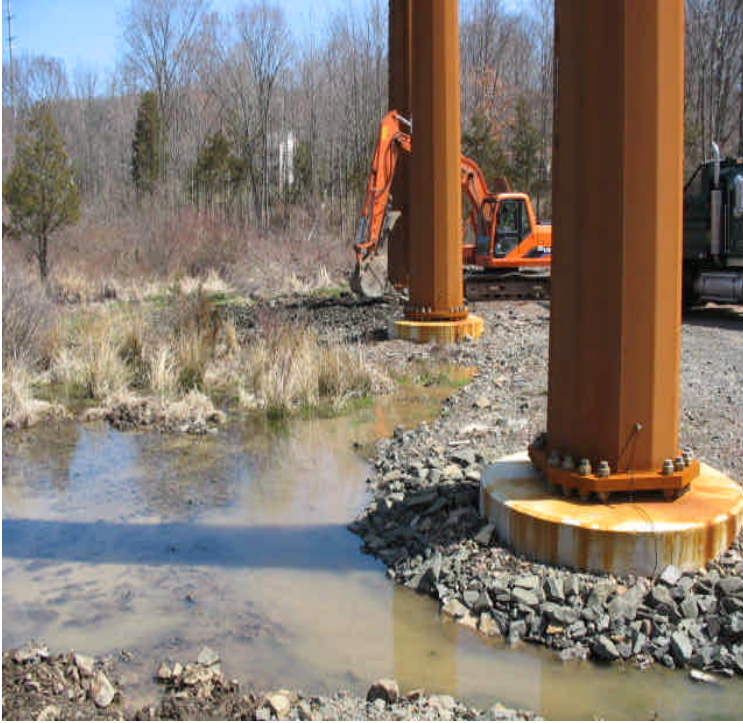
Carpenter Ln: Pad/road work was underway within the wetlands which was generating sediment that was entering the water and flowing off-site.
