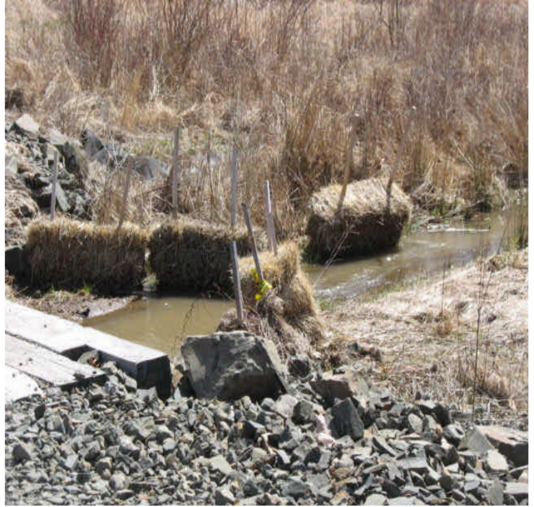
Carpenter Ln: The high flow at the outlet will not allow the haybale controls to stay in place. However, the turbid water resulting from the pad work needs to be filtered before it leaves the site. Install appropriate controls ASAP.
