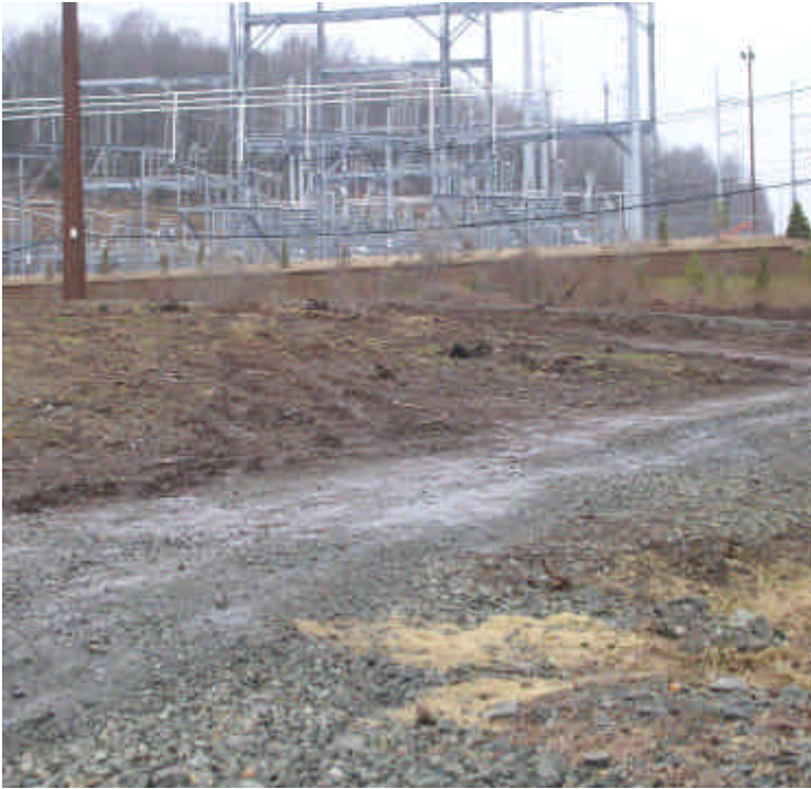
Carpenter Ln: A large, recently exposed area needs stabilization. (Beseck SS seen beyond the area, to the north of the roadway).
