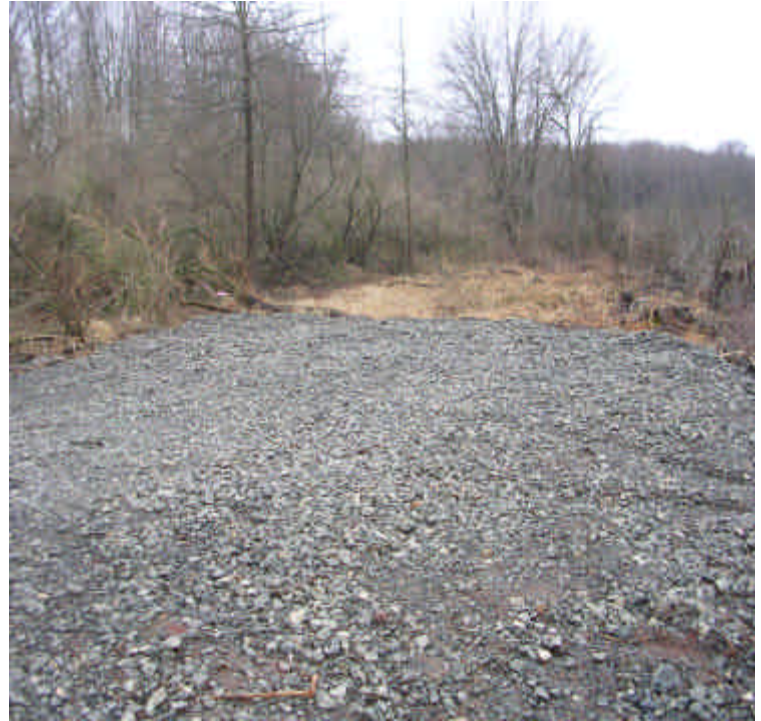
Tamarack Swamp Rd: The stone stockpile resulting from snowplowin has been removed and regraded.
