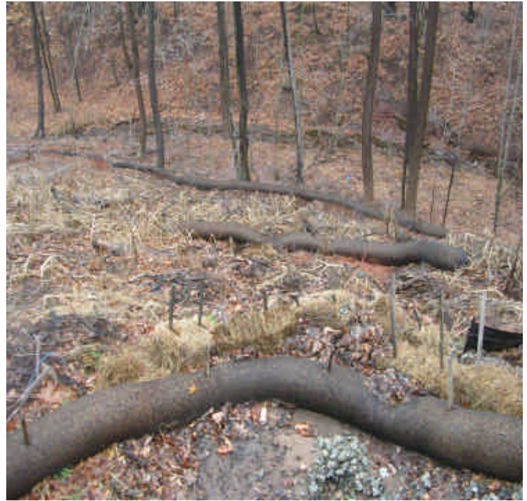
Harrison Rd: Hay was installed at the undermined areas within the controls. Sediment was pulled away from controls where needed. Work on a long term solution has been approved and will be implemented soon.
