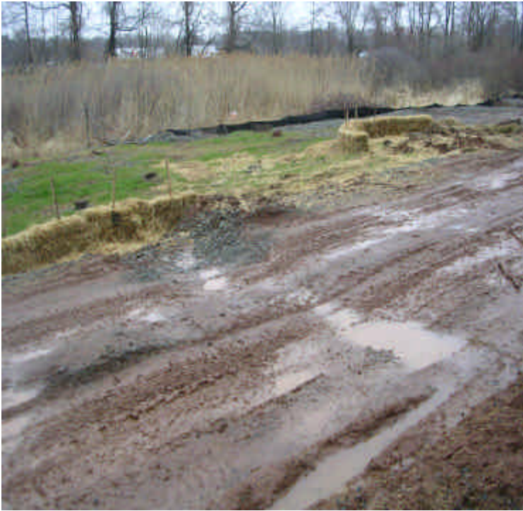
Powers Rd: Timber mat bypass remains stable. Additional controls were installed and run-off is being filtered.
