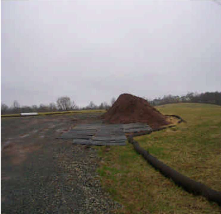
Tamarack Swamp: Stockpile should be removed or stabilized. Controls were present at the base but the soil is not fully contained.
