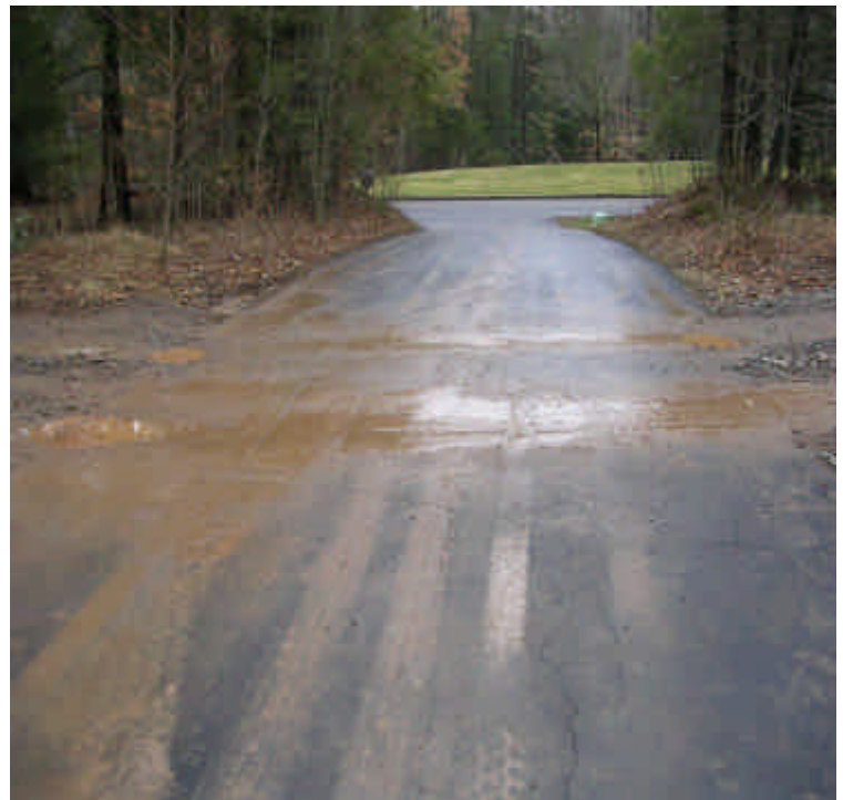
Old Farms Rd: Private driveway being used by equipment to access a section of ROW near Cook Hill Jct. Driveway should be swept and a tracking pad installed on either side. Monitor for any damage to the driveway
