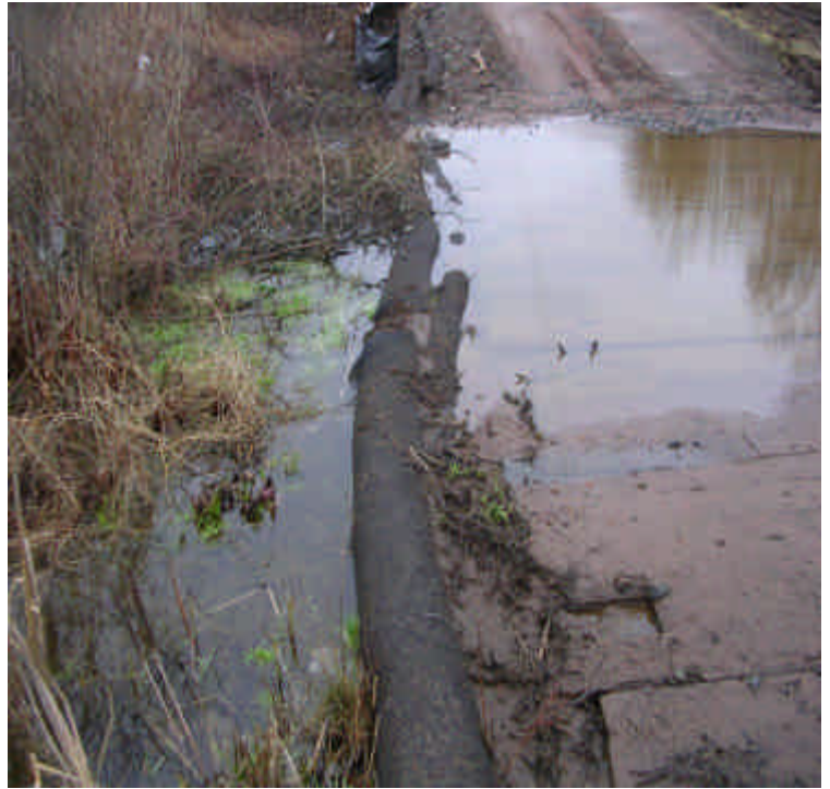
Durham Rd: Timber mats remain flooded at the wetland crossing, just before the bridge. Controls are still filtering the flow.
