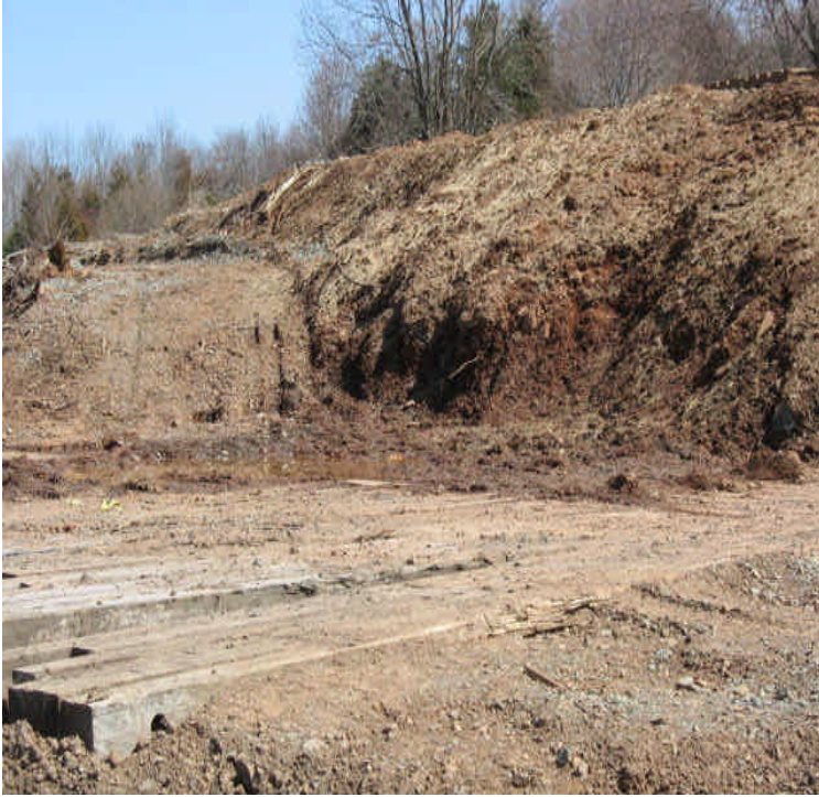
Powers Rd: Timber mat bypass is stable. Additional controls were installed downgradient.
