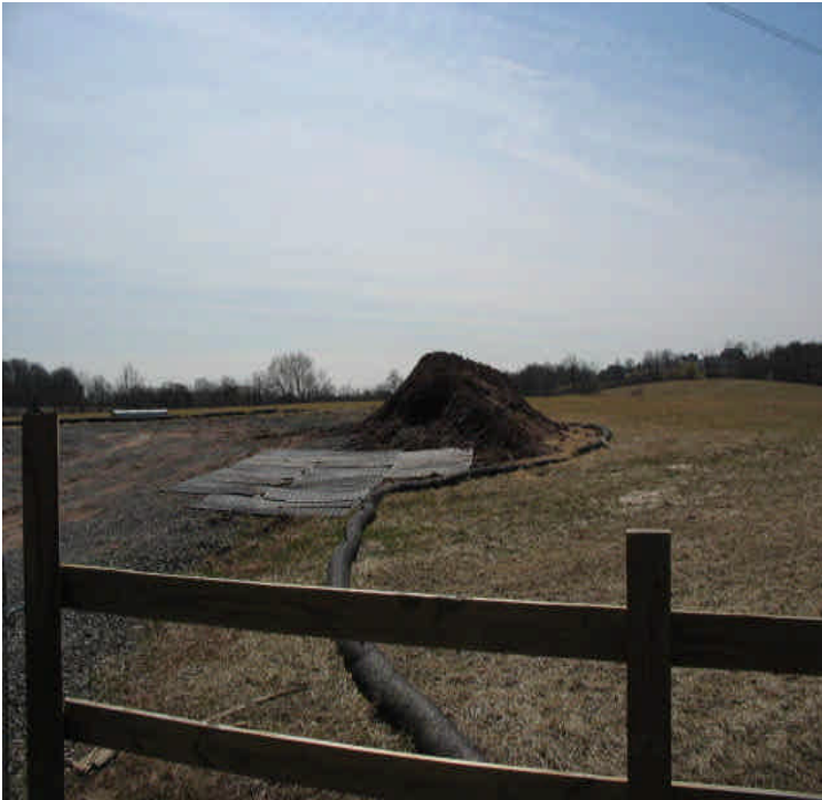
Tamarack Swamp Rd: Stockpile should be removed or stabilized. Controls were present at the base but the soil is not fully contained.
