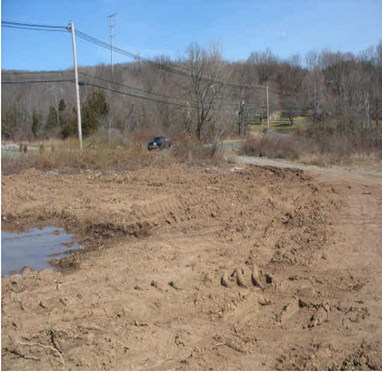
Carpenter Ln: A large, recently exposed area needs stabilization
