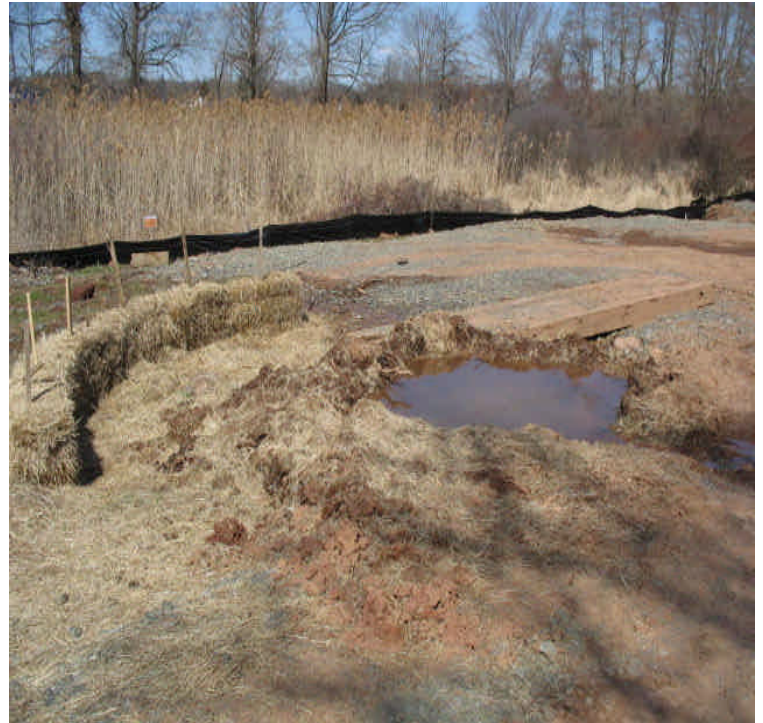
Powers Rd: Haybales and silt fence installed to filter run-off from the saturated, timber mat bypass-crossing.
