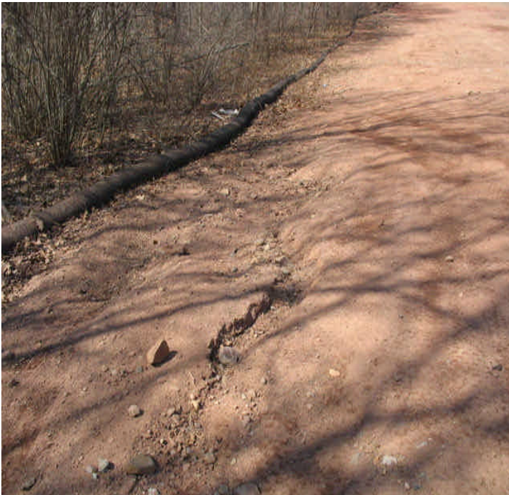
Docker Dr: Eroded rills/gullies had worsened along the slope due to heavy rain. Mulch/seed have washed away. Contractors are scheduled to return here with heavy mulch in an attempt to stabilize the area.
