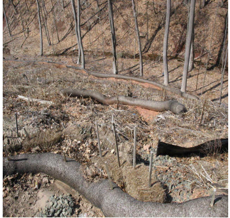
Harrison Rd: Stormwater has eroded soils and undermined controls where the gully had been noted on the slope for several months. Sediment has been pulled back from the controls but a long term solution needs to be evaluated.
