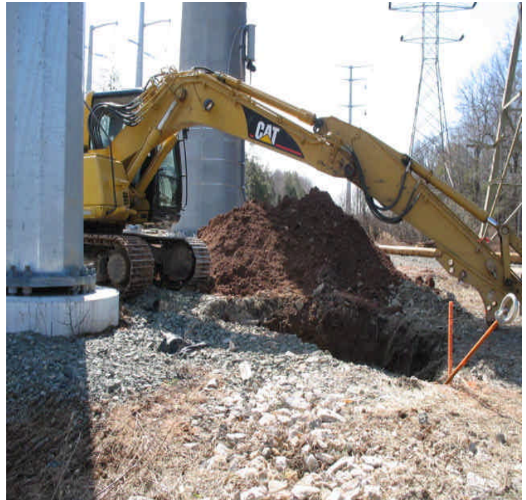
Old Farms Rd: Small stockpile and excavation/trench work noted at Cook Hill Jct. Fill and stabilize as needed upon the completion of work.
