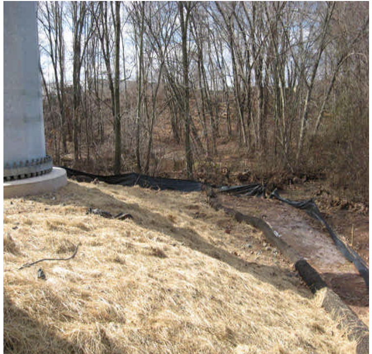
Docker Dr: Additional controls have been installed directly upgradient from wetlands.
