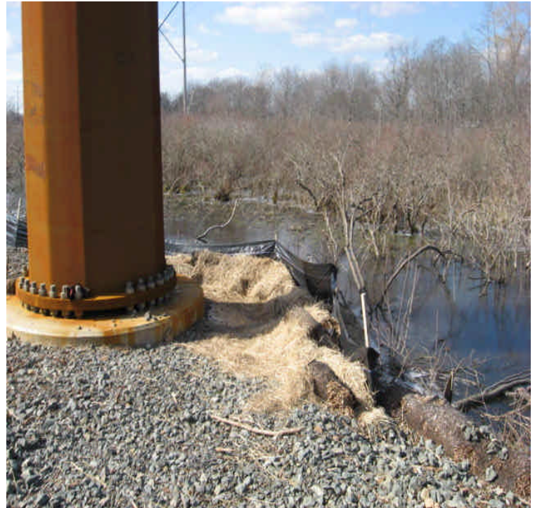
Tamarack Swamp Rd: Hay was added at foundation within the wetland.
