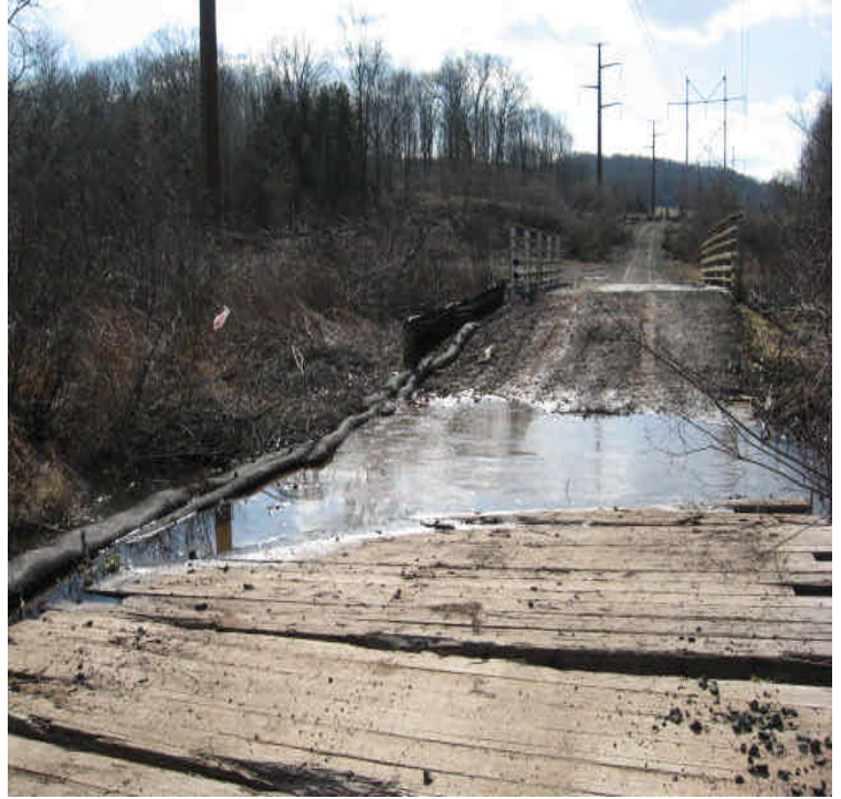
Durham Rd: Clear run-off noted across the access road and in the wetlands at the bridge over the Muddy River. Additional controls may be needed, especially when area is active.
