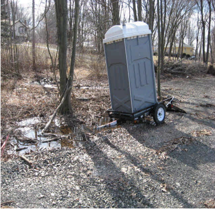
Powers Rd: Sanitary facility was located in standing water, upgradient from a wetland and not tied/secured into the trailer. This should be relocated, over 100 feet from wetlands.
