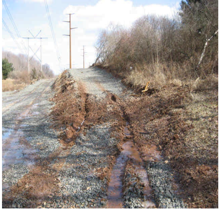
Powers Rd: Rutted tracks were noted at an access road by-pass. Turbid water from the tracks is eventually flowing into the wetlands.
