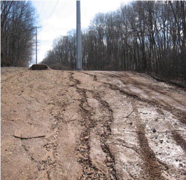
Docker Dr: Eroded channels/gullies from heavy rains and ruts from ATV traffic were noted along a steep slope. Contractors will return soon and attempt to stabilize with a bark mulch but there are large amounts of traffic here.
