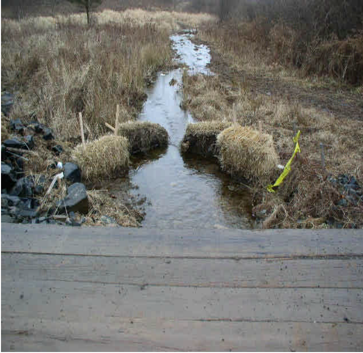
Carpenter Lane: Haybales have been knocked over at the wetland Outlet and should be righted and restaked. ATVs continue to damage controls and leave tracks in the wetlands.
