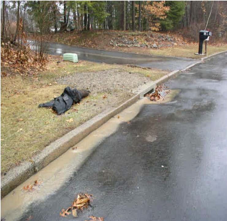
Old Farms Rd: Turbid run-off from access driveway and driveway crossings was entering CBs that did not have controls in place.
