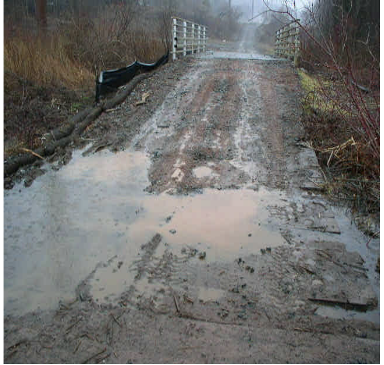
Durham Rd: Some run-off was noted but it is being filtered by control. Additional controls may be needed as water levels have the potential to overflow/overwhelm them here.
