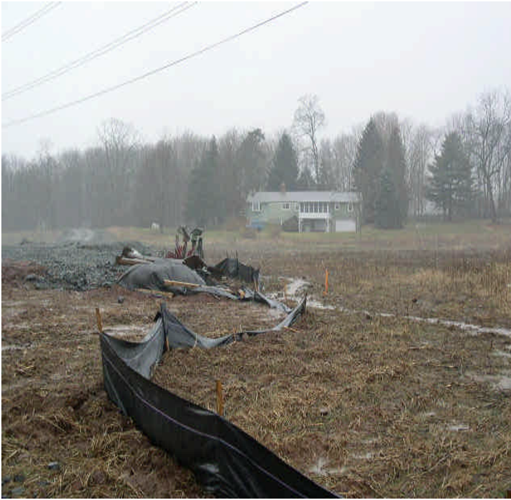
Tamarack Swamp Rd (east): Small section of deteriorated silt fence needs repair.
