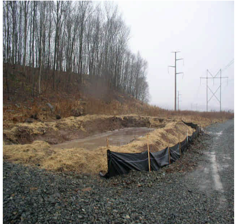
Stony Brook: Slurry dewatering pit appears contained. Once drilling is complete, this area should be graded and stabilized.
