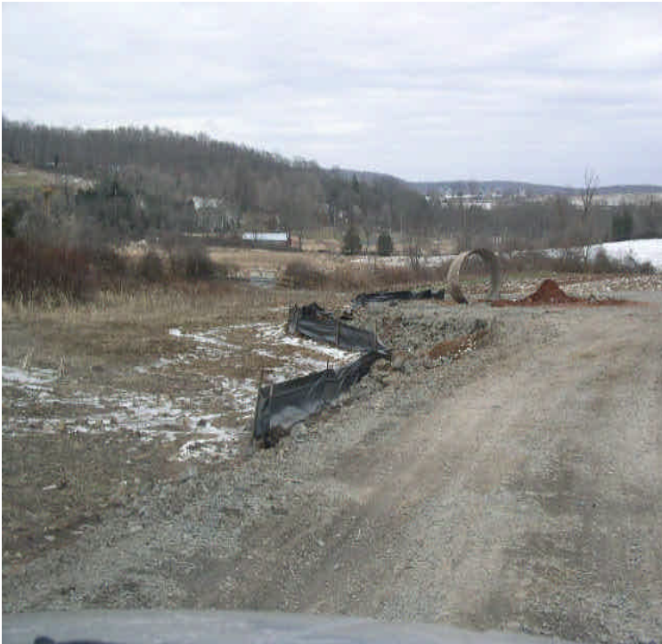
Tamarack Swamp: Controls noted along the pad and access road at wetland crossings. Wetland crossings will need to be removed and restored when access needs are complete.
