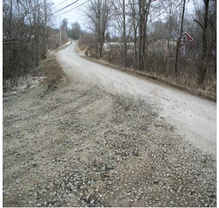
Tamarack Swamp Rd: New access road installation is complete. Wetland crossings were noted via culverts with controls. Sediment tracking was noted on the roadway and needs regular attention.
