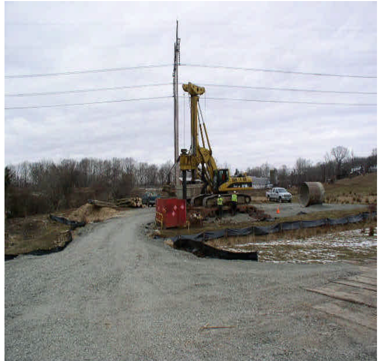
Tamarack Swamp: Foundation drilling underway. Small stockpiles associated with drilling were noted. Controls are in place.
