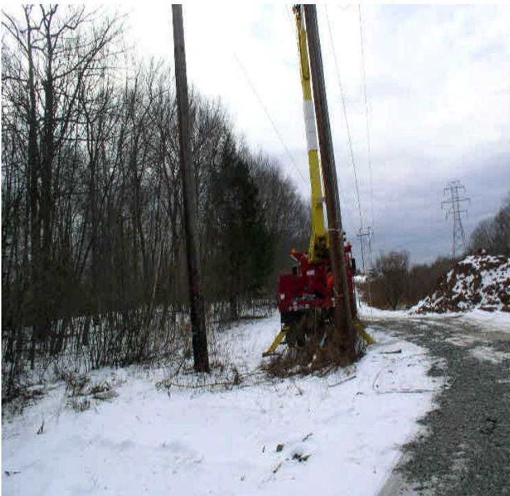
Old Farms Rd: Line work was underway at several sections in the ROW.
