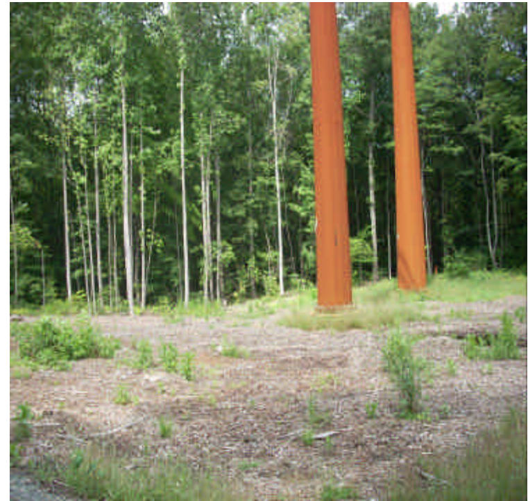
Another view of the pad/angle structure where vegetative cover is still sparse. The area remains stable with thick wood chips but vegetation will not be able to establish fully. The contractor plans to remove the chips and seed the area when feasible.
