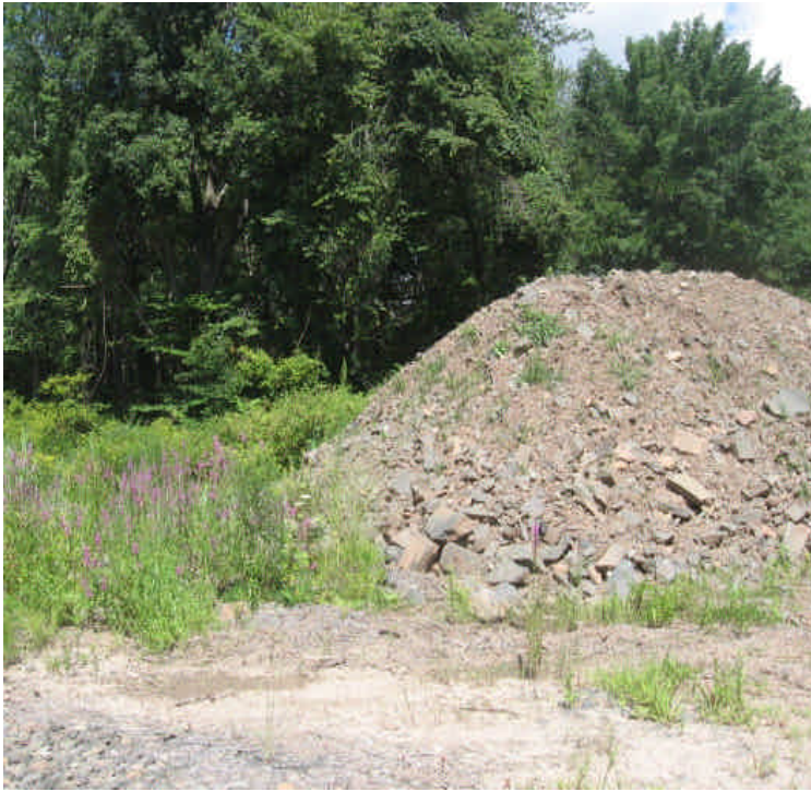
View of the stone/soil stockpile remaining in the contractor yard. Controls are in place but the pile is located just upgradient from wetlands and should be relocated.
