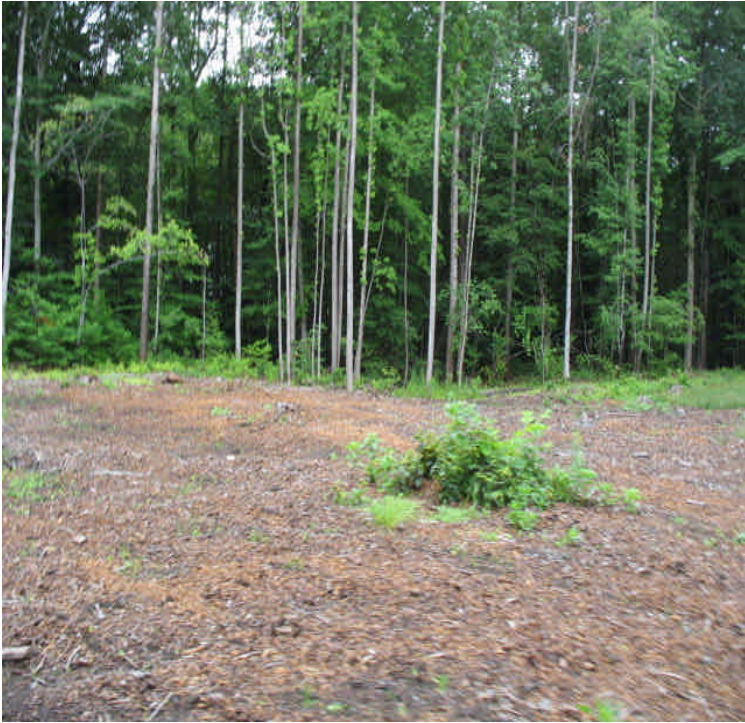
The pad at the turn towards Little Lane off the Receiving Yard has thick mulch/chips that are inhibiting vegetative growth.
