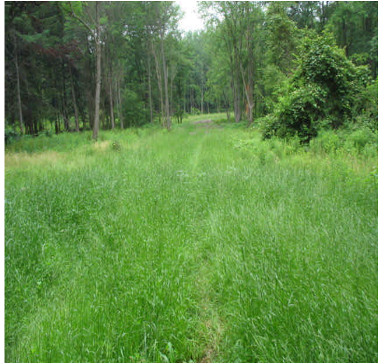
Grass is well established on the access road to Structure #24530. Minimal impacts were noted from culvert installation. Area is stable.
