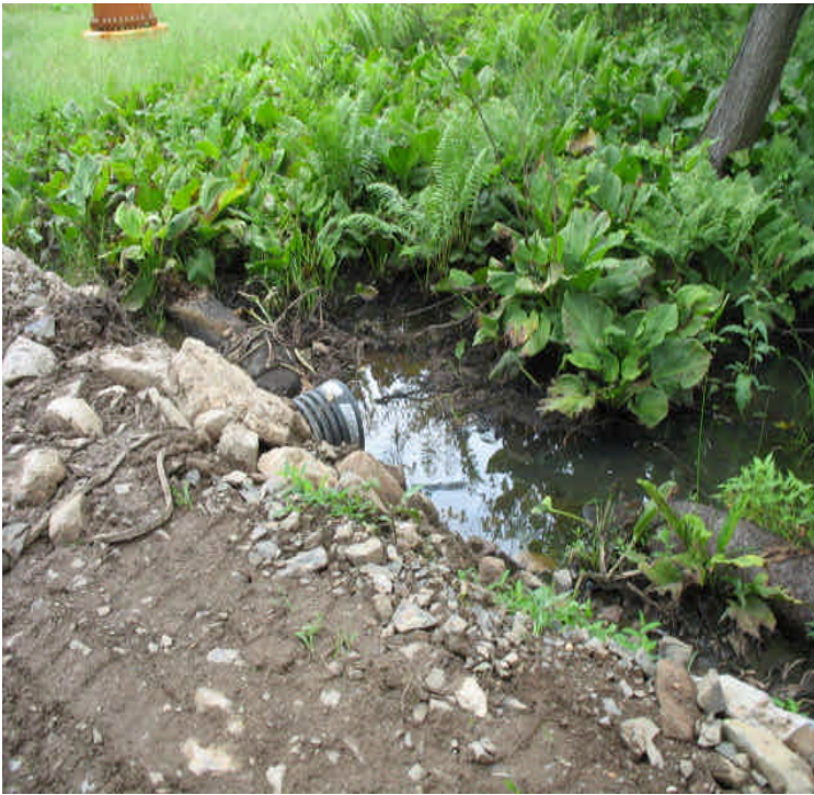
Culvert installed at the bisected channel crossing to Structure #24530. Continue to monitor to ensure hydrology is intact.
