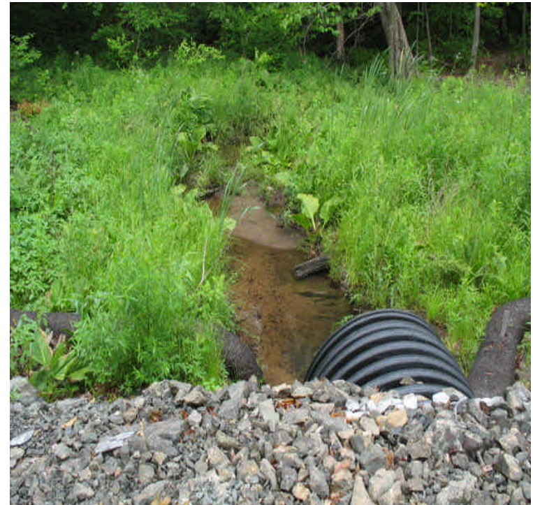
Clear water with tadpoles noted at the second culverted crossing past the receiving yard.
